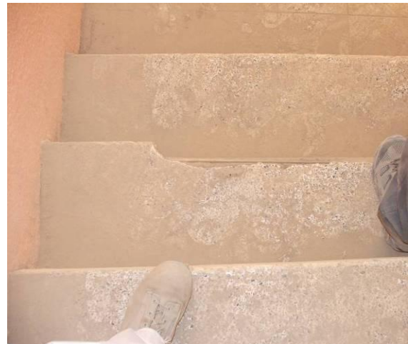
Site Photo 40. Broken stairs (Al Mualameen)
