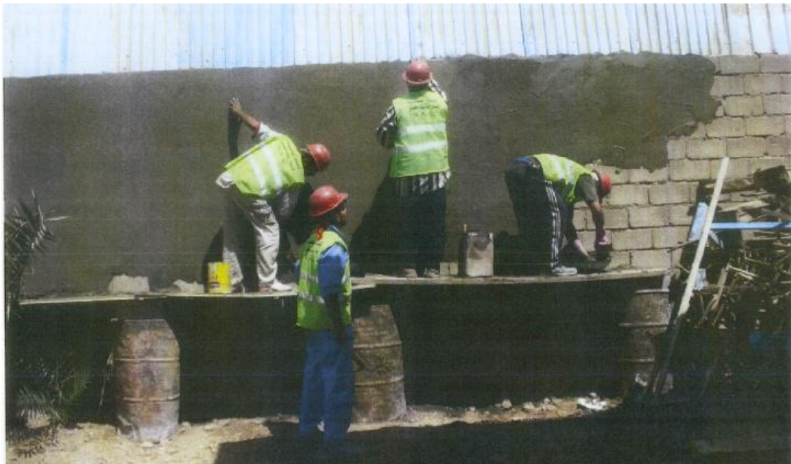
Site Photo 5. Plastering the wall at Al Mualameen (Photo courtesy of MNC-I)
