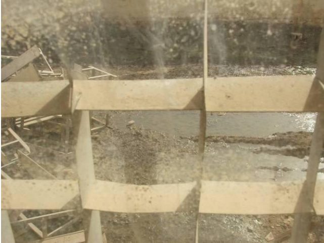
Site Photo 41. Exterior debris (Al Faoo)
