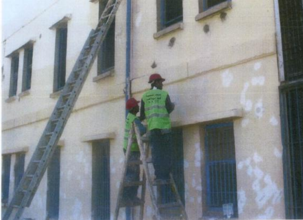
Site Photo 8. Plastering and painting the Al Faoo school exterior (Photo courtesy of MNC-I)
