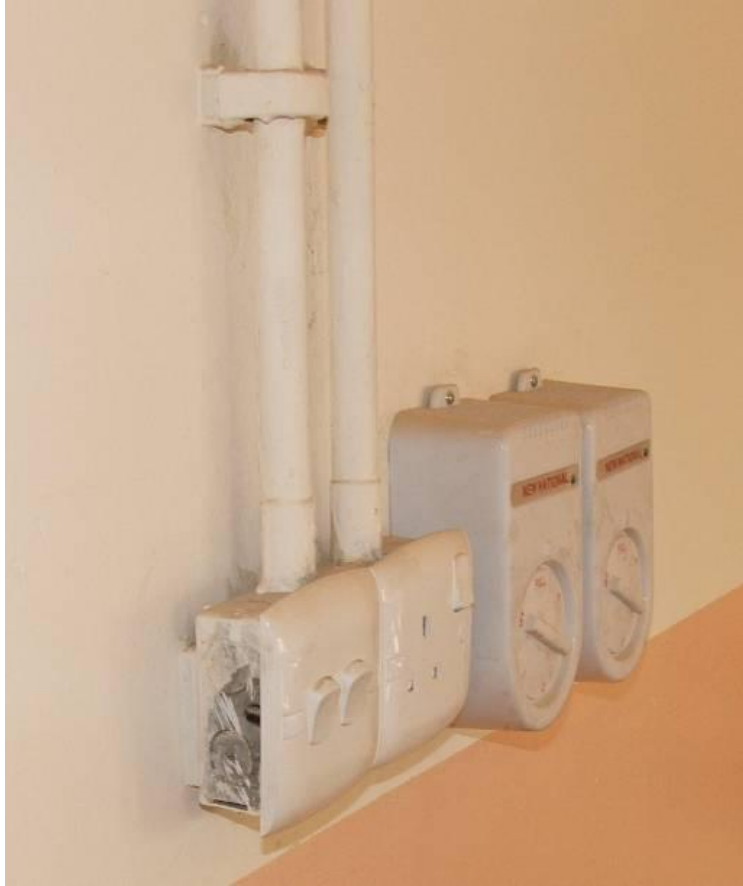
Site Photo 34. Proper electrical installation (Al Faoo) (Note: Paint not fully applied to side of electrical box).
