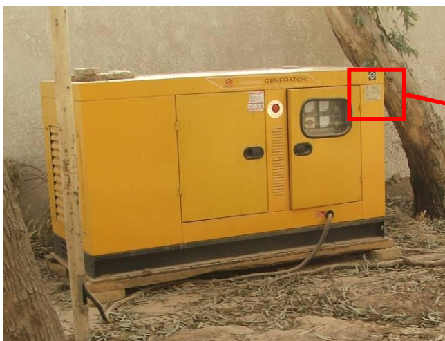
Site Photo 19. Generator (Al Mualameen)
