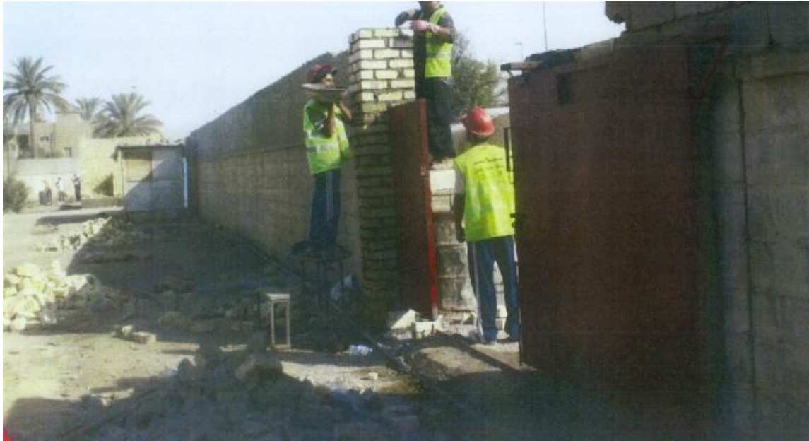
Site Photo 7. Repairing wall at the Al Faoo school (Photo courtesy of MNC-I)
