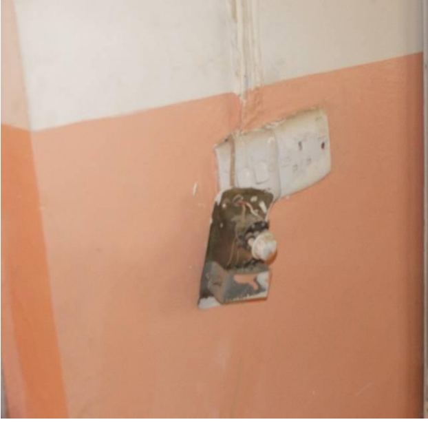
Site Photo 35. Poor electrical installation (Al Mualameen)
