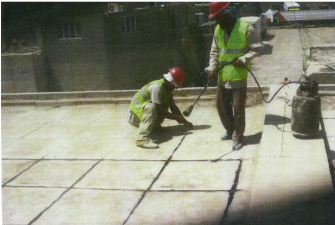
Site Photo 3. Repairing the roof at Al Quds (Photo courtesy of MNC-I)
