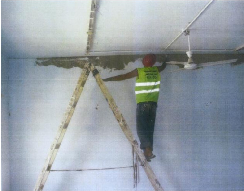
Site Photo 4. Reworking electrical lines & installing fan at Al Quds (Photo courtesy of MNC-I)
