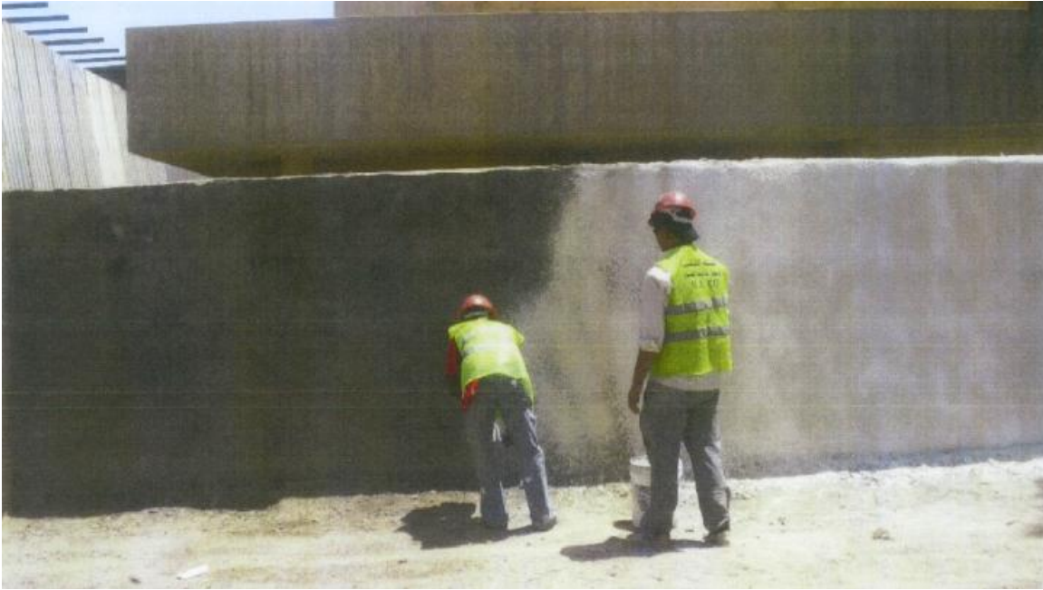
Site Photo 6. Repairing the wall at Al Mualameen (Photo courtesy of MNC-I)
