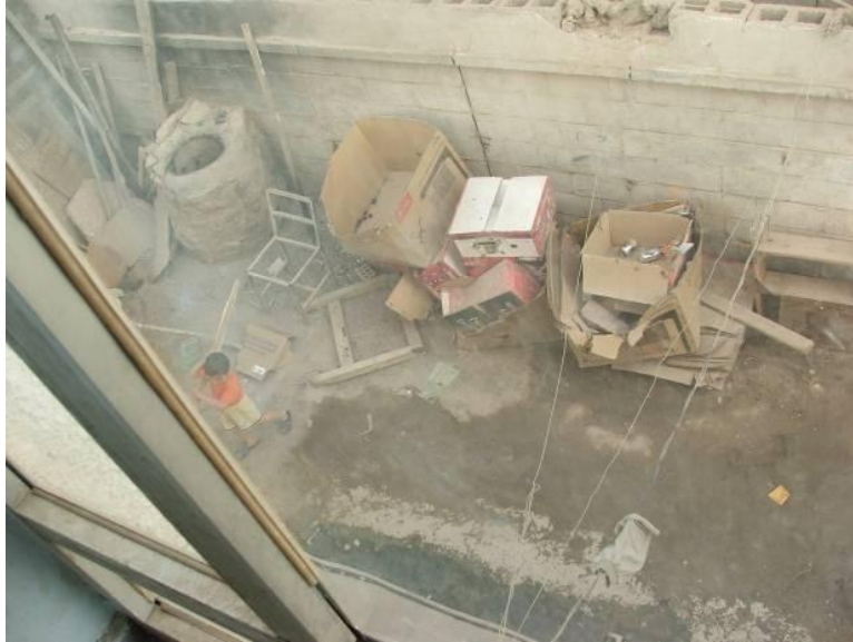
Site Photo 38. Site debris (Al Quds)
