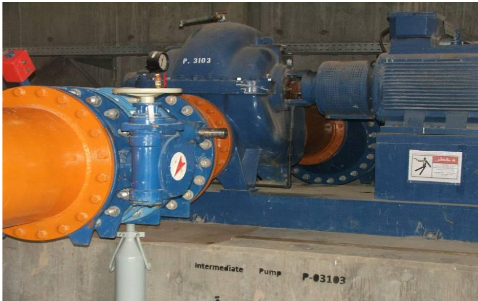
Site Photo 15. Intermediate pump station
