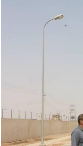
Site Photo 3. Perimeter lighting
