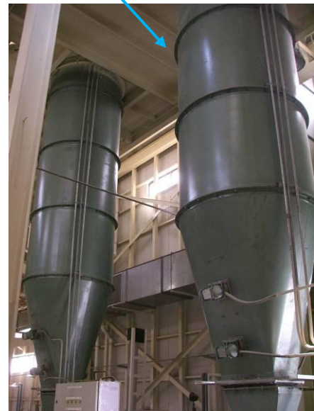
Site Photo 20. Alum storage hoppers
