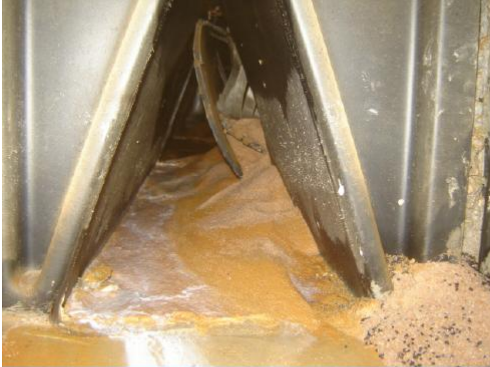
Site Photo 23. Damaged filter under drain
