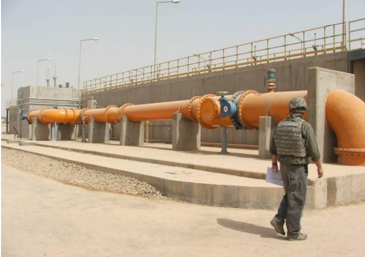
Site Photo 10. 1000-mm raw water inlet piping
