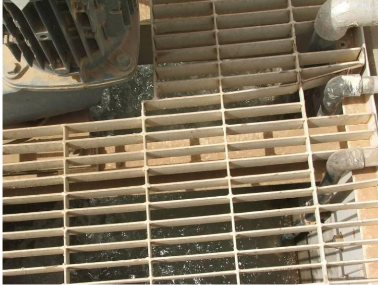
Site Photo 12. Rapid mix tank
