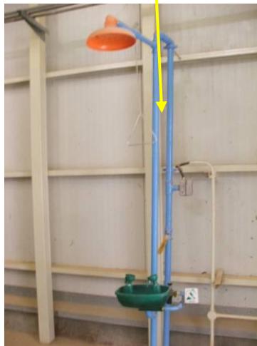
Site Photo 21. Chemical wash and eye flusher
