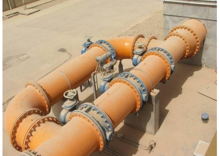
Site Photo 11. Raw water metering and flow control station
