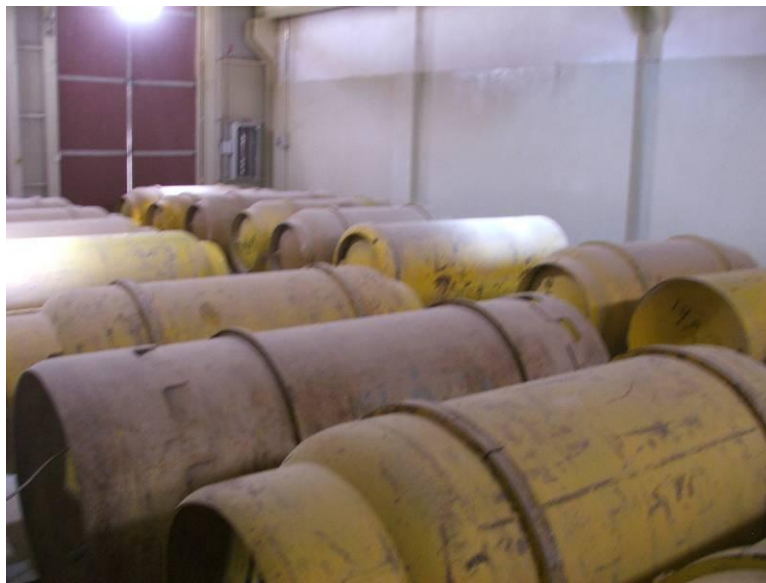
Site Photo 18. Chlorination containers
