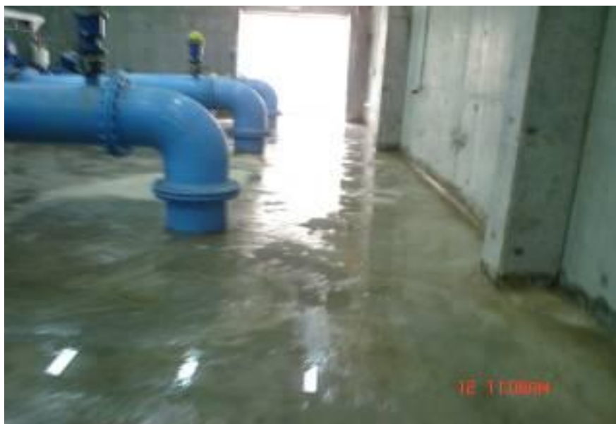
Site Photo 22. Accumulation of water due to floor slope
