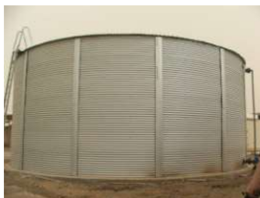
Site Photo 30. Two water storage tanks
