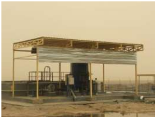
Site Photo 24. Sewage treatment plant
