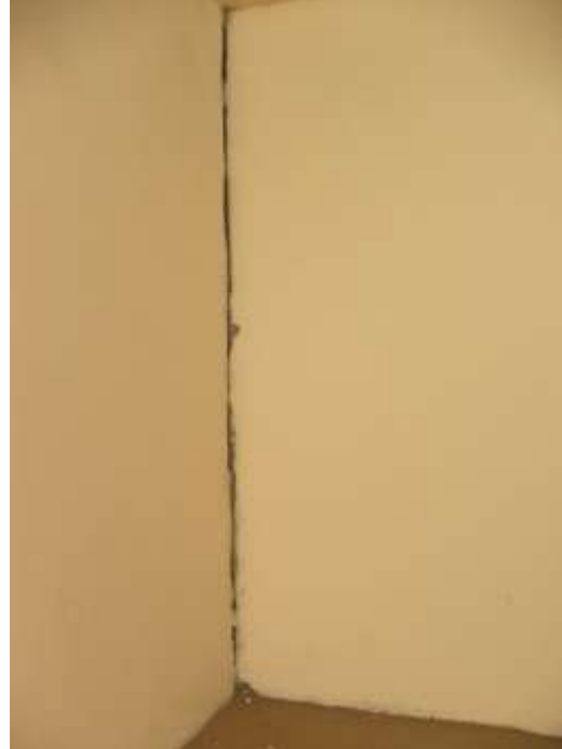
Site Photo 35. Cracked corner of sun room
