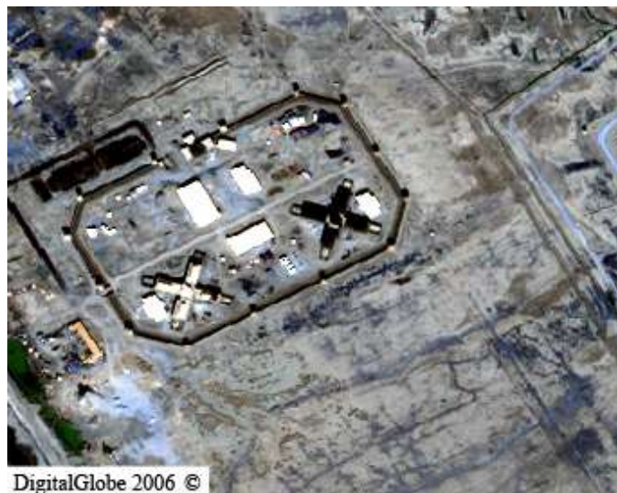
Aerial Image 1. Imagery taken 02DEC06 of the Nassriya Prison Facility under construction.
