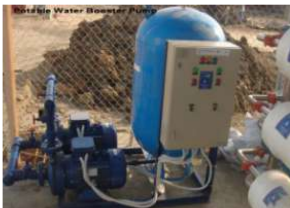
Site Photo 29. Portable water booster pump (Photo courtesy of the USACE)
