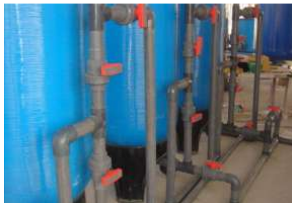
Site Photo 28. Sand filters (Photo courtesy of the USACE)
