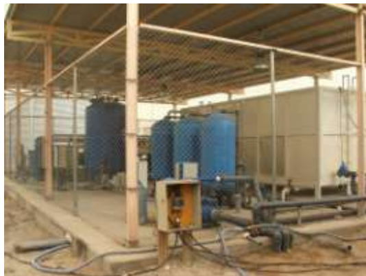
Site Photo 27. Water treatment center
