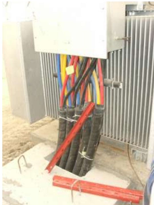
Site Photo 36. Exposed generator cables going to substation plant
