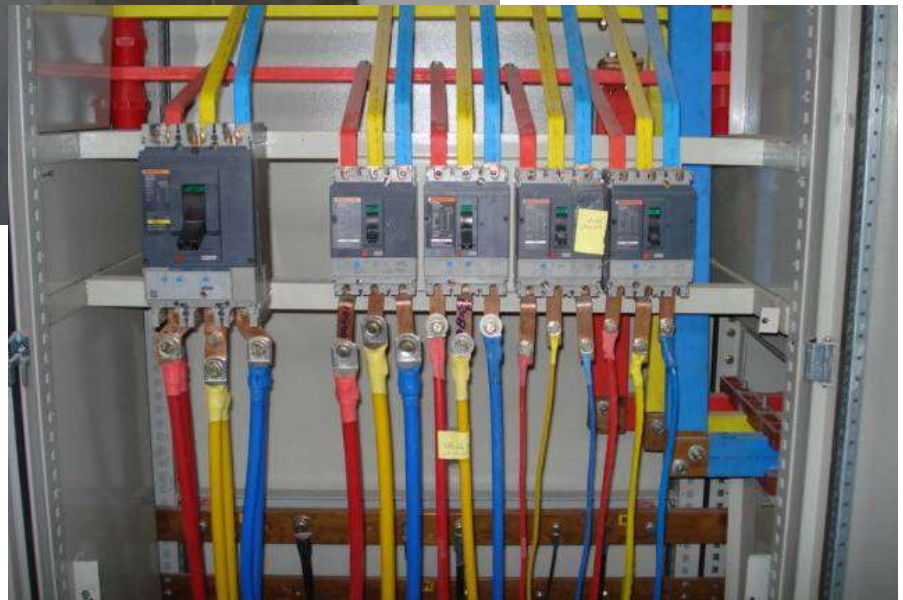
Site Photos 31 and 32. Substation plant transformer side and cables connected to generator (Photos courtesy of the USACE)
