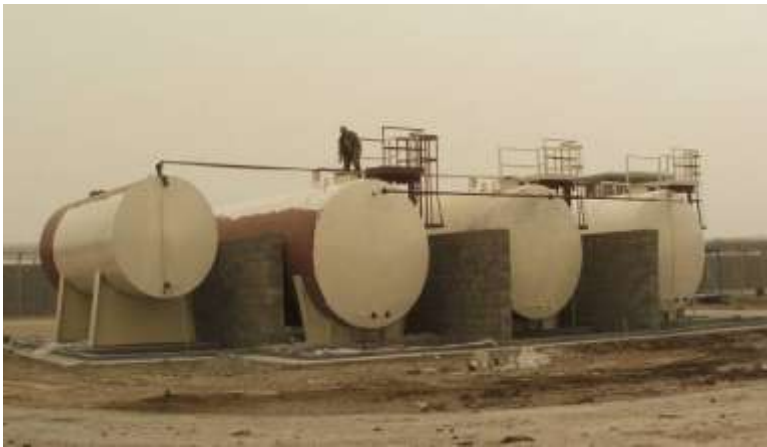
Site Photo 33. Fuel tanks
