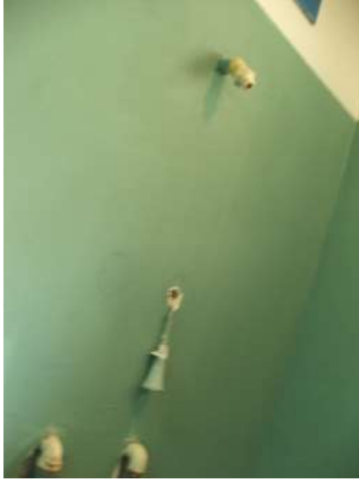
Site Photo 34. Punch list item – missing shower head
