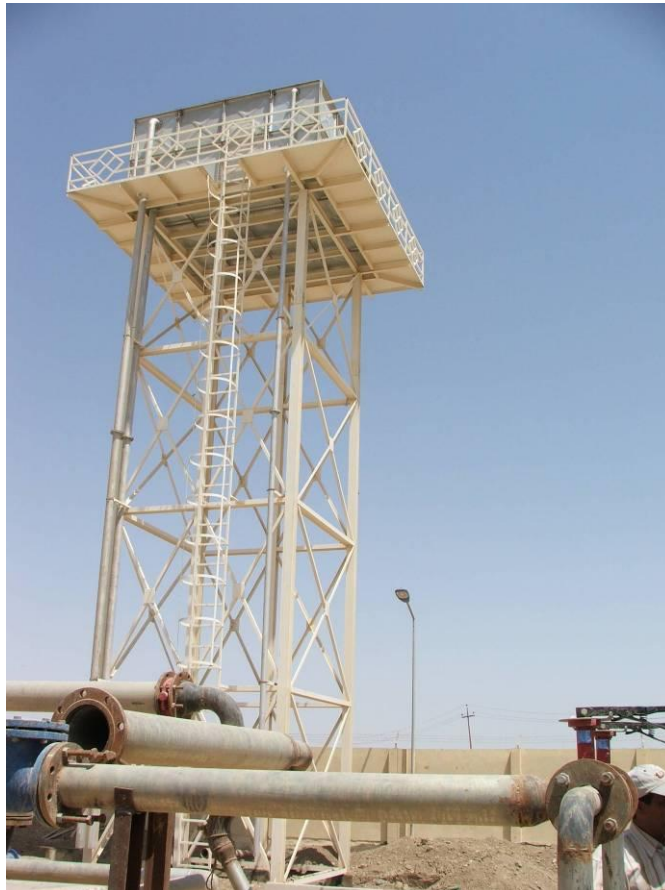
Site Photo 13. Elevated storage tank
