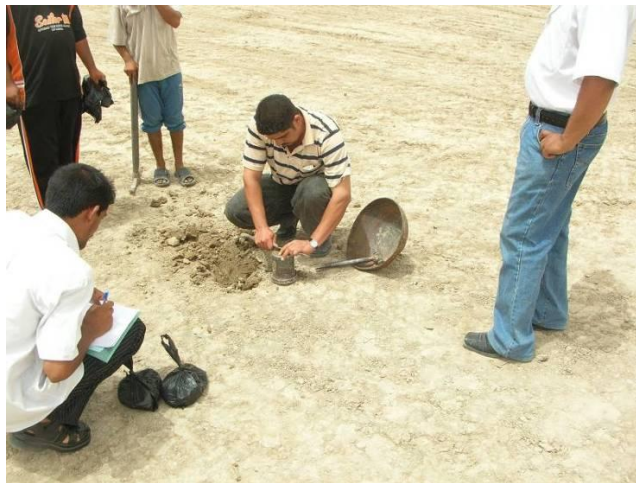
Site Photo 4. Compaction test of first layer of backfill (Courtesy of the USACE)
