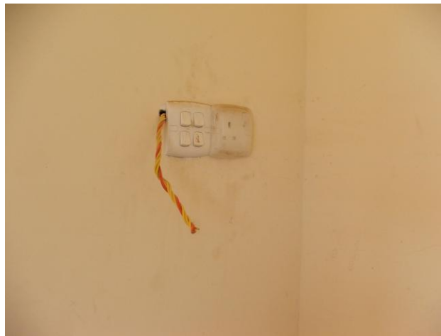
Site Photo 11. Electrical work left unfinished
