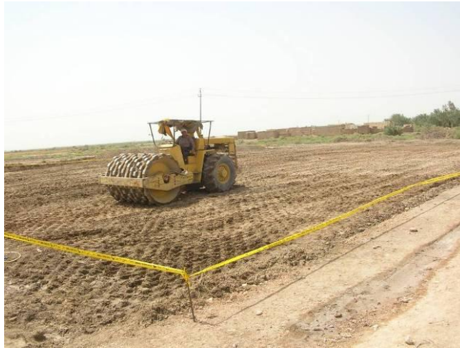
Site Photo 3. Compaction of first layer of backfill (Courtesy of the USACE)
