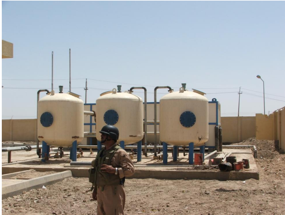
Site Photo 16. Water compact unit without sunshade.
