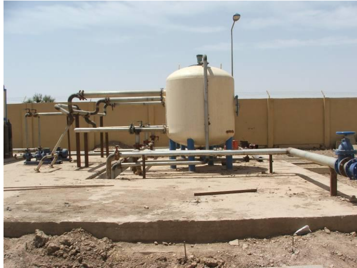
Site Photo 5. Reinforced concrete pad for 50-m 3 /hr compact unit water treatment plant
