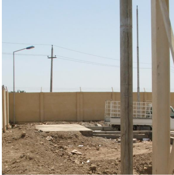
Site Photo 10. Generator and fuel tank concrete foundation
