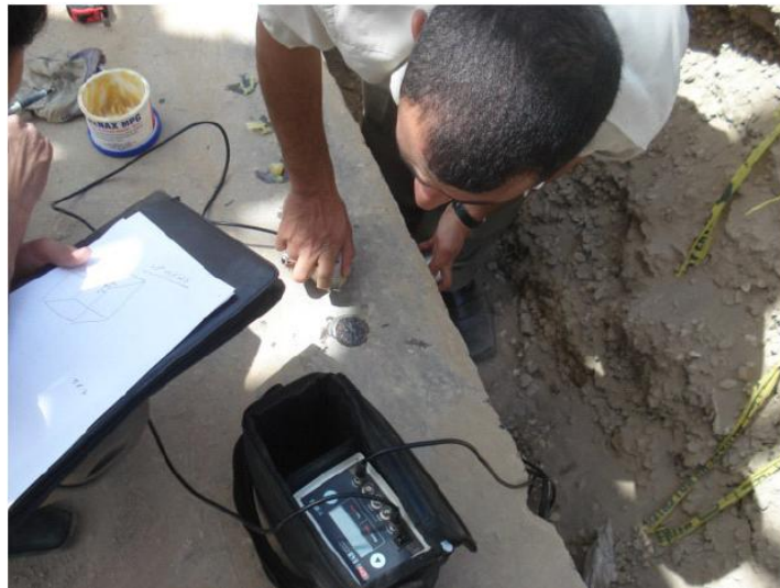
Site Photo 15. Ultrasonic test for elevated storage tank (Courtesy of the USACE)
