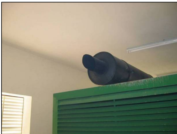
Site Photo 17. Generator exhaust inside the school
