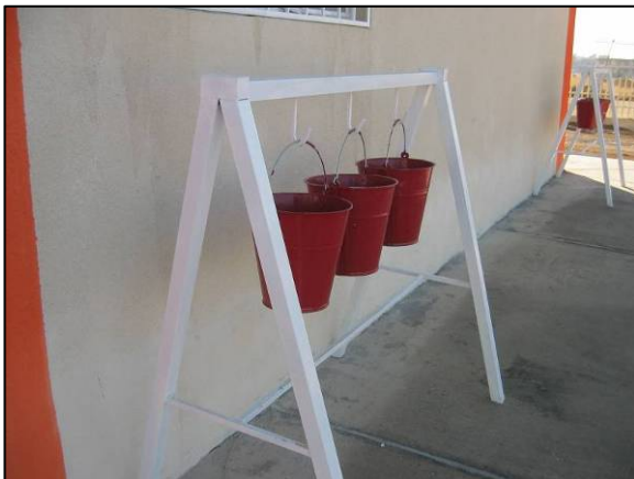
Site Photo 21. Fire bucket racks, the only fire safety equipment observed at the time of the site visit.
