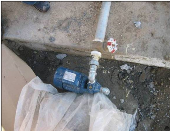
Site Photo 25. Exposed water pump used to fill the main water tower from the city water supply.
