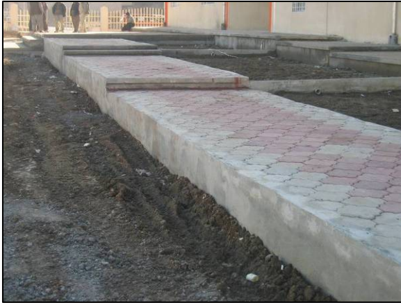
Site Photo 1. Safety hazard at the time of the site visit presented by grading one meter lower than sidewalk
