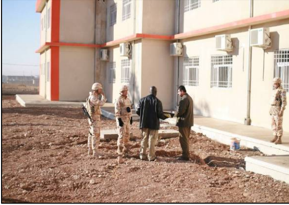
Site Photo 23. Unsecured septic tank and cesspool area with rough and uneven grading.
