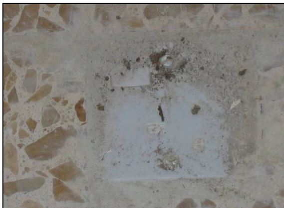
Site Photo 8. Computer room uncovered receptacle filled with dirt.
