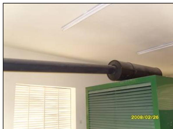
Site Photo 18. Corrective action subsequent to site visit to vent the exhaust out of the building. (Photo courtesy of MND-NE).
