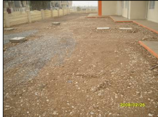
Site Photo 24. Corrective action subsequent to site visit to properly grade the area. (Photo courtesy of MND-NE).
