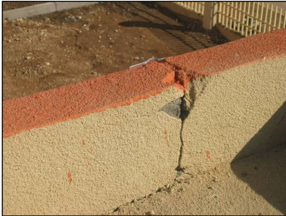
Site Photo 19. Stress crack in concrete covering an expansion joint.
