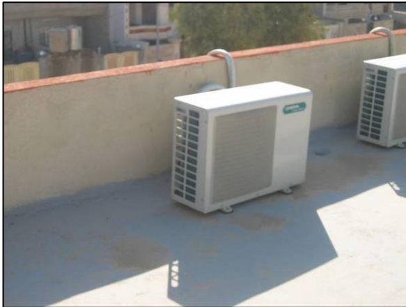
Site Photo 27. Split heating/air conditioning units not anchored.
