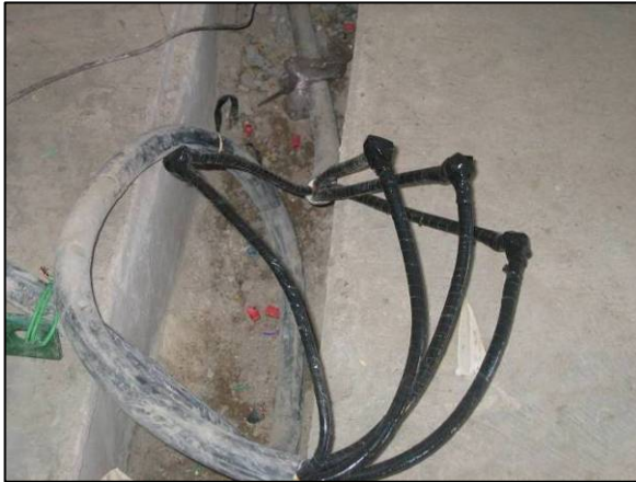
Site Photo 15. Backup generator connection to the school
