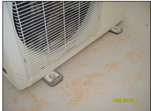
Site Photo 28. Corrective action subsequent to site visit to anchor air conditioning unit . (Photo courtesy of MND-NE).
