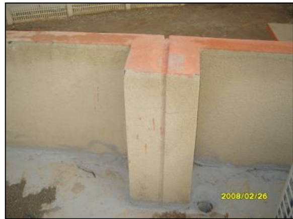
Site Photo 20. Corrective action subsequent to site visit to reconstruct parapet and expansion joint. (Photo courtesy of MND-NE).
