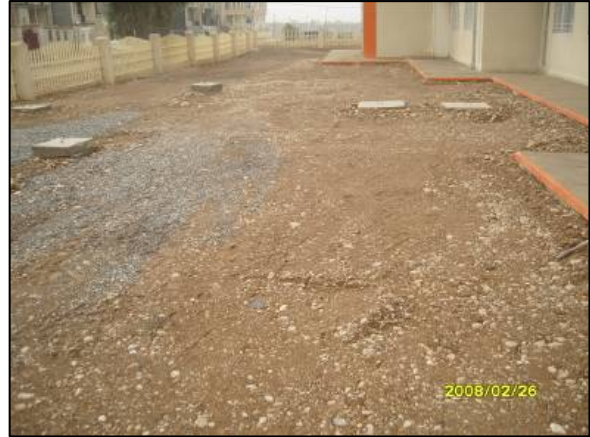
Site Photo 2. Correction of grading and grading level subsequent to site visit (Photo courtesy MND-NE).
