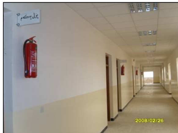
Site Photo 22. Corrective action subsequent to site visit to provide interior fire fighting equipment (Photo courtesy of MND-NE).
