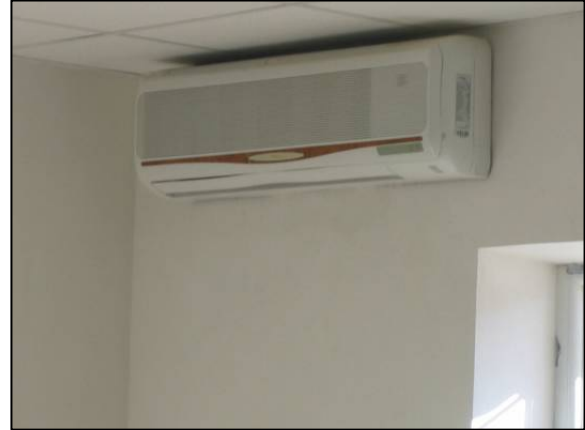
Site Photo 7. Split air conditioning unit
