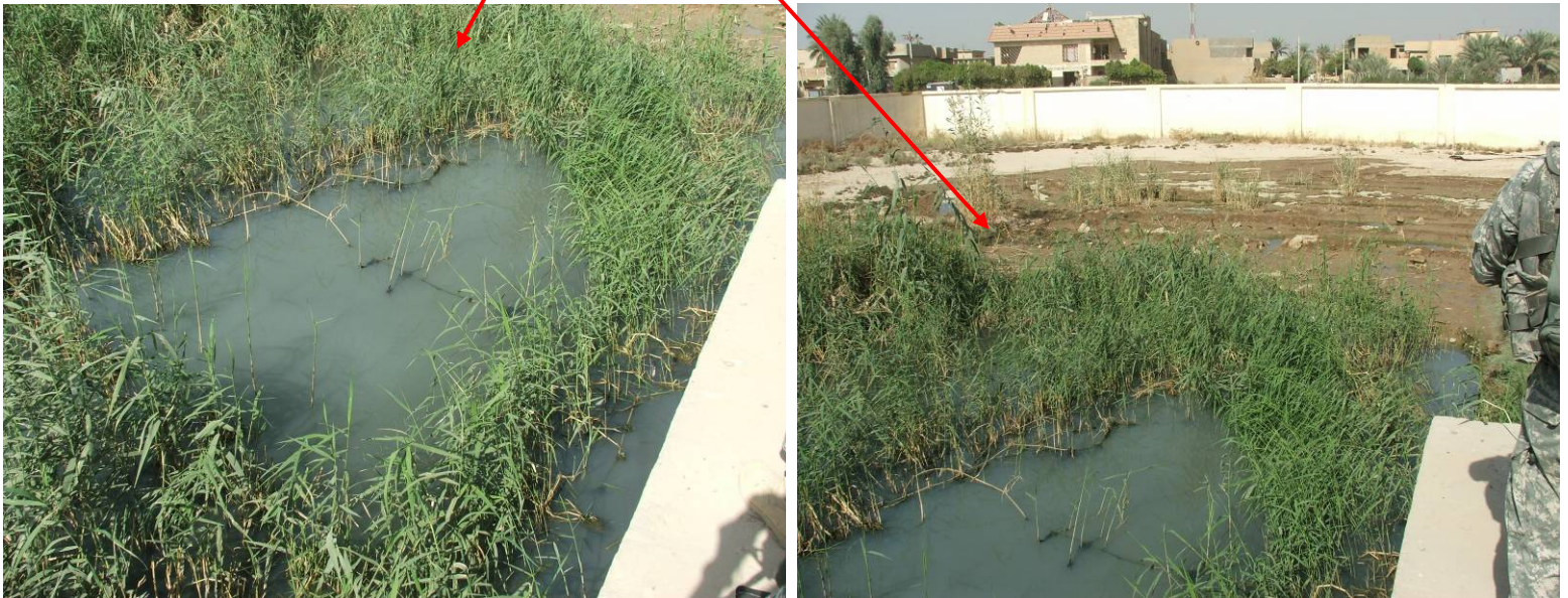
Site Photos 6 and 7. View of pool of accumulated sewage water outside the G-7 lift station
