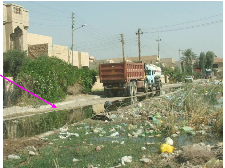
Site Photo 3. Backed-up sewer water
