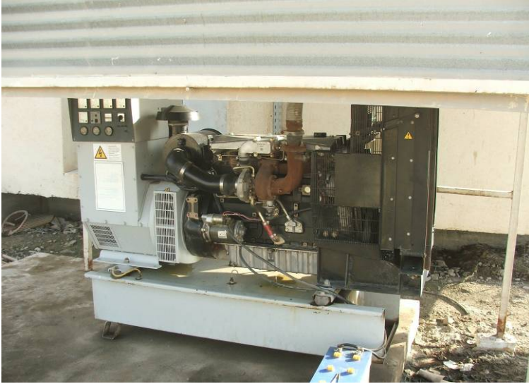
Site Photo 15. Contractor provided 100 kVA generator
