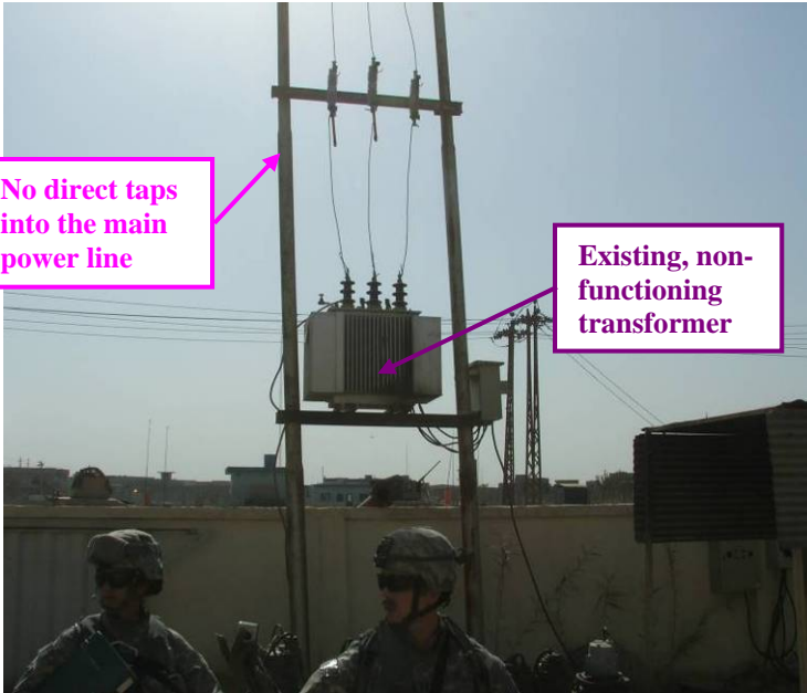
Site Photo 18. Existing transformer
