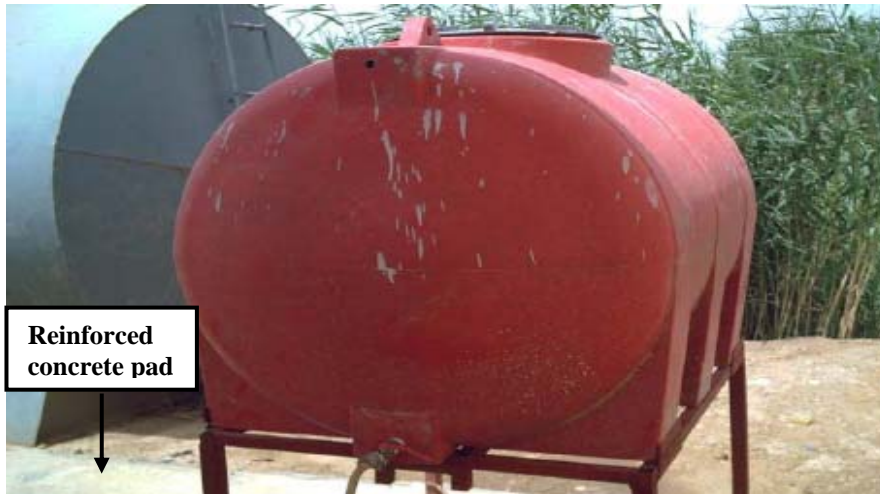
Site Photo 17. 1,000 liter generator fuel tank
