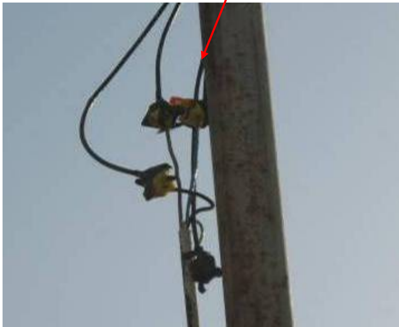
Site Photo 20. Unsafe splices directly into the main power line
