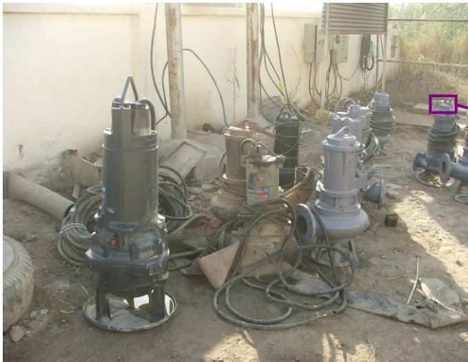
Site Photo 13. Submersible pumps located outside the G-7 lift station
