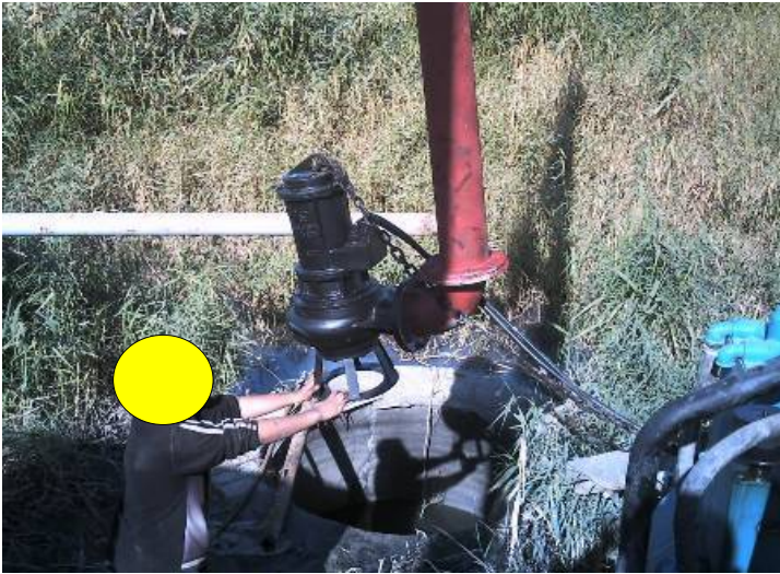
Site Photo 11. Installation of 150 mm submersible pump into manhole outside G-7 lift station (Photo courtesy of USACE)
