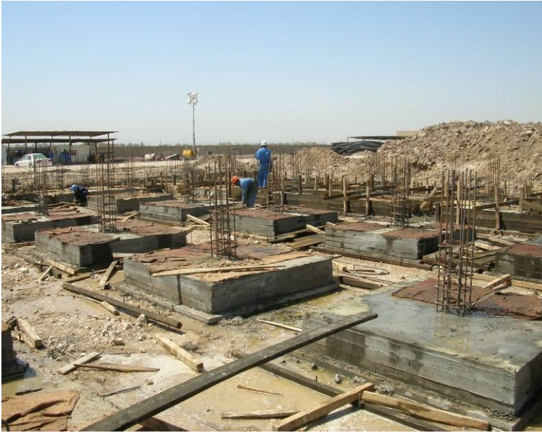
Site Photo 3. Concrete foundation for the chlorination area (Photo courtesy of the USACE)
