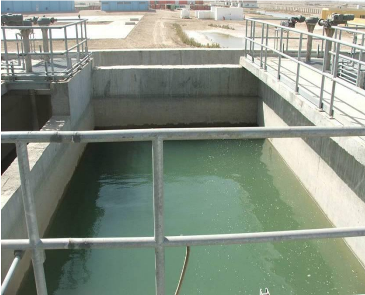
Site Photo 19. Filter tank
