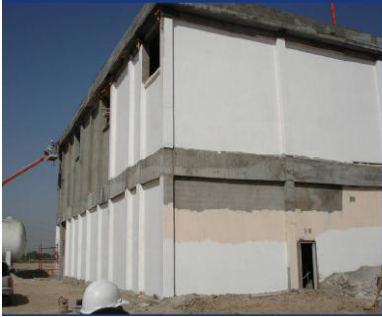
Site Photo 7. Construction of the booster pump station (Photo courtesy of the USACE)
