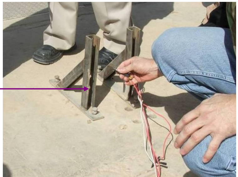
Site Photo 10. Evidence the flow meter was intentionally disabled
