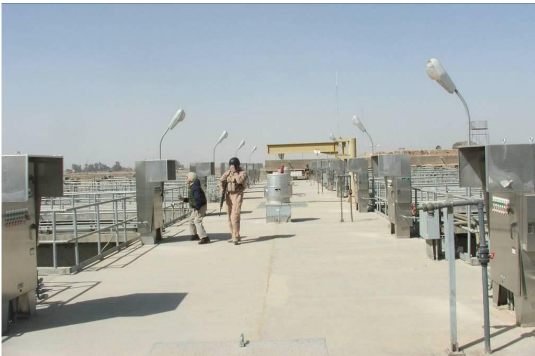
Site Photo 18. Gravity filter control panels
