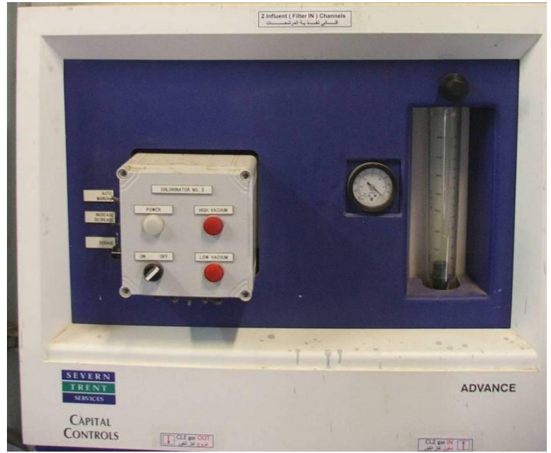
Site Photo 25. Remote chlorine injector
