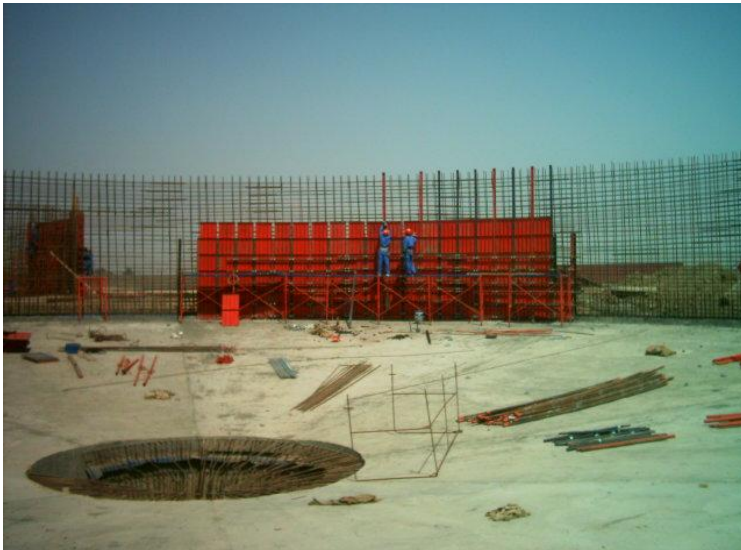
Site Photo 5. Form work for clarifier wall (Photo courtesy of the USACE)
