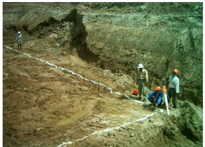
Site Photo 2. Excavation for an elevated storage tank (Photo courtesy of the USACE)
