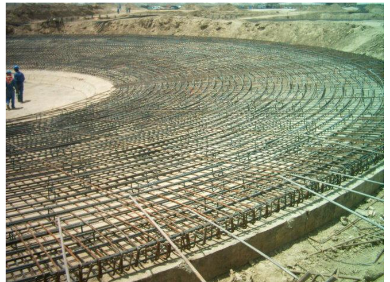
Site Photo 6. Steel reinforcement for clarifier base (Photo courtesy of the USACE)
