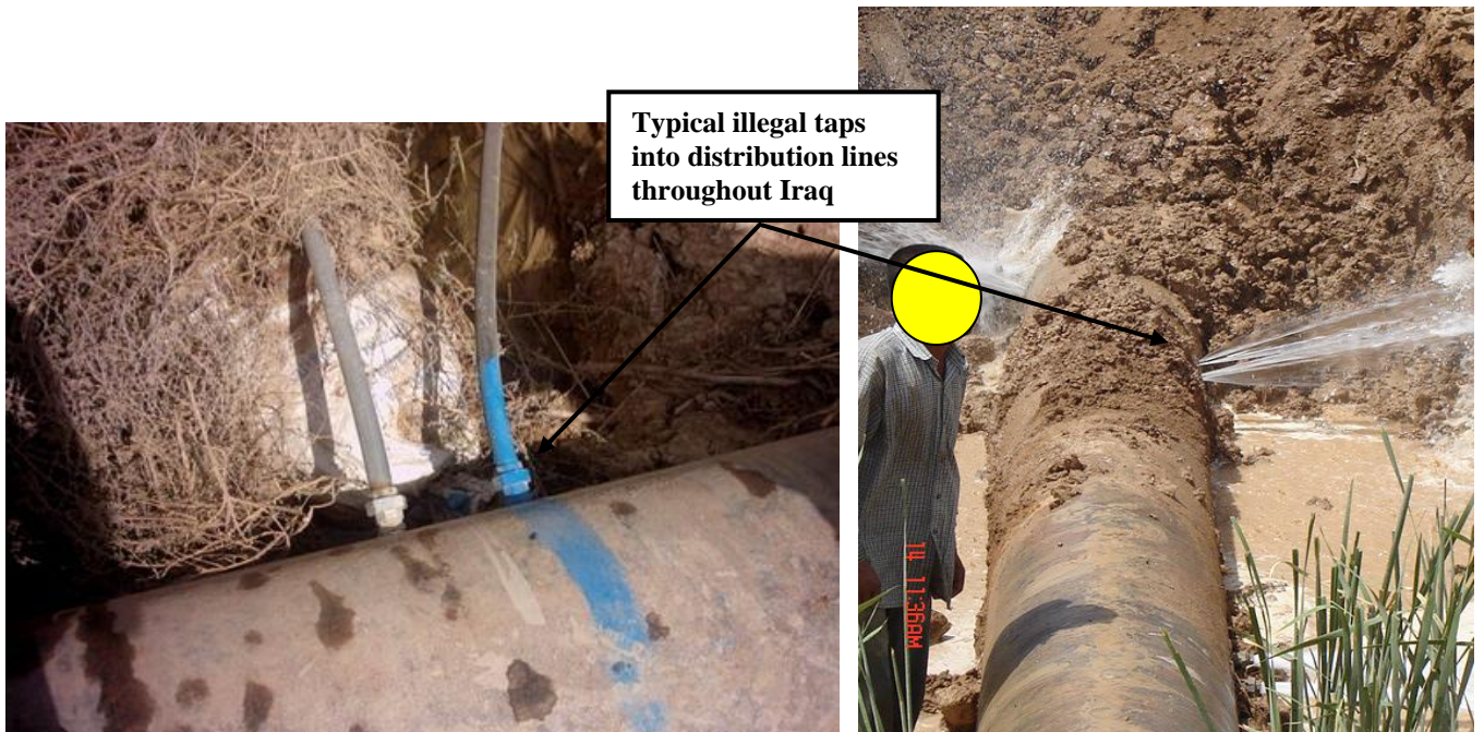
Site Photos 31 and 32. Examples of typical illegal taps and leaks in the distribution lines throughout Iraq
