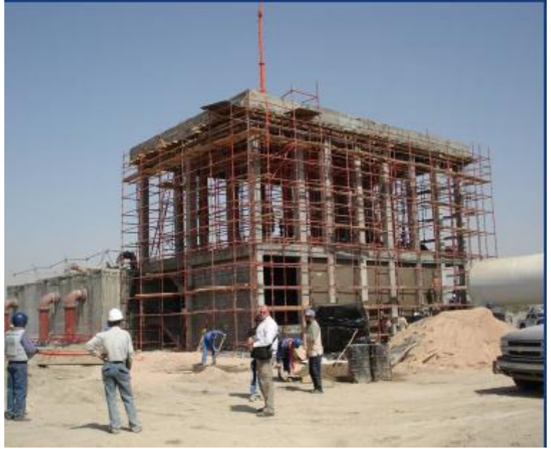
Site Photo 8. Frame for another booster pump station (Photo courtesy of the USACE)
