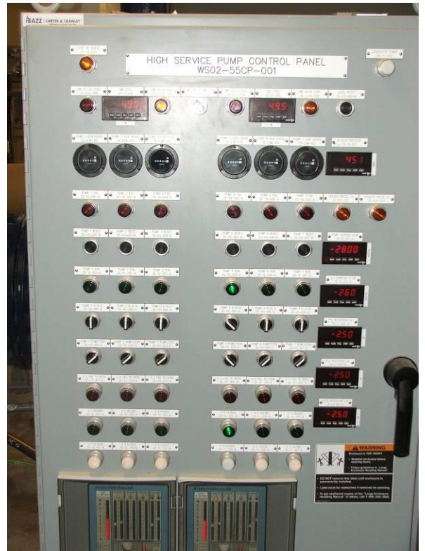
Site Photo 22. High service pump control panel
