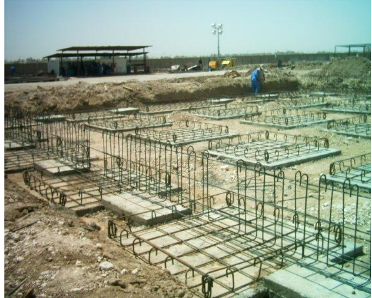
Site Photo 4. Steel reinforcement for the chlorination foundation (Photo courtesy of the USACE)
