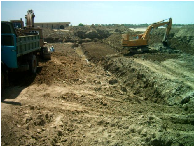
Site Photo 1. Excavation at the WTP site (Photo courtesy of the USACE)
