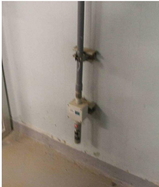
Site Photo 26. Chlorine leak detector
