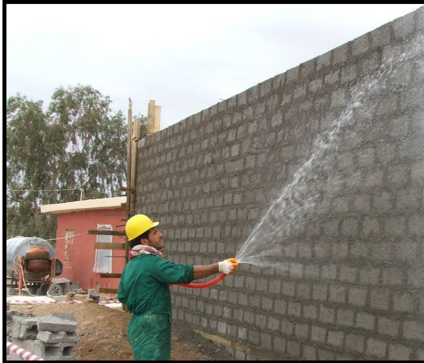
SIGIR Photo 19. Walls were sprayed to prevent excessive shrink in joint mortar.
