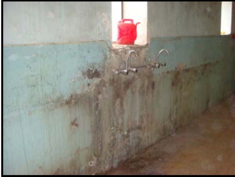
Site Photo 7. Before renovation, food prep areas appeared unsanitary. (Photo courtesy of Toltest)
