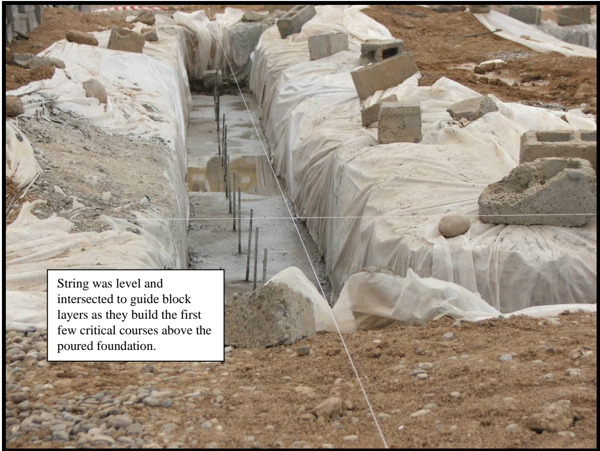
Site Photo 15. String at proper height with square corners will guide block layers.
