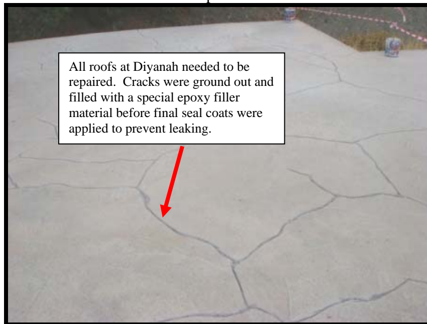
Site Photo 5. Before repair, water leaked through cracks in the original roof. (Photo courtesy of Toltest)
