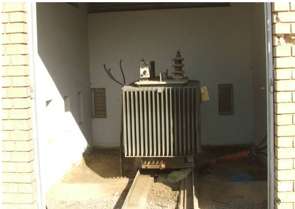
Site Photo 34. Pump station's old and poorly maintained transformer.
