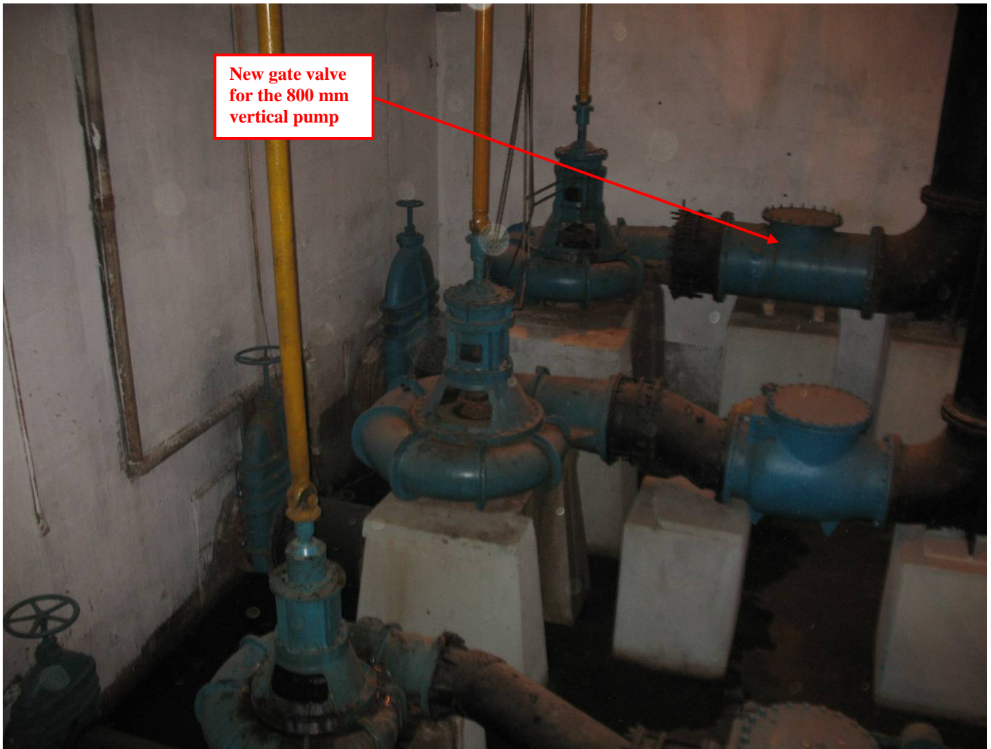
Site Photo 29. View of the vertical pumps within the pump station dry well
