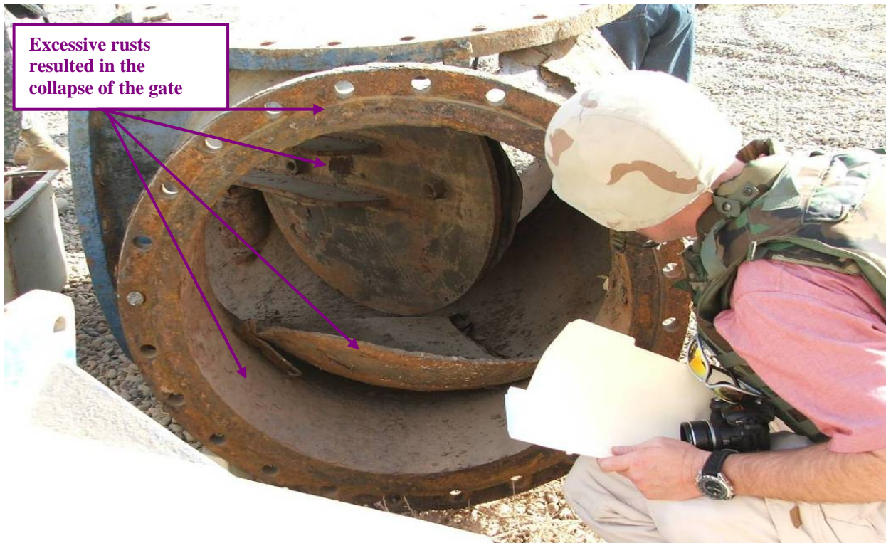
Site Photo 30. View of the original gate valve for the 800 mm vertical pump
