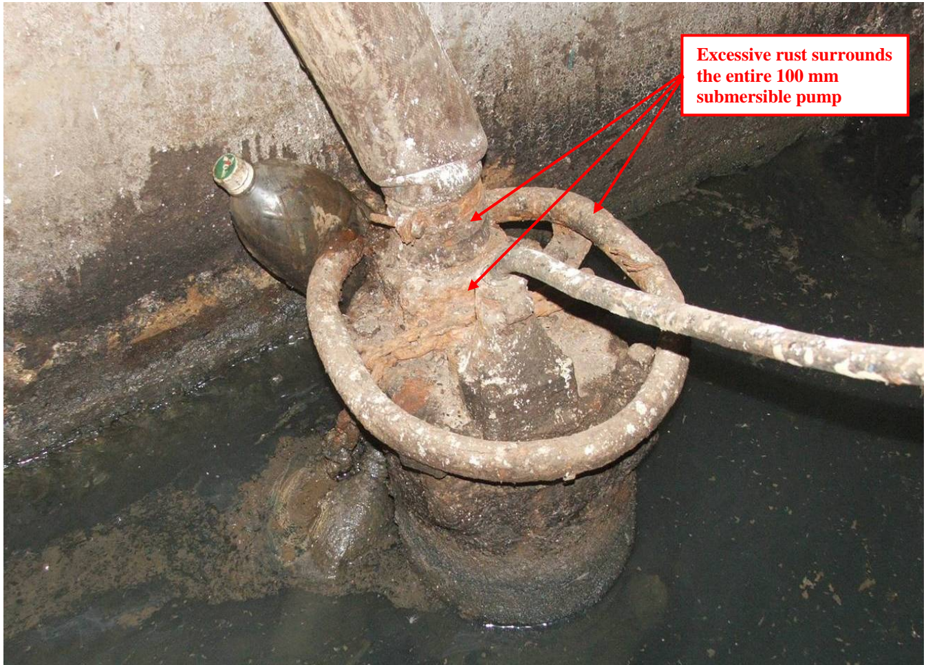
Site Photo 17. Heavily rusted and corroded 100 mm submersible pump
