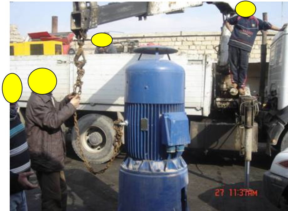
Site Photo 5. Delivery of the new motor for the 350 mm vertical pump. (Photo courtesy of USACE)
