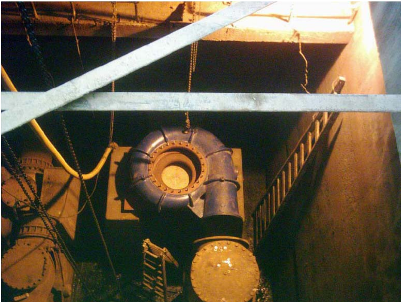
Site Photo 21. Photograph from daily QA report documenting contractor progress installing the 800 mm vertical pump (Photo courtesy of the USACE)
