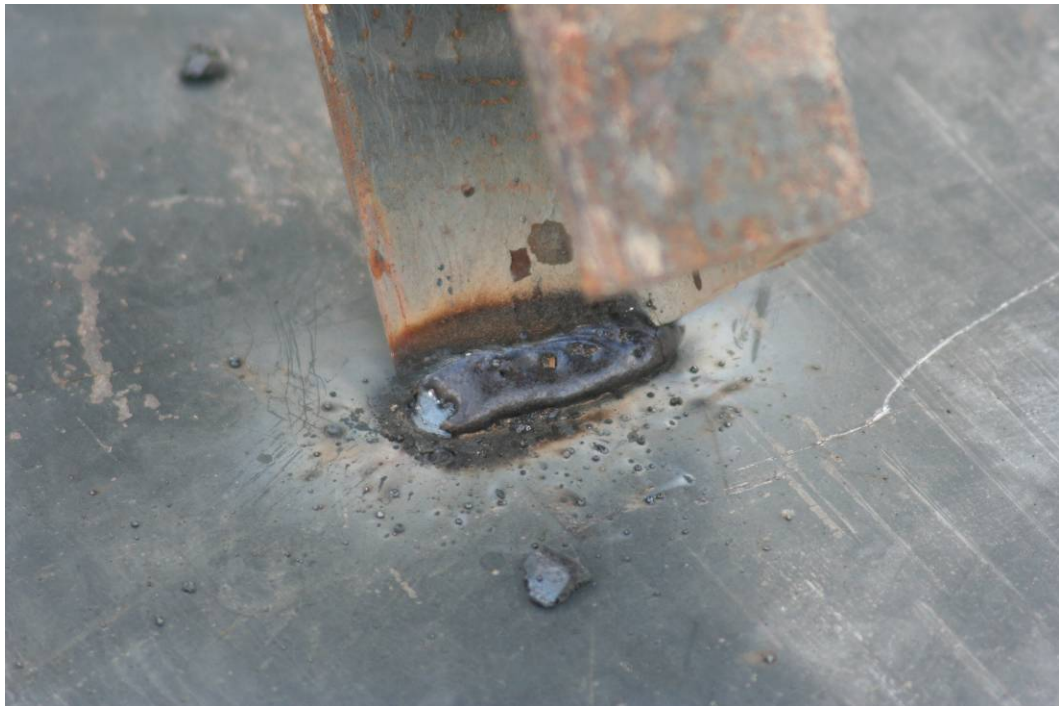
Site Photo 19. Bottom ends of steel beams are tack welded to the floor plates.
