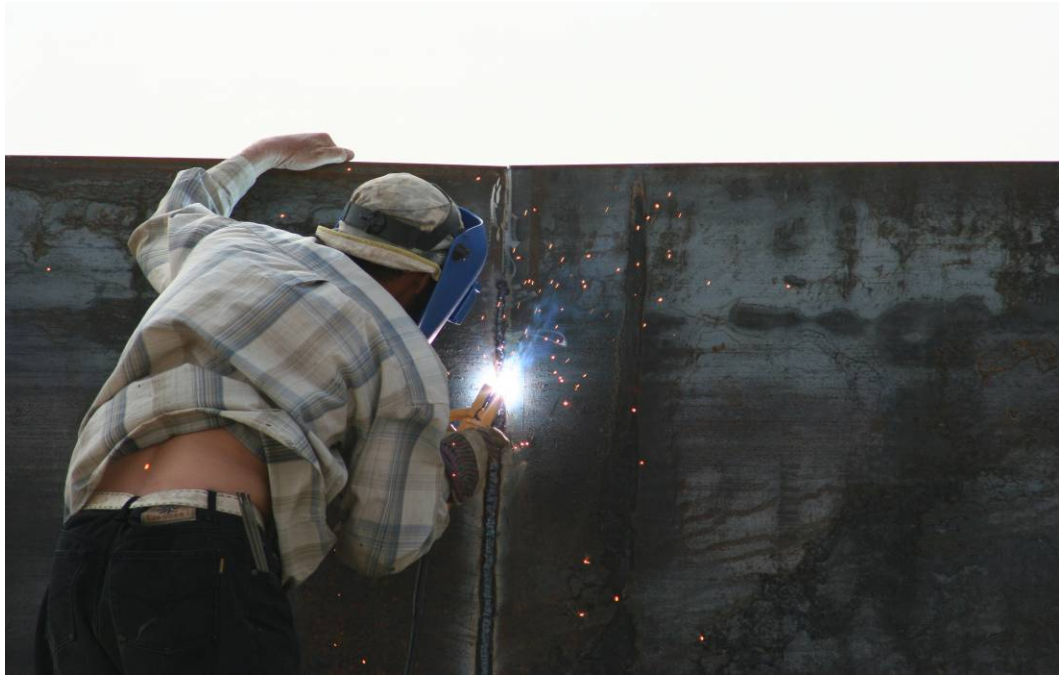
Site Photo 23. Worker completes second run vertical weld on a shell plate.
