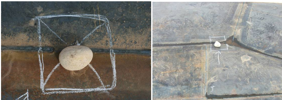
Site Photos 10 and 11. Stones and chalk mark leaks in the steel plating.
