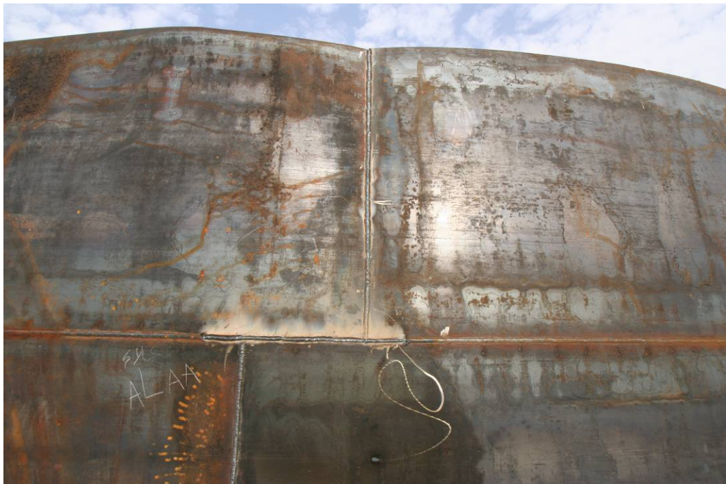
Site Photo 24. Completed second run on a vertical weld of a shell plate.
