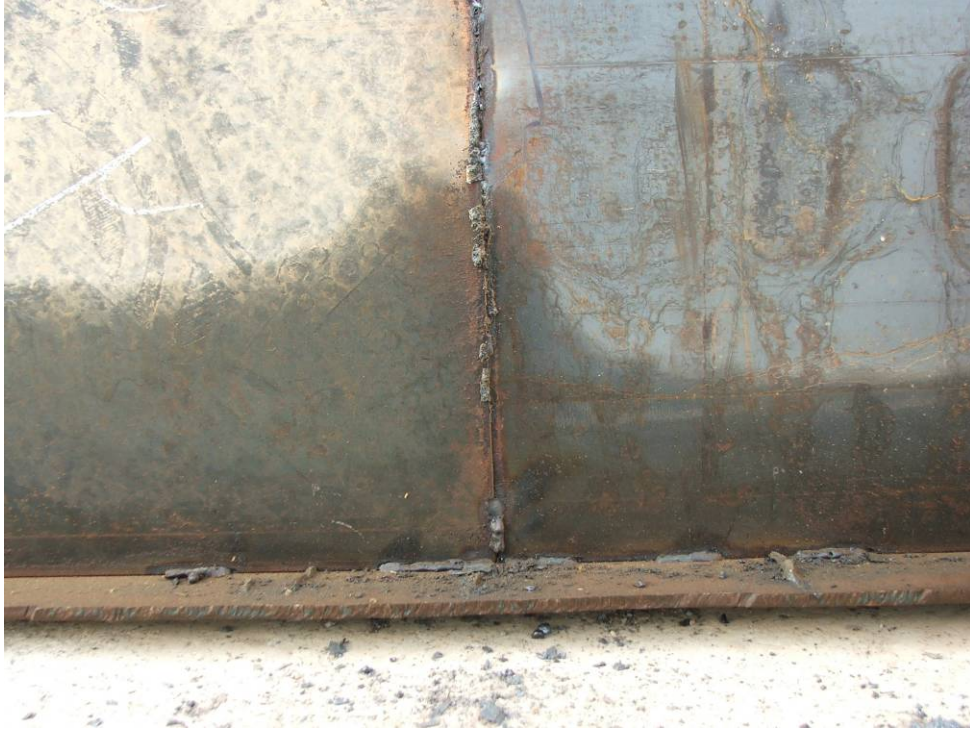
Site Photo 15. Diesel penetrated the welds within 24 hours of test.
