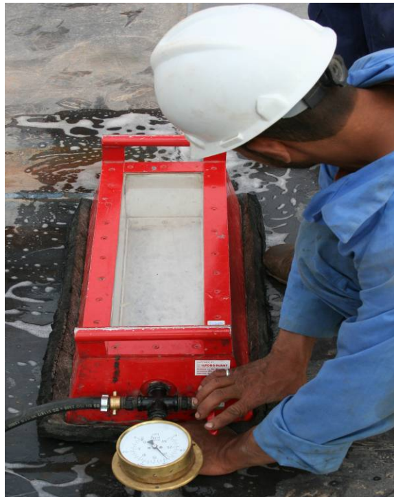
Site Photo 8. A vacuum box was used to test for leaks along floor welds.
