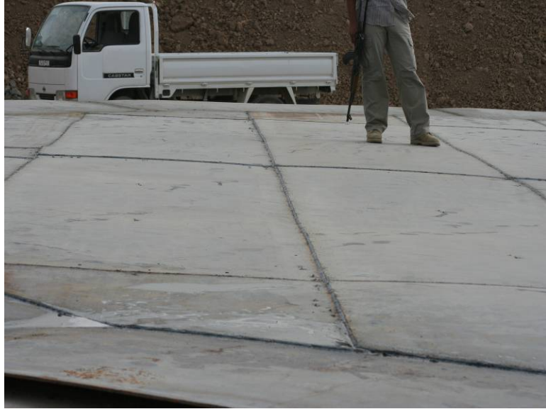
Site Photo 7. After fitting, the sheets were welded along seams to form a sealed tank floor.
