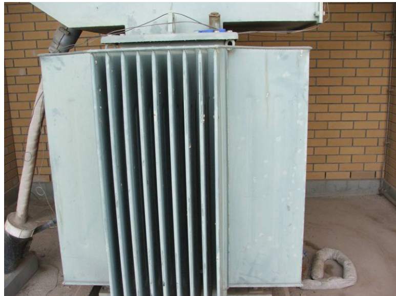
Site Photo 4: Transformer located at S-330
