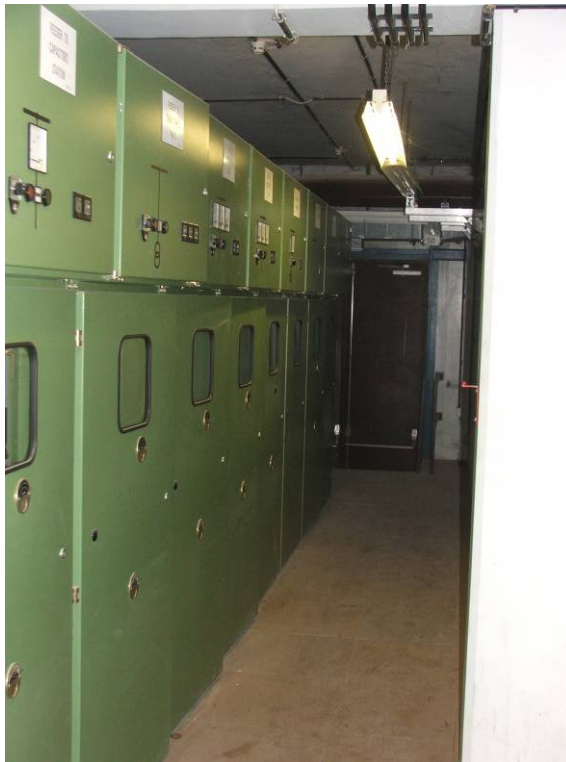
Site Photo 2: Exterior view of 33 kV to 11 kV switchgear cabinets
