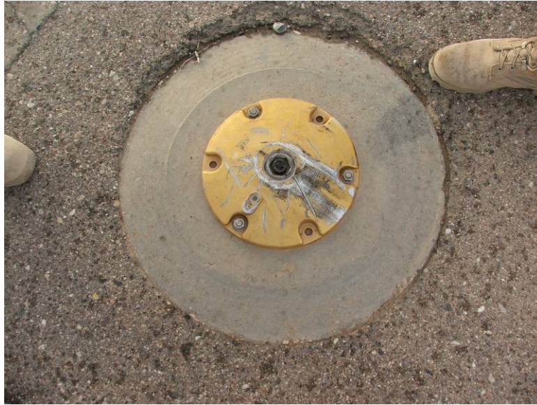
Site Photo 7: Runway light (VISAID)
