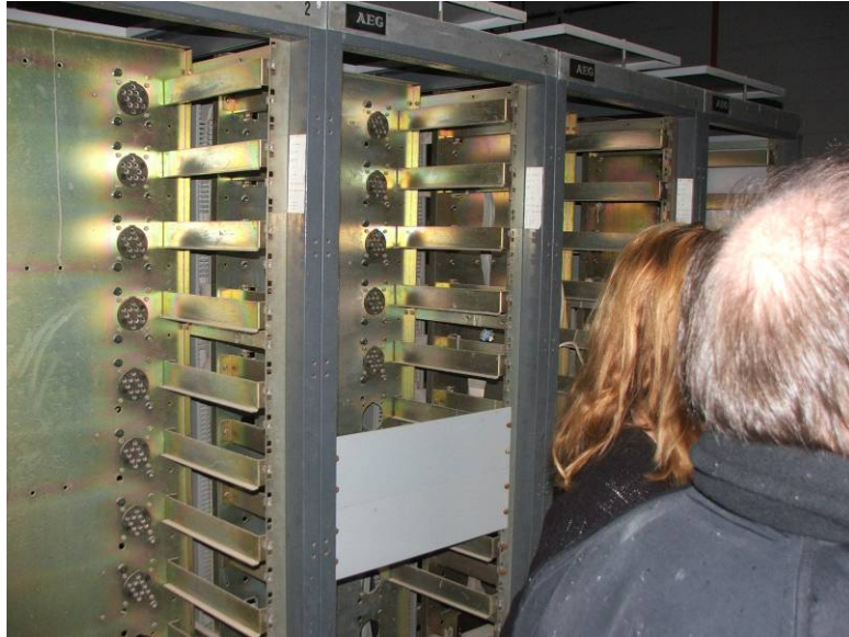
Site Photo 5: Missing electronic equipment at S-330
