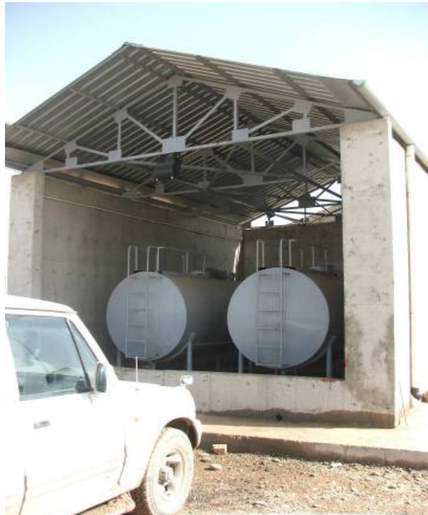
Photo 14. Central fuel supply
