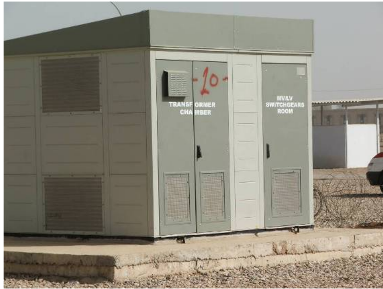
Photo 13. Electrical transformers and switchgears
