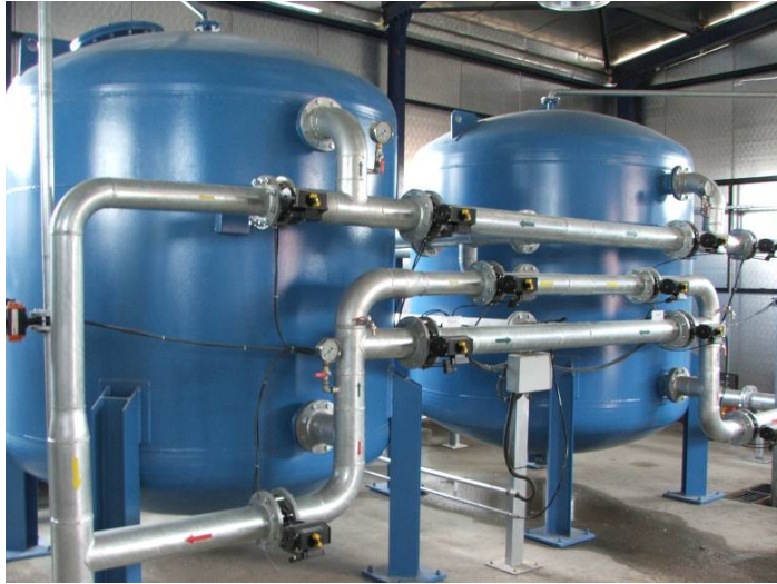
Site Photo 15. Tanks enclosing the 15 micron filters
