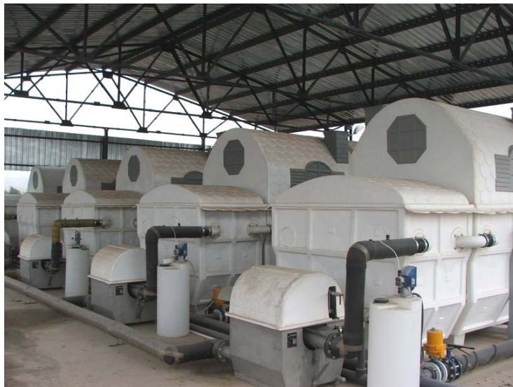
Site Photo 17. Five RBC units for treating domestic wastewater at the WWTP
