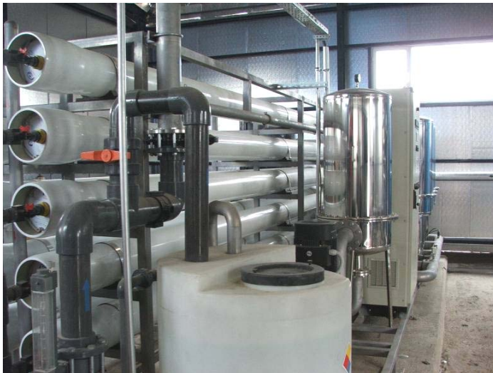
Site Photo 16. Reverse osmosis purification units
