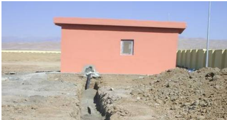
Site Photo 18. Water main installation from new well house – Photo provided by USACE
