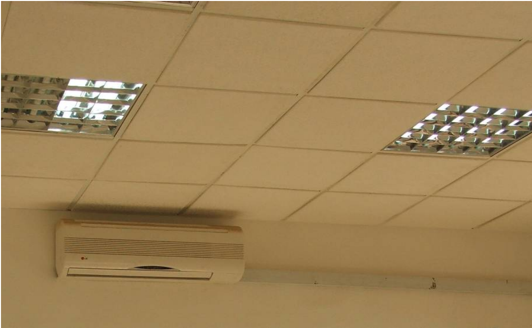
Site Photo 3. Interior Recessed Lighting and False Ceiling
