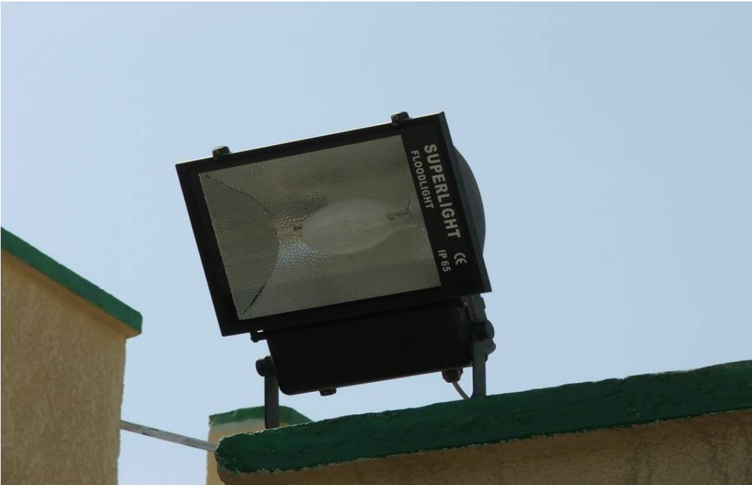
Site Photo 2. Mounted Exterior Light Unit
