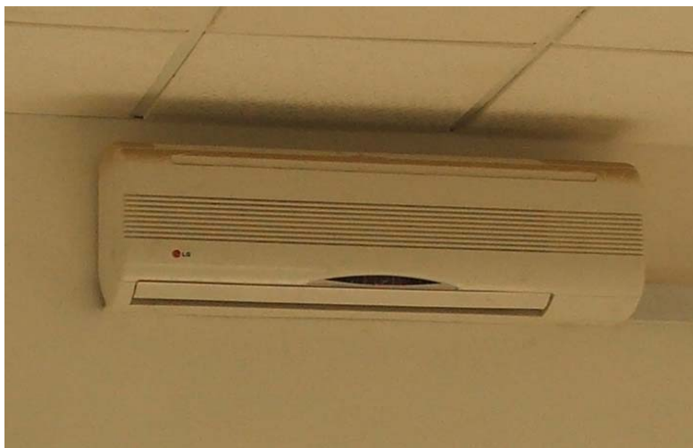
Site Photo 5. Interior Split A/C Cooling/Blower Unit
