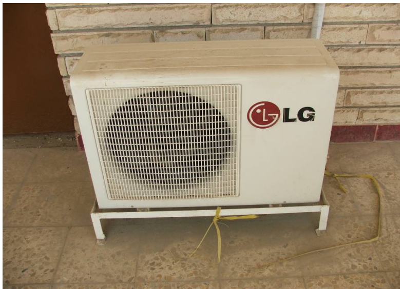
Site Photo 4. Exterior Split A/C Condensing Unit
