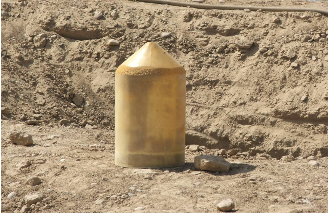
Site Photo 6: 20-Inch Pig
