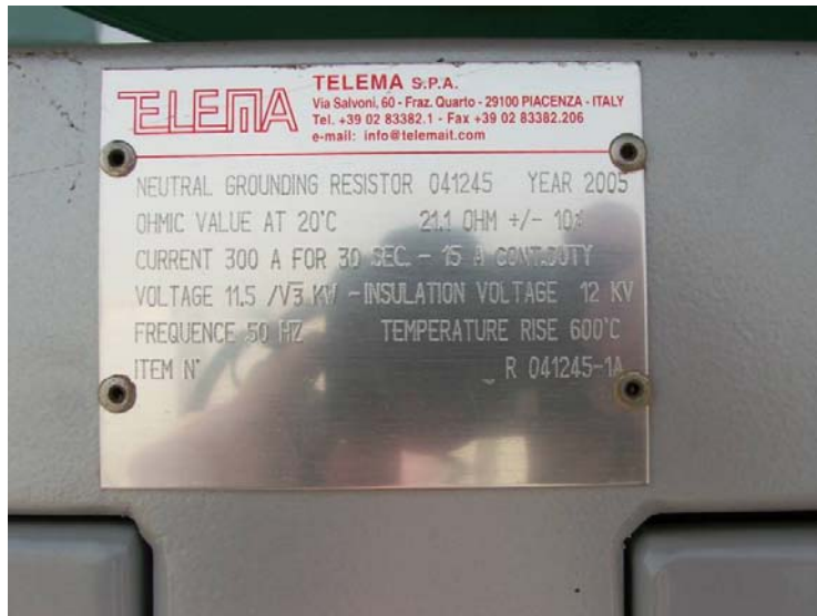
Site Photo 8: Factory nameplate of grounding system
