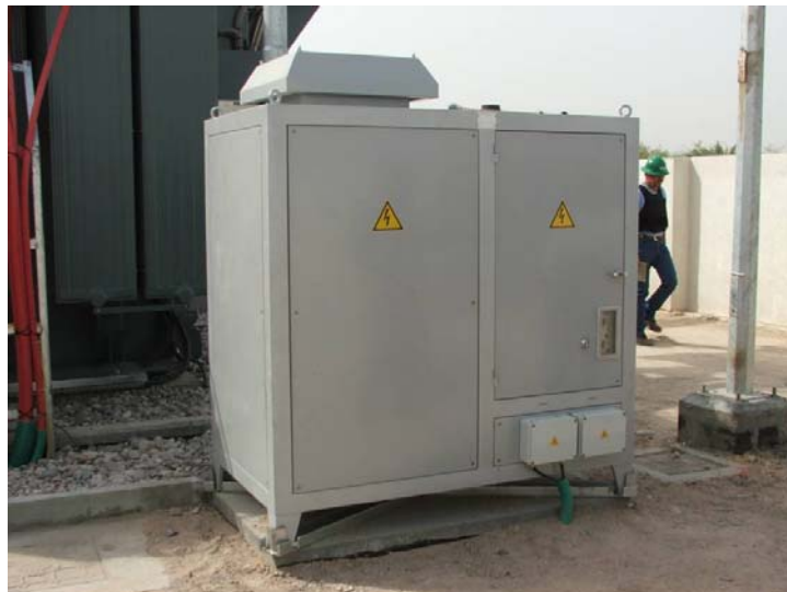
Site Photo 7: Grounding system
