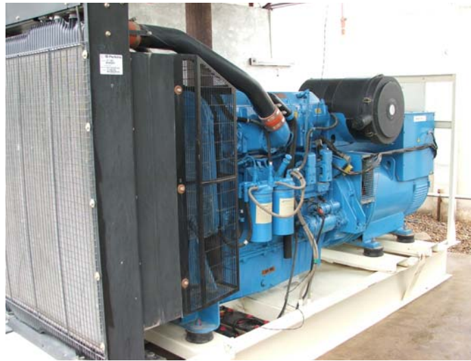
Site Photo 15: 615 KW Generator at the Hilla Police Academy
