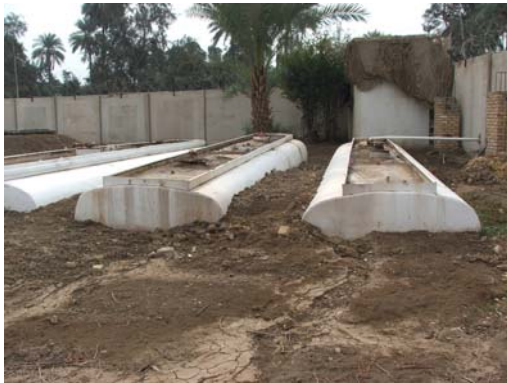
Site Photo 3. Partially Buried Wastewater Tank
