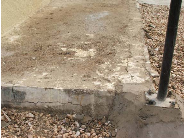
Site Photo 10. Rough Surface Texture and Cracks in Concrete Sidewalk
