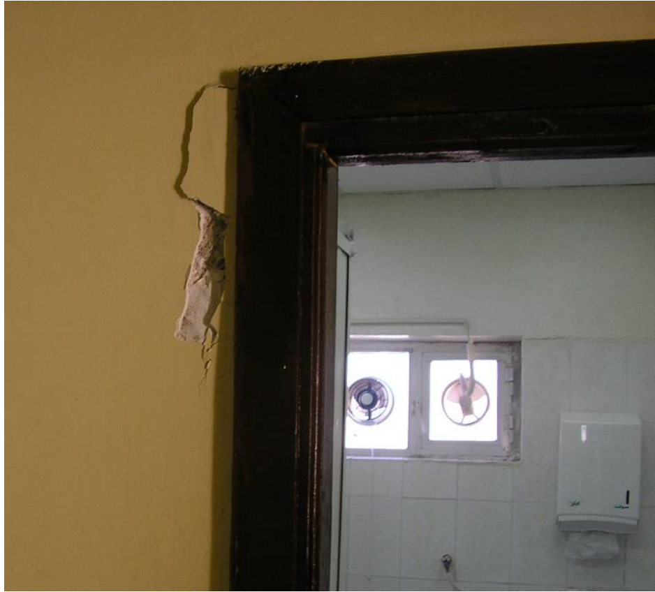
Site Photo 7. Crack in Hallway Wall in Instructor Billeting Area (Photo courtesy of Contracting Officer Representative; taken on 9 December 2005)
