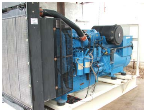
Site Photo 1. 615 Kilowatt Generator
