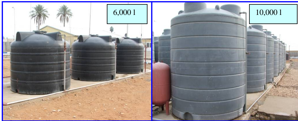
Site Photo 5. Water Storage Tanks
