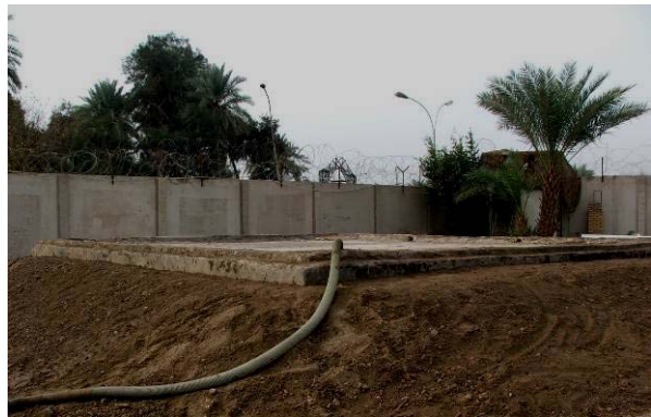
Site Photo 4. Underground Wastewater Tank
