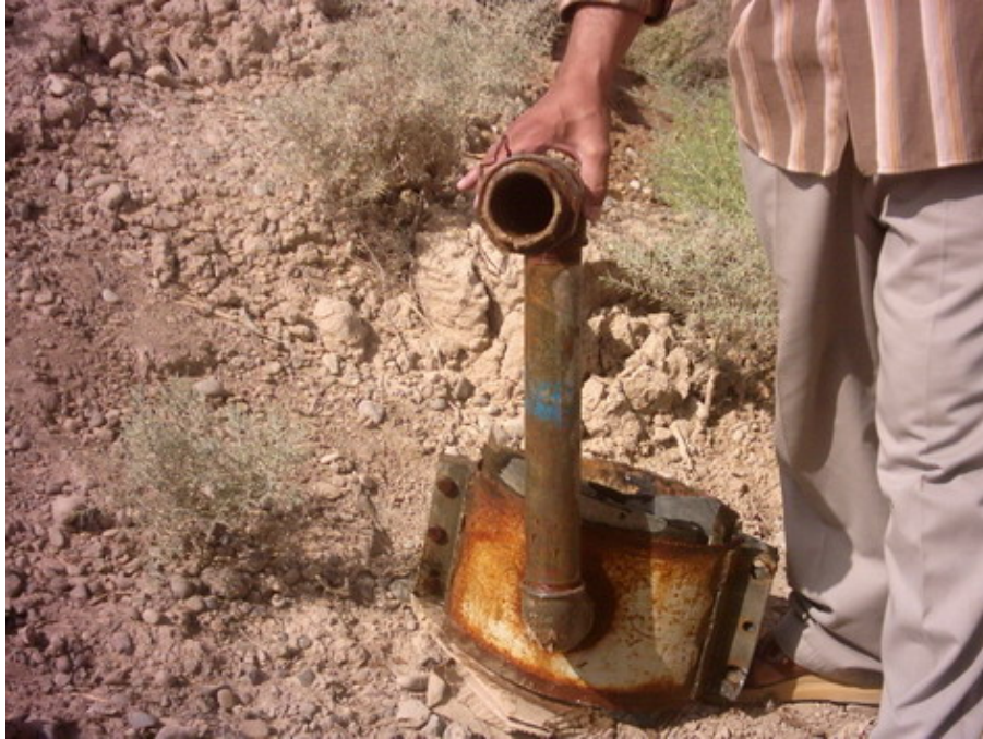
Photo 6: Illegal connection (saddle used to tap into water main)
