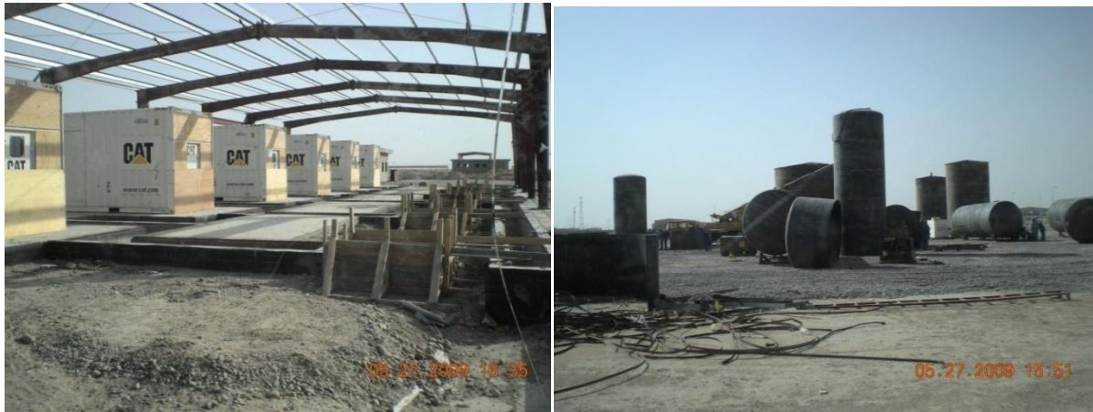
Figure 5—Diesel Generators and Fuel Tanks
