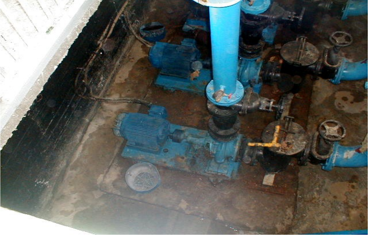
Photo 3. Al Hillah Olympic Swimming Pool Pumps
