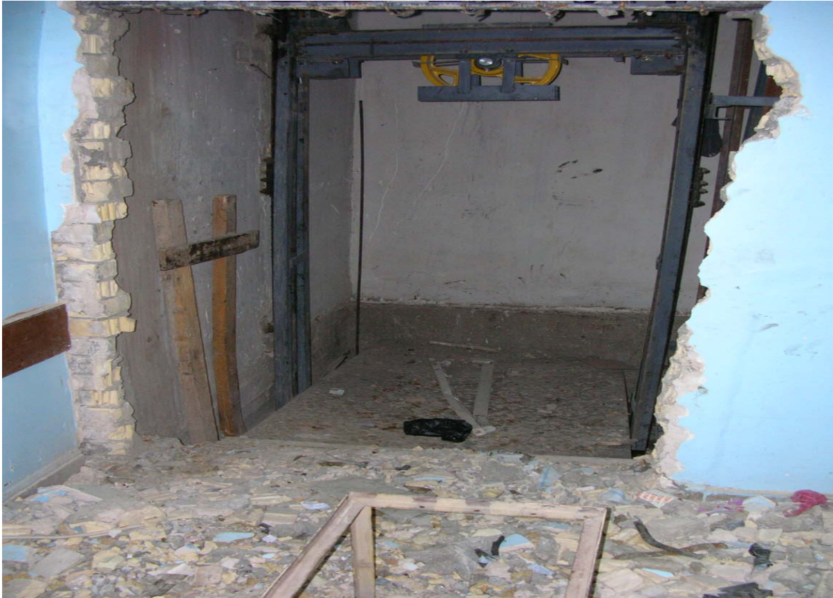
Photo 2. Al Hillah General Hospital Elevator
