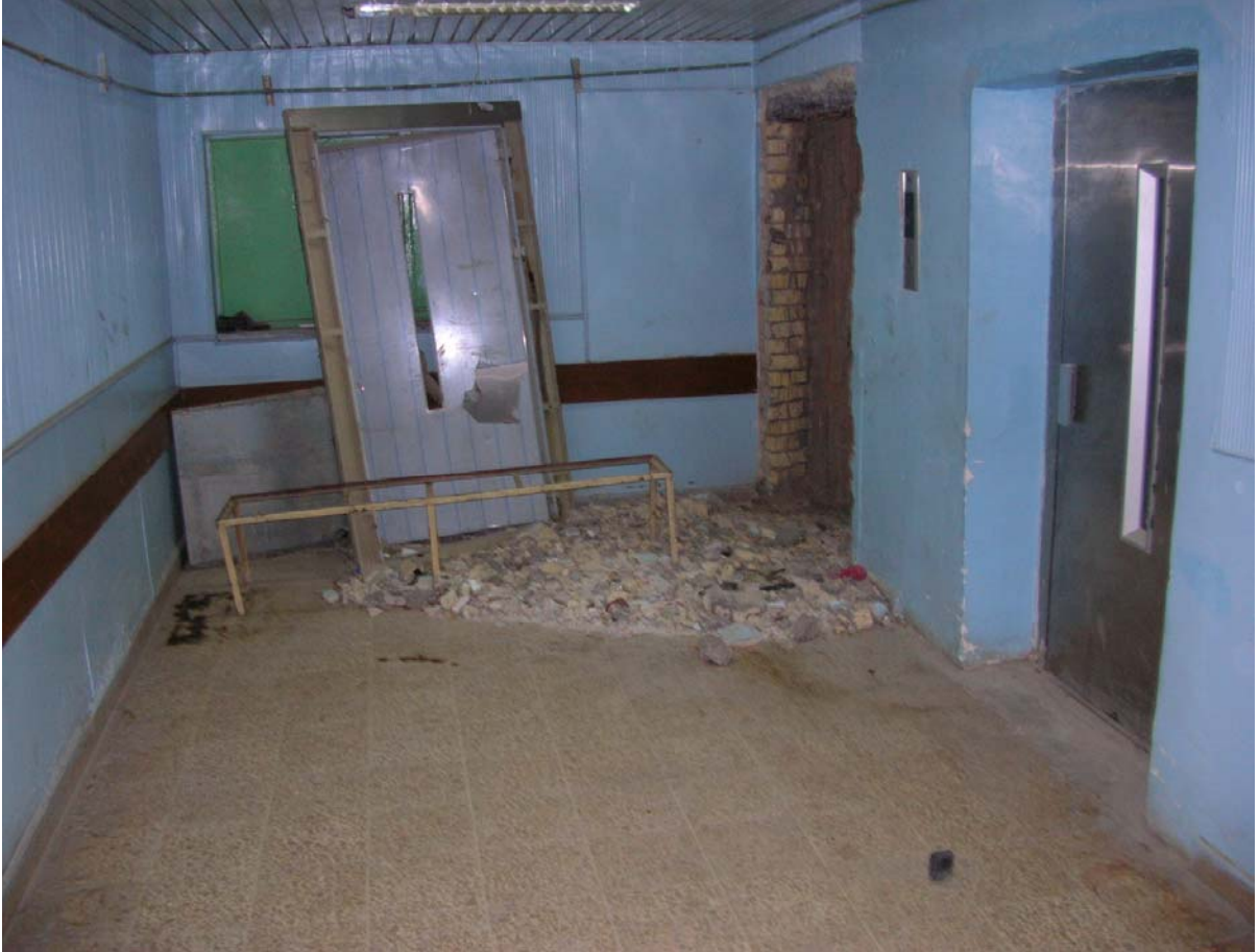
Photo 1. Al Hillah General Hospital Elevator
