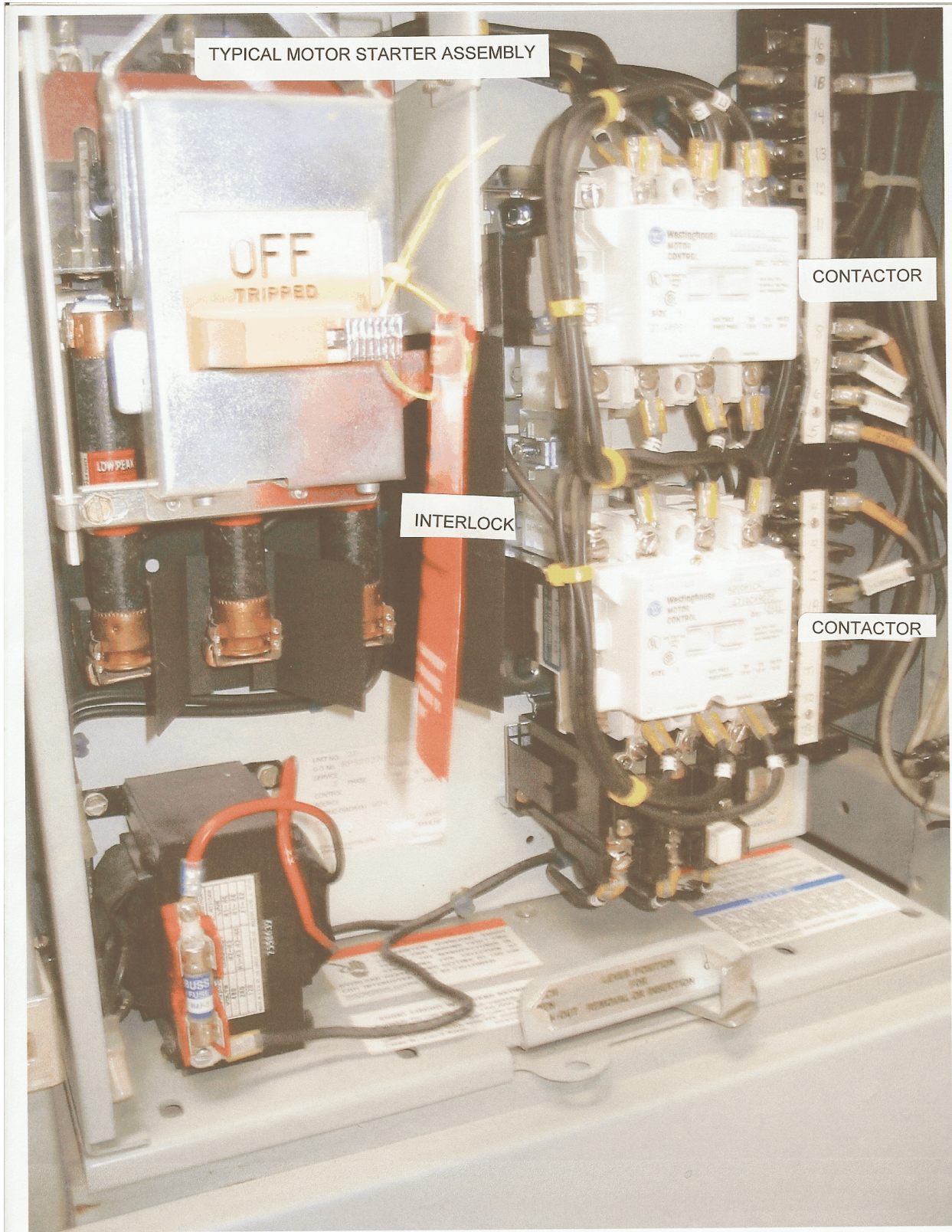
Figure 1: Typical Westinghouse Full Voltage, Reversing Starter Assembly, NEMA Class 1
