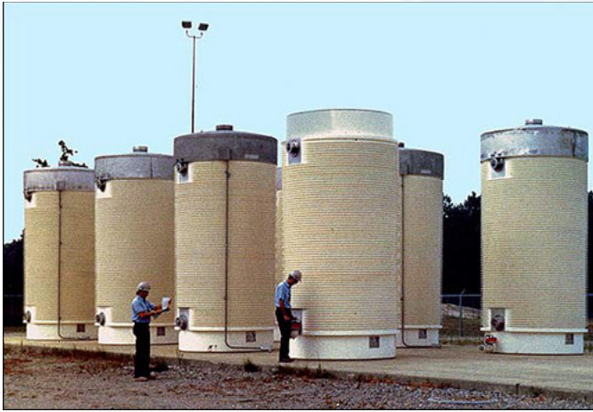
Spent Fuel Dry Cask Storage
