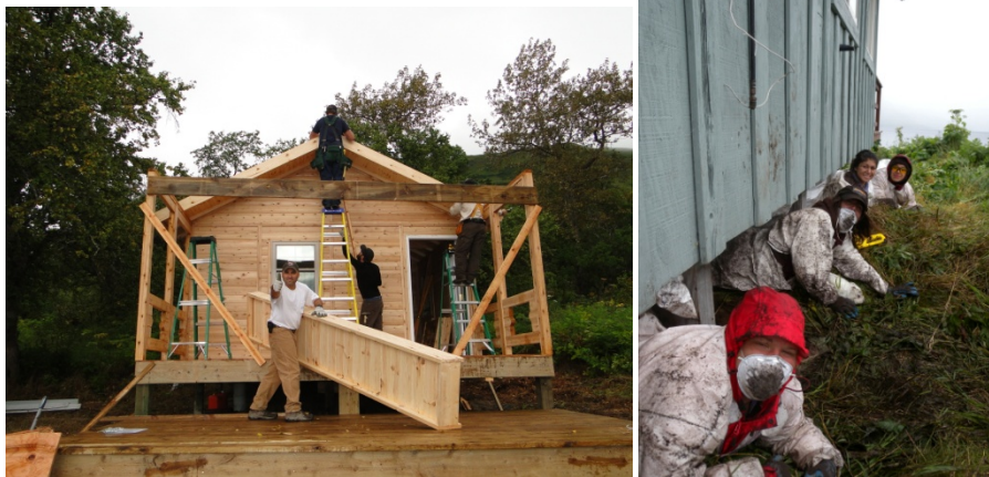
Volunteer crew working on the Uganik Island Cabin, and YCC crew working on weatherizing Deadman Cabin.
