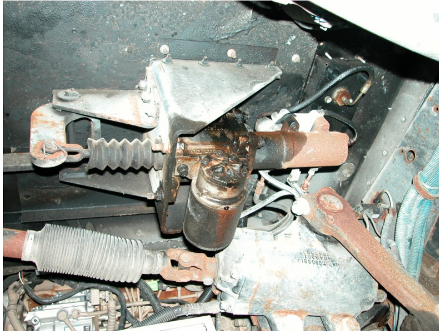
Figure 13. Master cylinder (center) in lead school bus, with hydraulic fluid seepage covering cylinder body.
