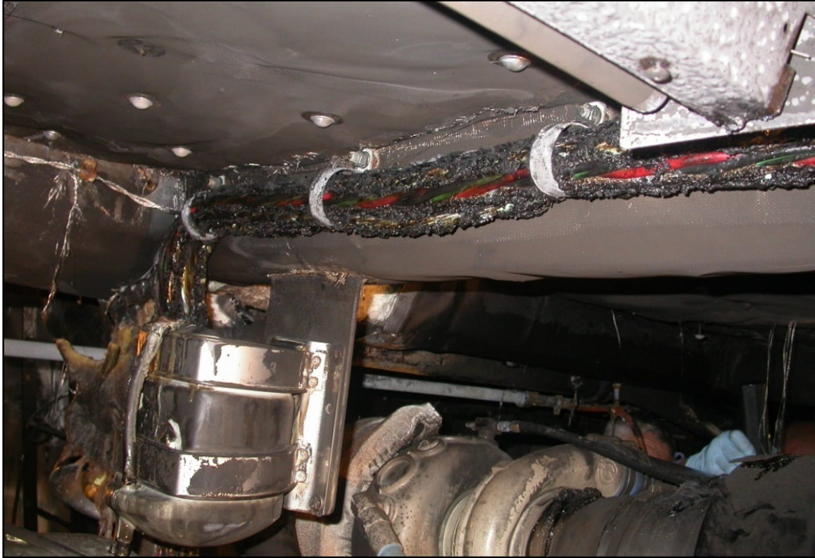
Figure 6. Damage to overhead wiring in engine room.
