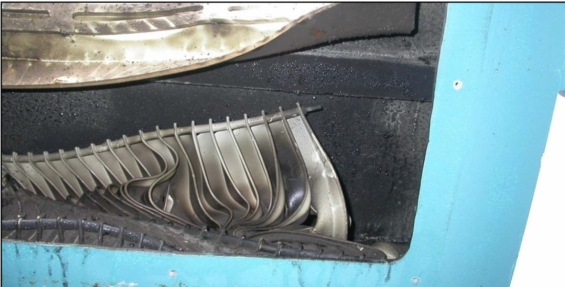
Figure 5. Closeup of damaged starboard vent cover (viewed from inside vent).
