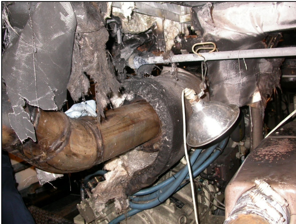
Figure 8. Charred lagging on port engine exhaust duct.
