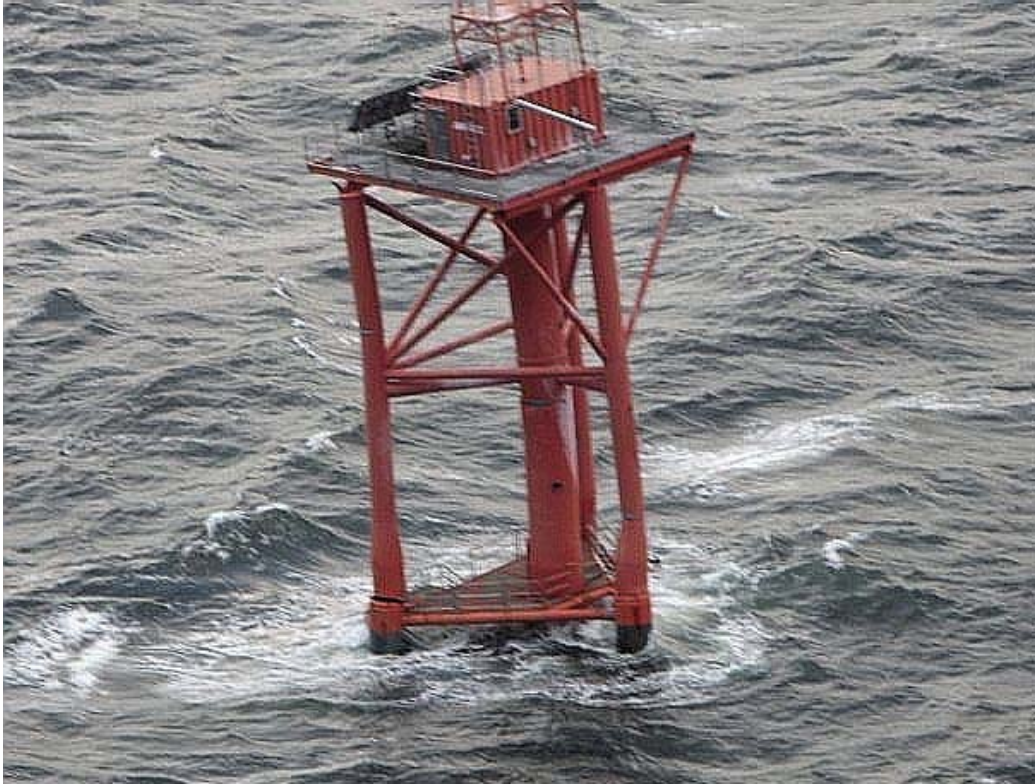
Figure 8. Ambrose Light, leaning after sustaining damage. Photo by the Coast Guard.
