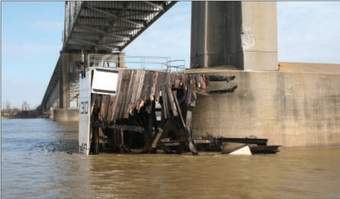
Figure 3. Damage to the I-10 bridge fender system and pier.
