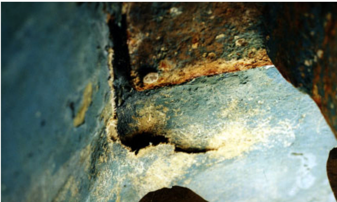
Figure 6b. Closeup of 2-inch opening in fracture around strut plate.
