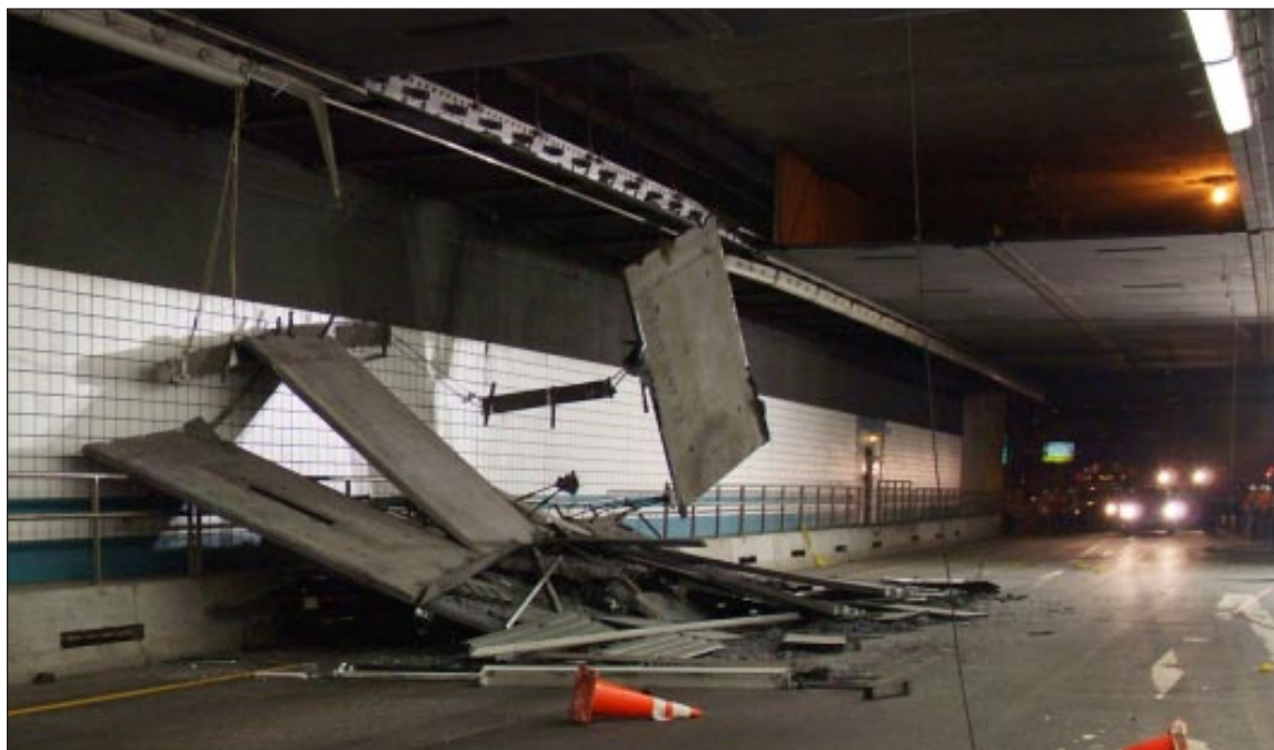
Figure 1. Postaccident scene with the crushed passenger car barely visible under the wreckage. The open area in the ceiling is the original location of the concrete panels. (Photograph courtesy Massachusetts State Police)
