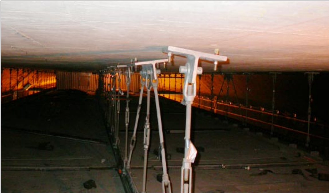
Figure 10. This photograph, taken in the westbound D Street portal tunnel after the accident, shows a number of roof hanger plates that have begun to pull away from the tunnel roof, including the two-anchor hanger plate in the foreground and the four-anchor plate adjacent to it.
