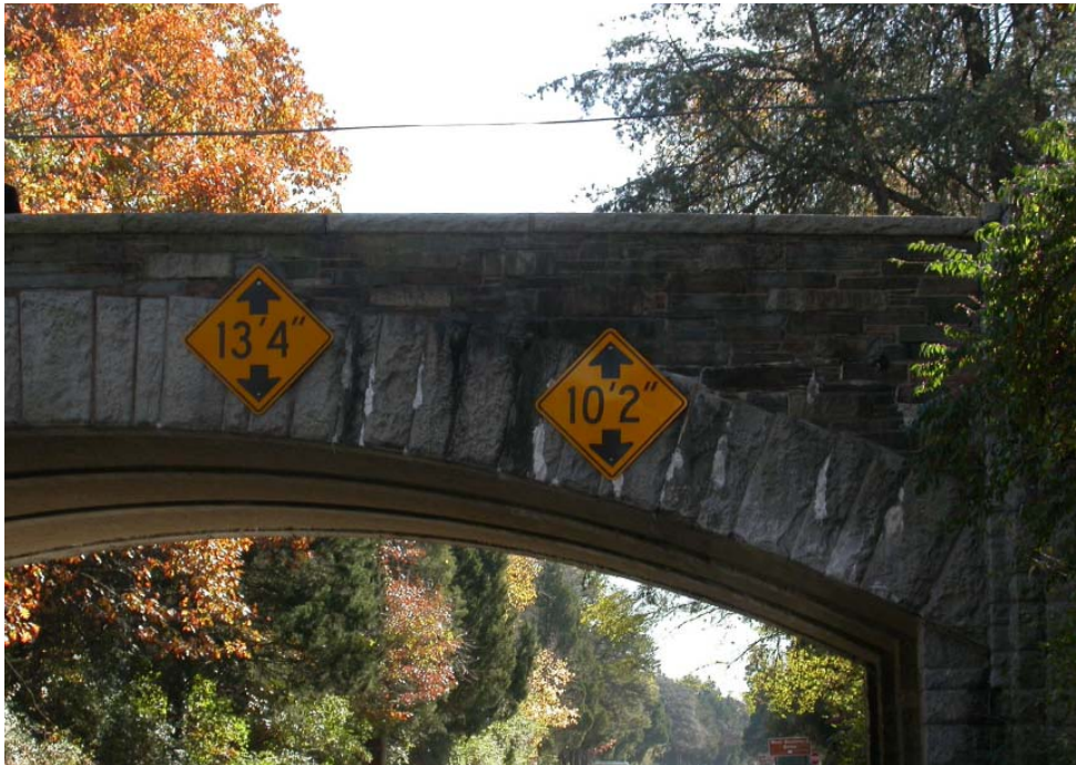
Figure 4. Mounted warning signs—Alexandria Avenue bridge clearance.
