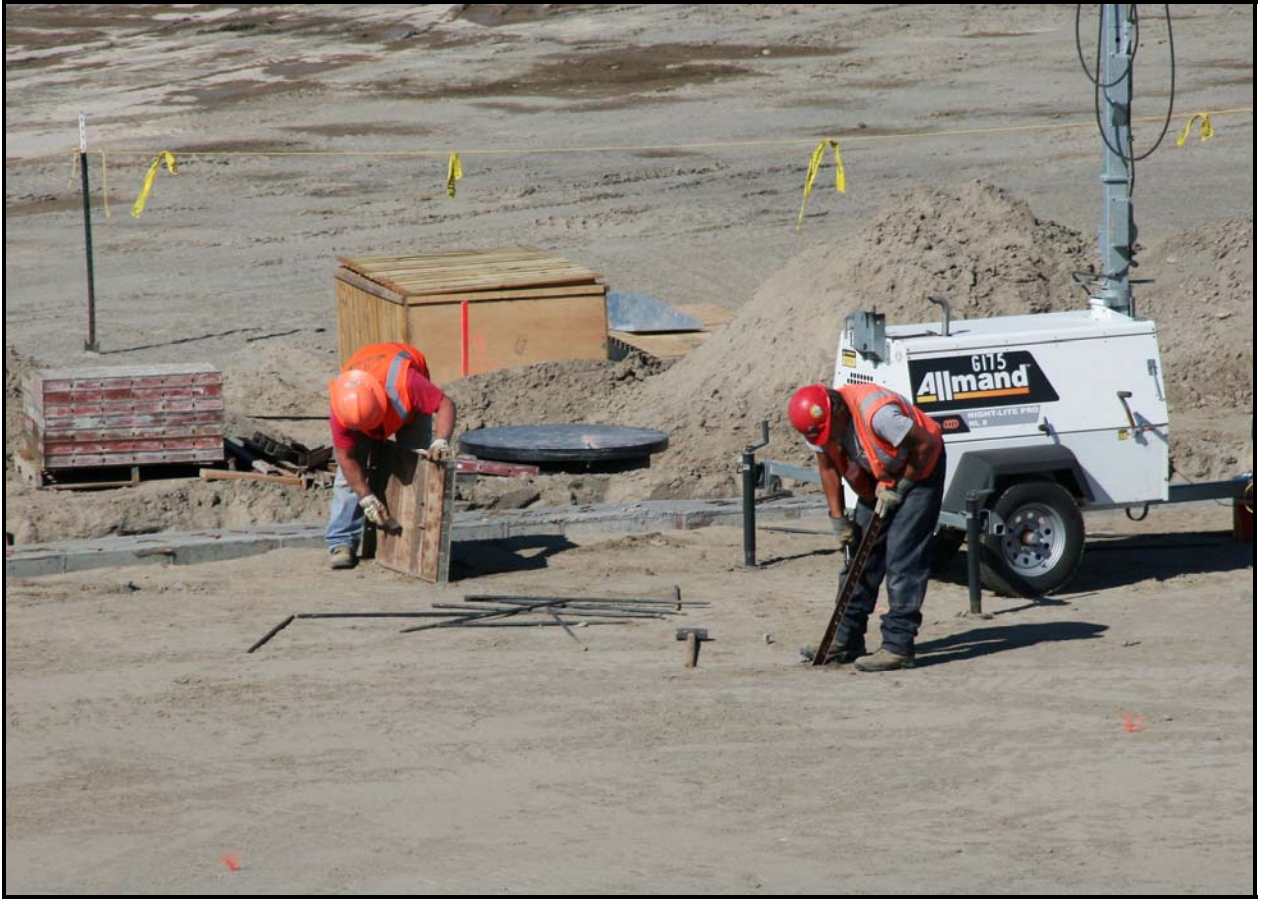
Workers remove the forms used to pour the foundation of leachate holding tank no. 4 at the Environmental Restoration Disposal Facility. (Photo 3)
