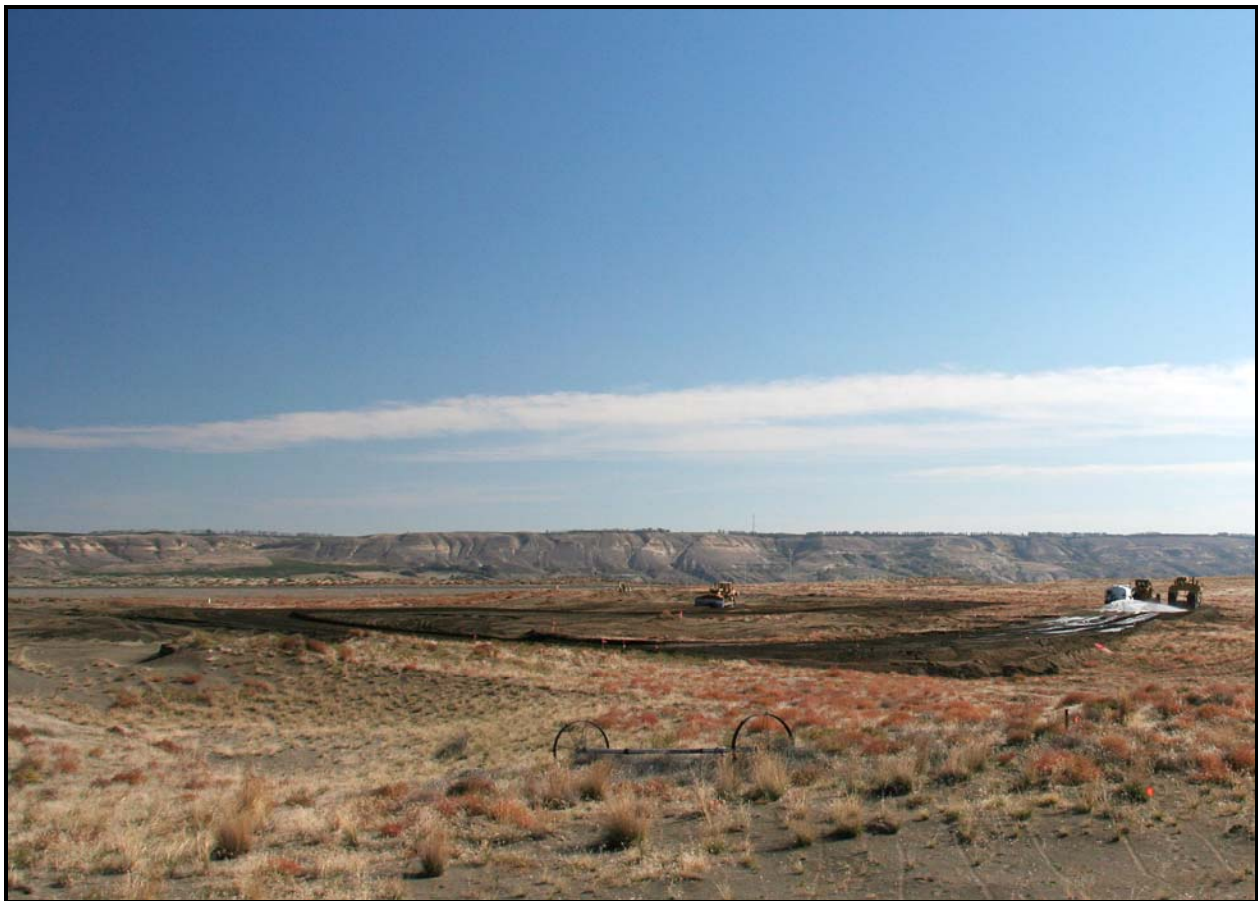
Washington Closure Hanford subcontractor White Shield/Apollo continues with earthwork activities at the 618-10 Burial Ground. (Photo 7)
