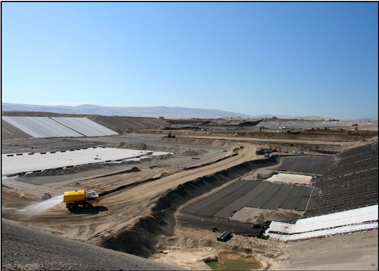
A view from the northwest corner of the super cell 10 shows liner construction progress at the Environmental Restoration Disposal Facility. (Photo 1)
