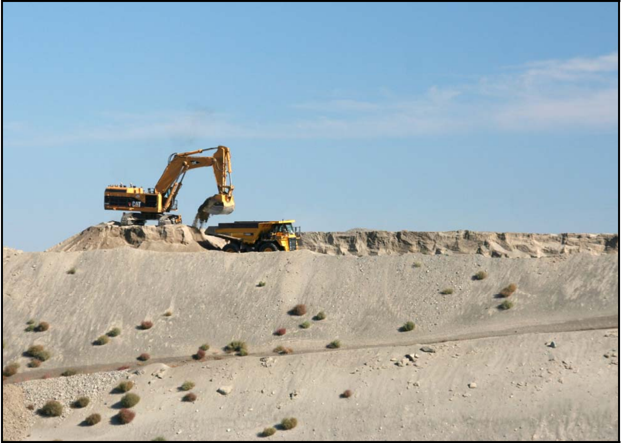
The soil used for the operations layer of super cell 9 is loaded for placement at the Environmental Restoration Disposal Facility. (Photo 2)
