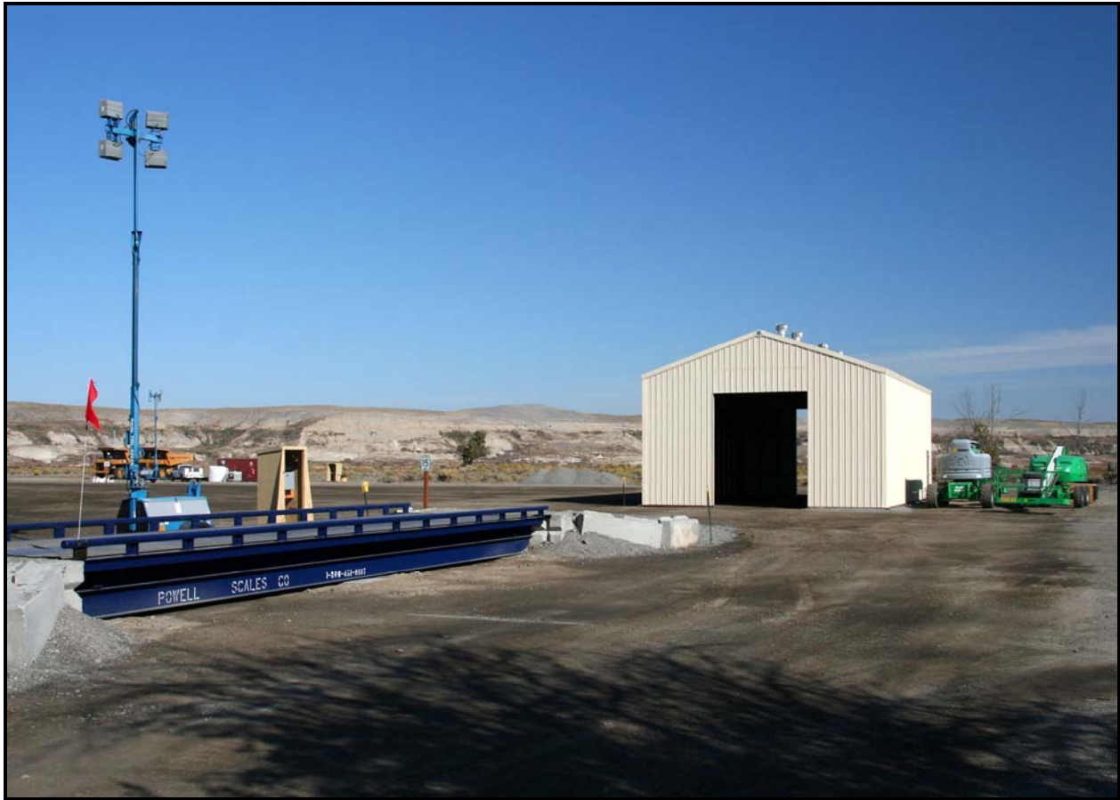
Work continues to construct the subcontractor survey structure at 100-F Area. (Photo 10)
