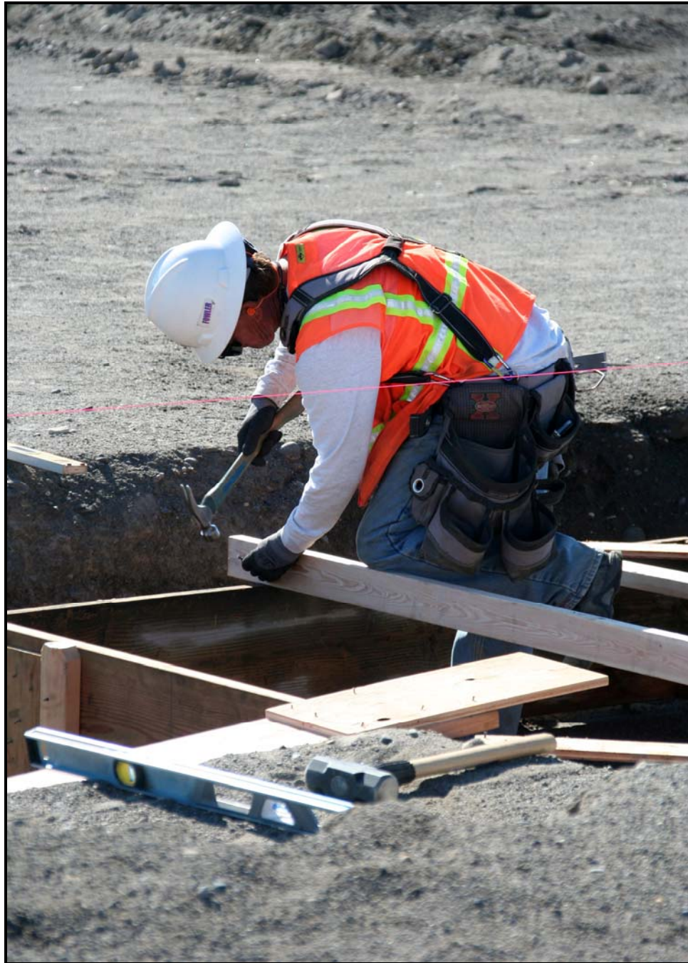
A worker installs forms for the footings at the equipment maintenance facility/operations center. (Photo 6)
