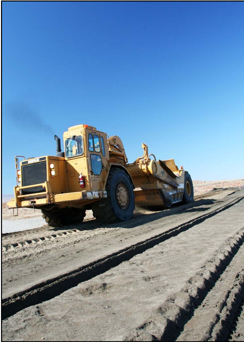
An earth scraper operates at the 618-10 Burial Ground. Work to construct a container transfer area and a trailer complex is under way. (Photo 8)
