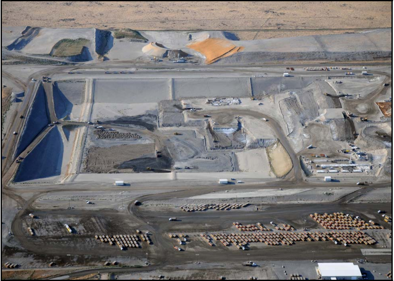
The construction of super cells 9 and 10 increased the Environmental Restoration Disposal Facility's capacity by 5.6 million tons. The facility, which contains 12 million tons of waste, has a capacity of 16.4 million tons. (Photo 1)
