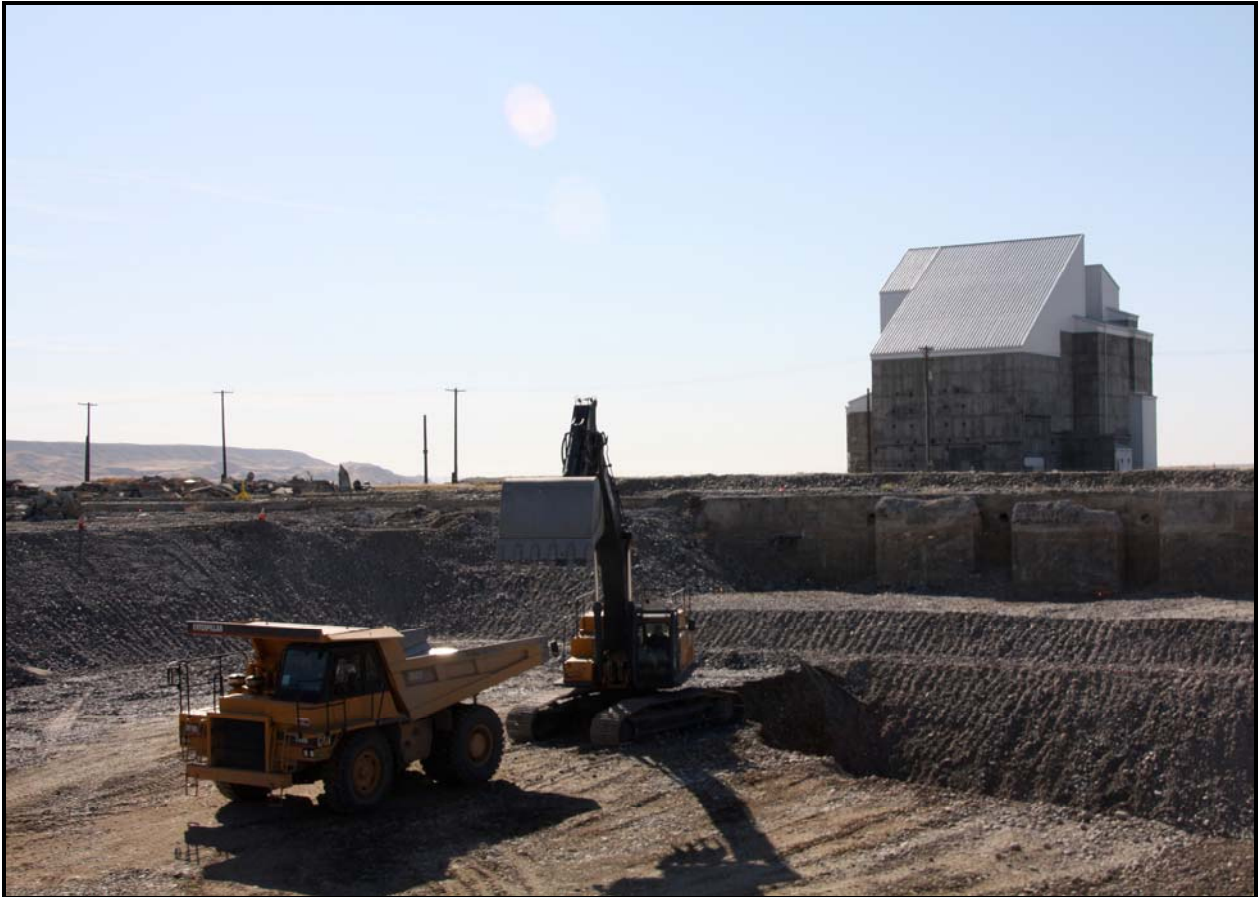
Washington Closure Hanford subcontractor Ojeda Business Ventures continues excavation and loadout activities at 100-F-57. (Photo 5)
