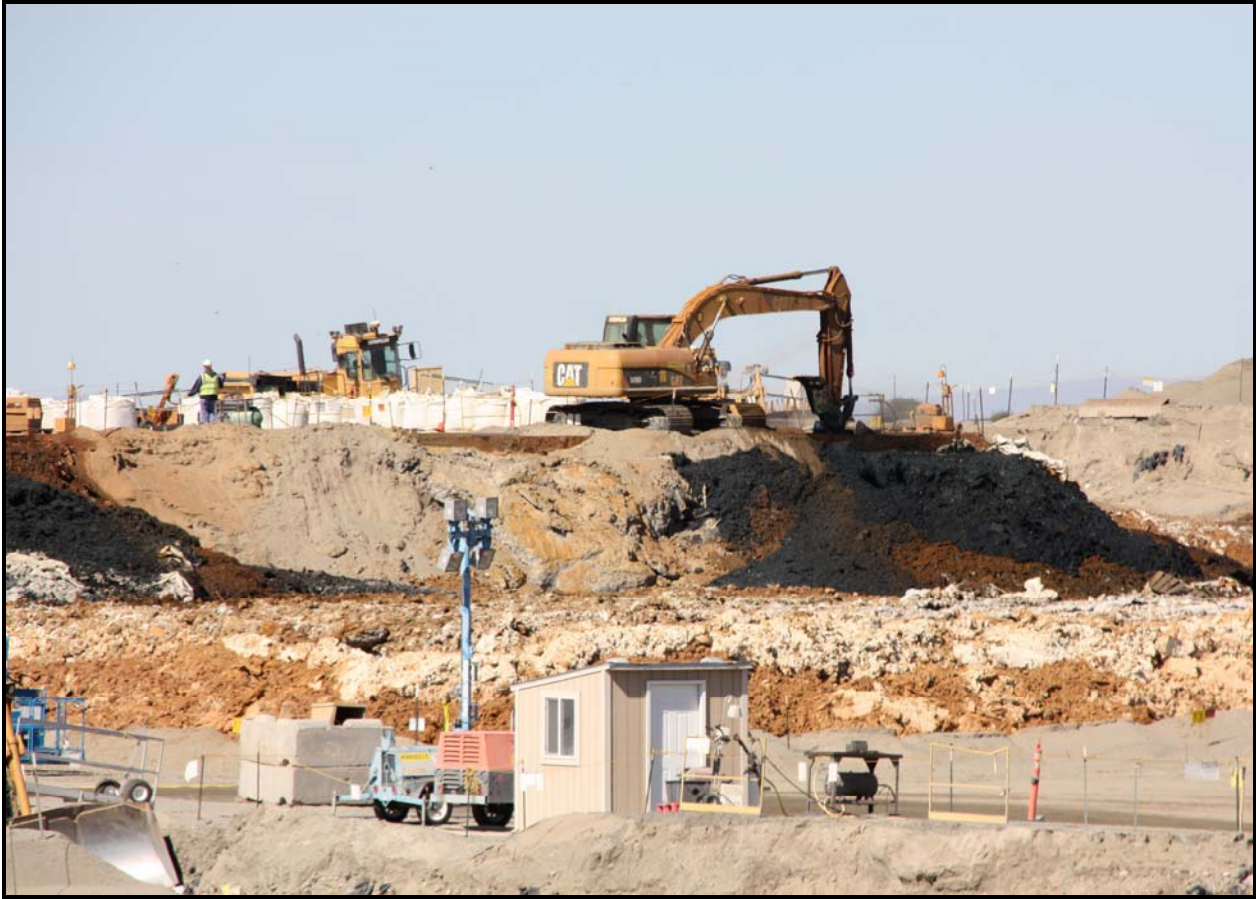
Washington Closure Hanford continues to treat chromium-contaminated waste at the Environmental Restoration Disposal Facility. (Photo 3)
