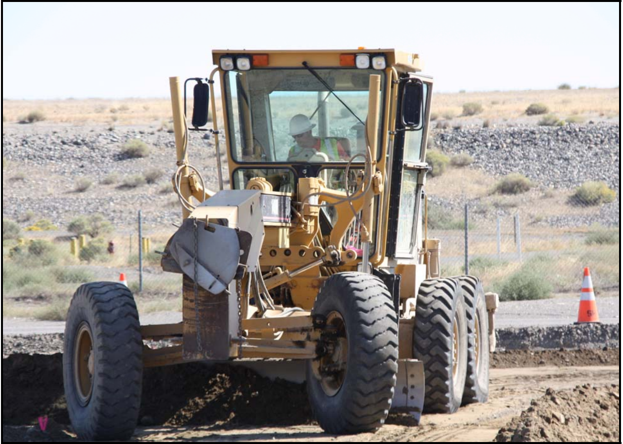
Washington Closure Hanford subcontractor Grant Construction continues road construction at the Environmental Restoration Disposal Facility. (Photo 4)
