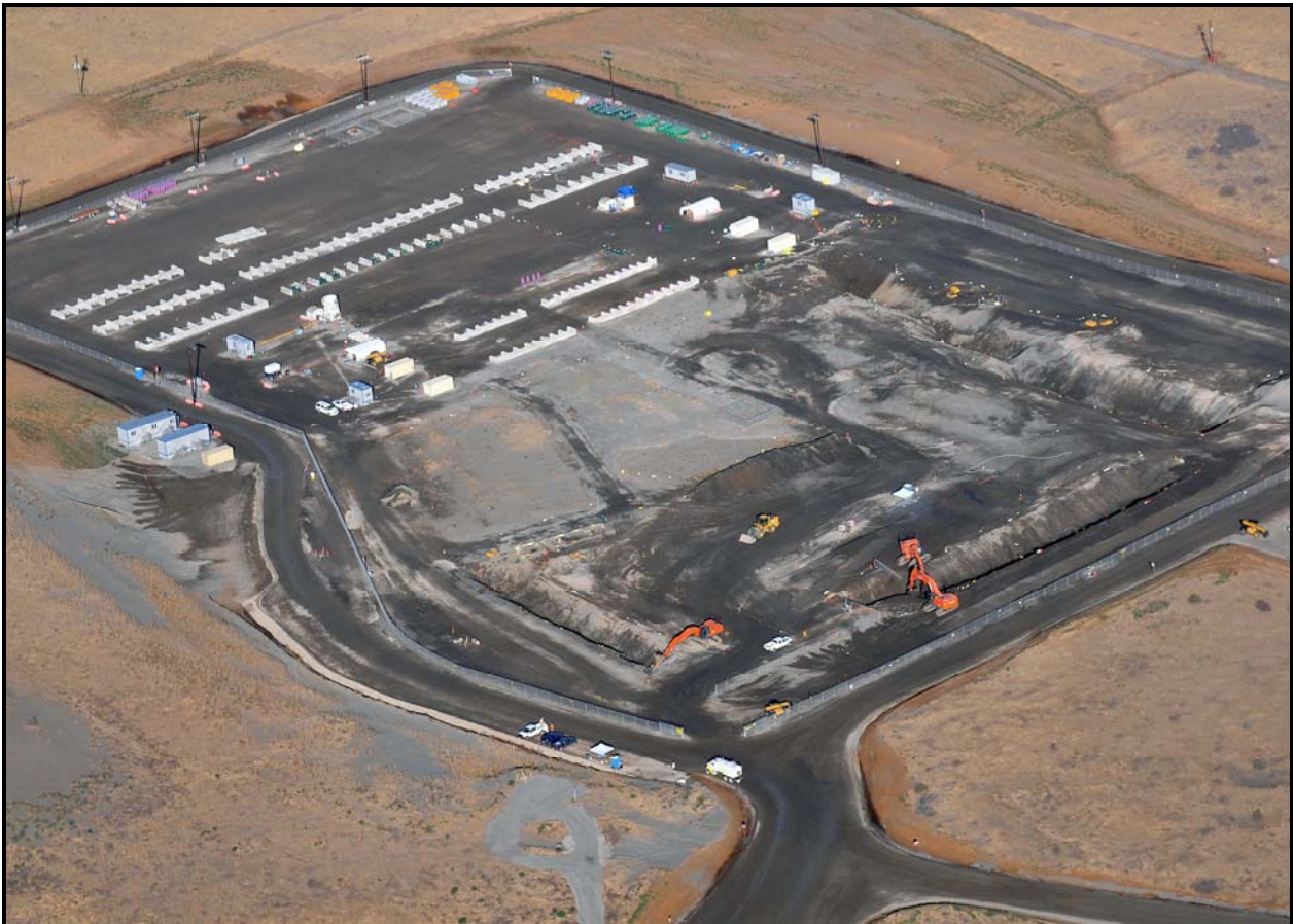
Washington Closure Hanford continues with excavation of waste trenches at the 618-10 Burial Ground, which is one of the most hazardous sites at Hanford. (Photo 4)
