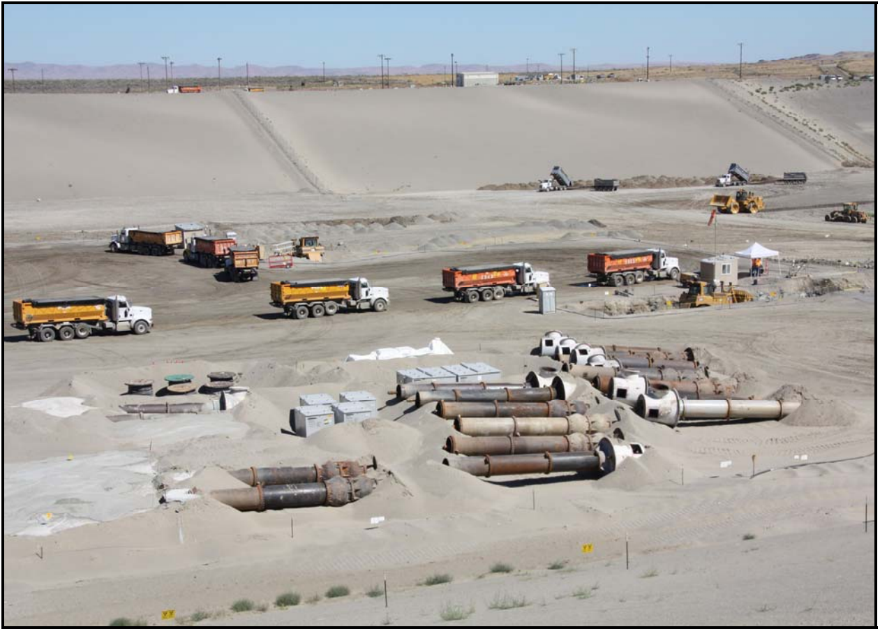
Trucks prepare to dispose of waste off a recently constructed dump ramp at the Environmental Restoration Disposal Facility. The waste is being spread into super cell 10. Pumps from the water intake structures from K reactors are being disposed in the foreground. (Photo 2)
