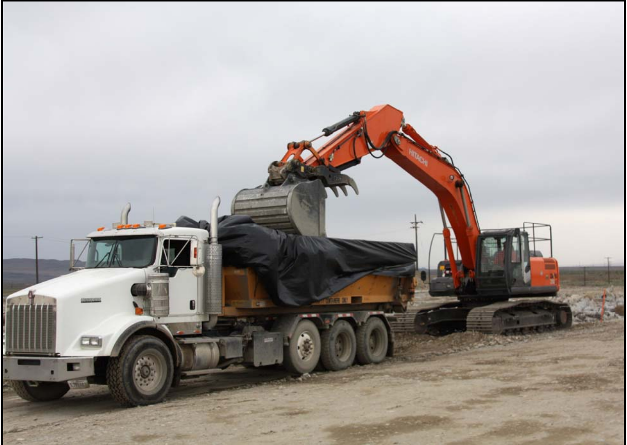
Washington Closure Hanford subcontractor Ojeda Business Ventures loads out rubble from 100-F-57. (Photo 11)
