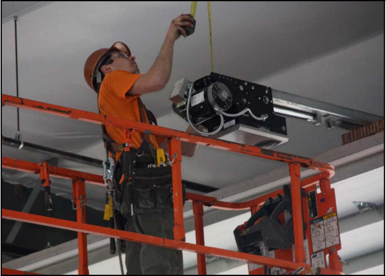
An ELRFowler employee installs a garage door opener in ERDF's new equipment maintenance facility/operations center. (Photo 4)
