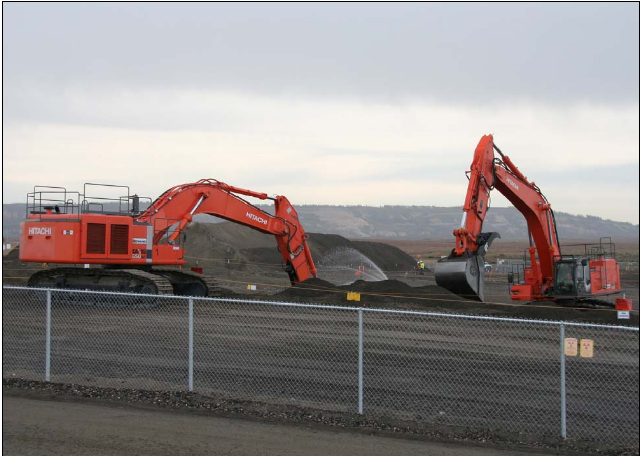
Washington Closure Hanford continues trench excavation on the north side of the burial ground. (Photo 6)
