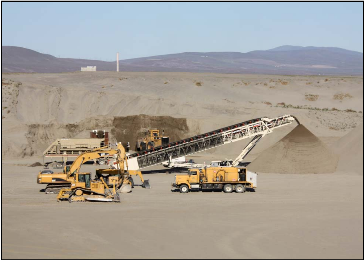
Washington Closure Hanford subcontractor DelHur Industries tests a soil screen plant set up in support of ERDF's new batch plant. (Photo 5)
