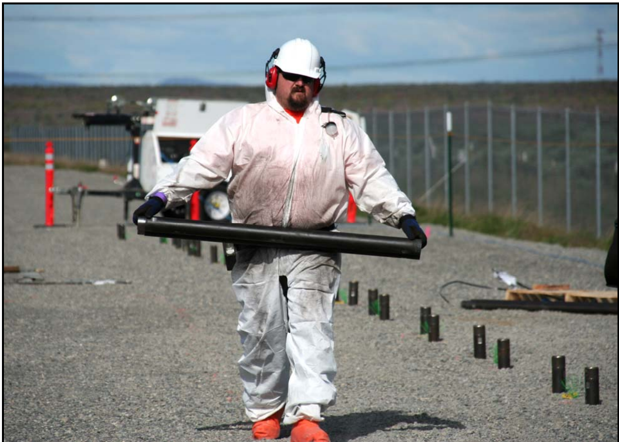
Washington Closure Hanford subcontractor North Wind installing cone penetrometers at the 618-11 Burial Ground. (Photo 8)
