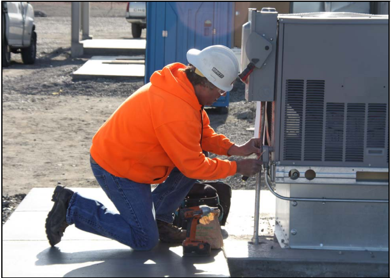
An employee with Sun River Electric Service works on an air conditioning unit at ERDF's new equipment maintenance facility/operations center. (Photo 3)
