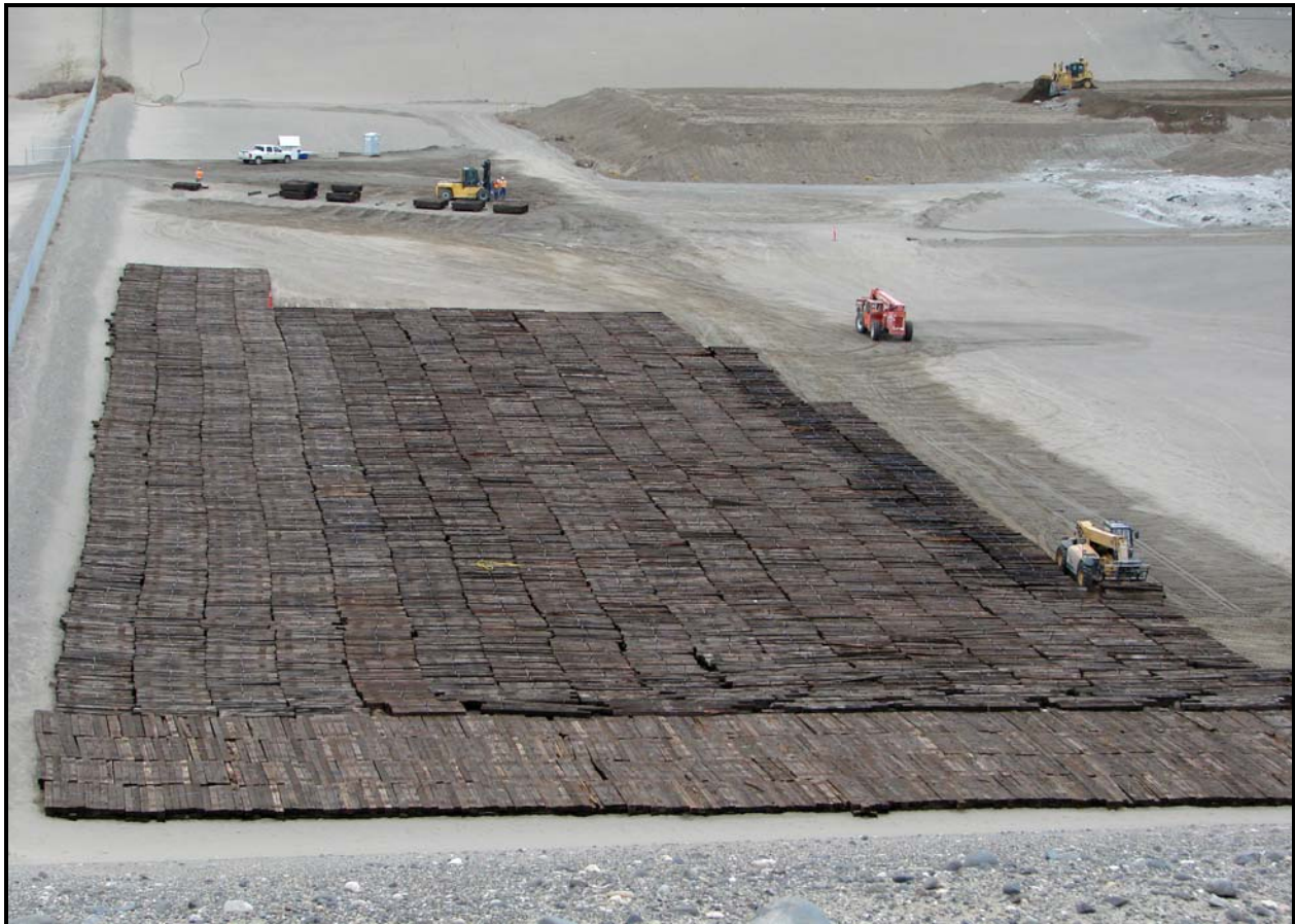
About 65,000 railroad ties from the Hanford Site are being disposed in super cell 9 at the Environmental Restoration Disposal Facility. (Photo 1)
