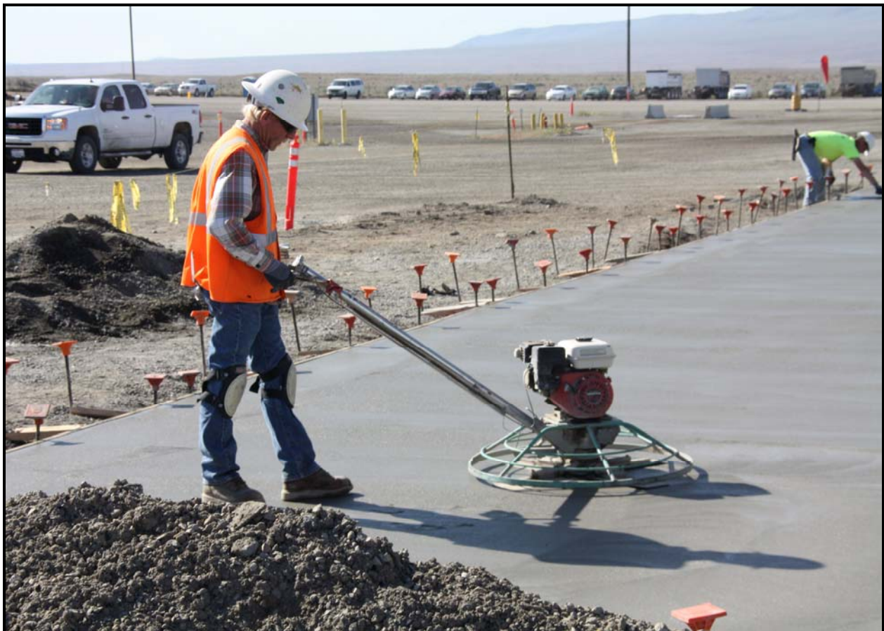
An ELRFowler employee uses a power trowel on recently poured concrete at the east side of ERDF's transportation maintenance facility. (Photo 2)
