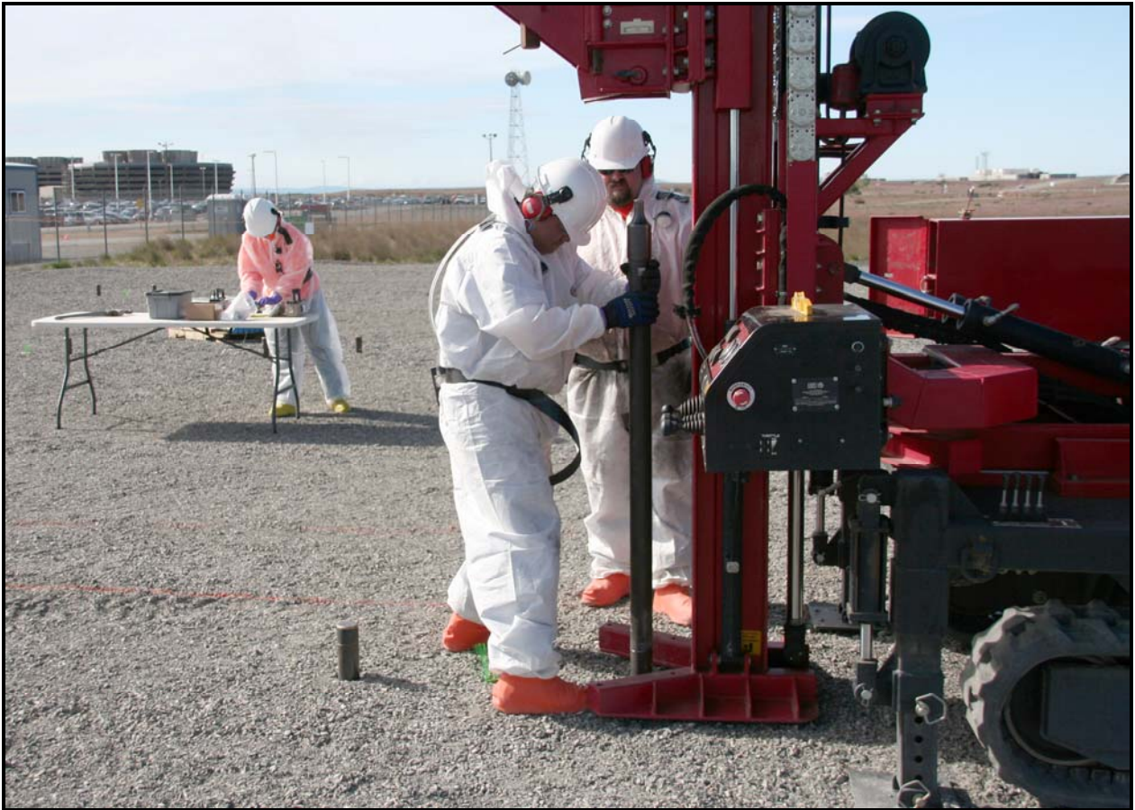
The cone penetrometers are narrow steel tubes that will house instrumentation to identify the location of radioactive materials within the vertical pipe units at the 618-11 Burial Ground. (Photo 10)
