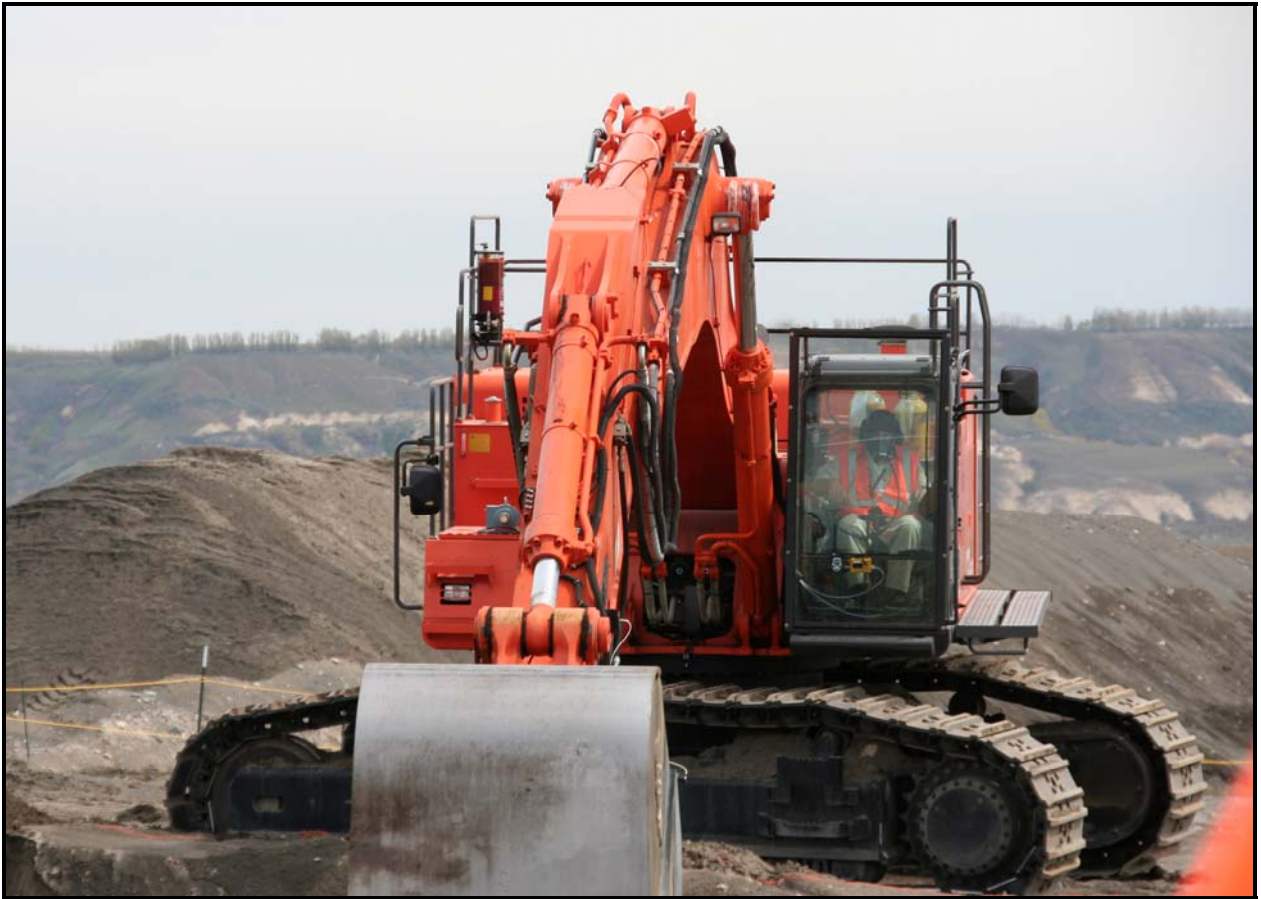
Excavation of the 618-10 Burial Ground is scheduled to be completed in April 2012. (Photo 5)
