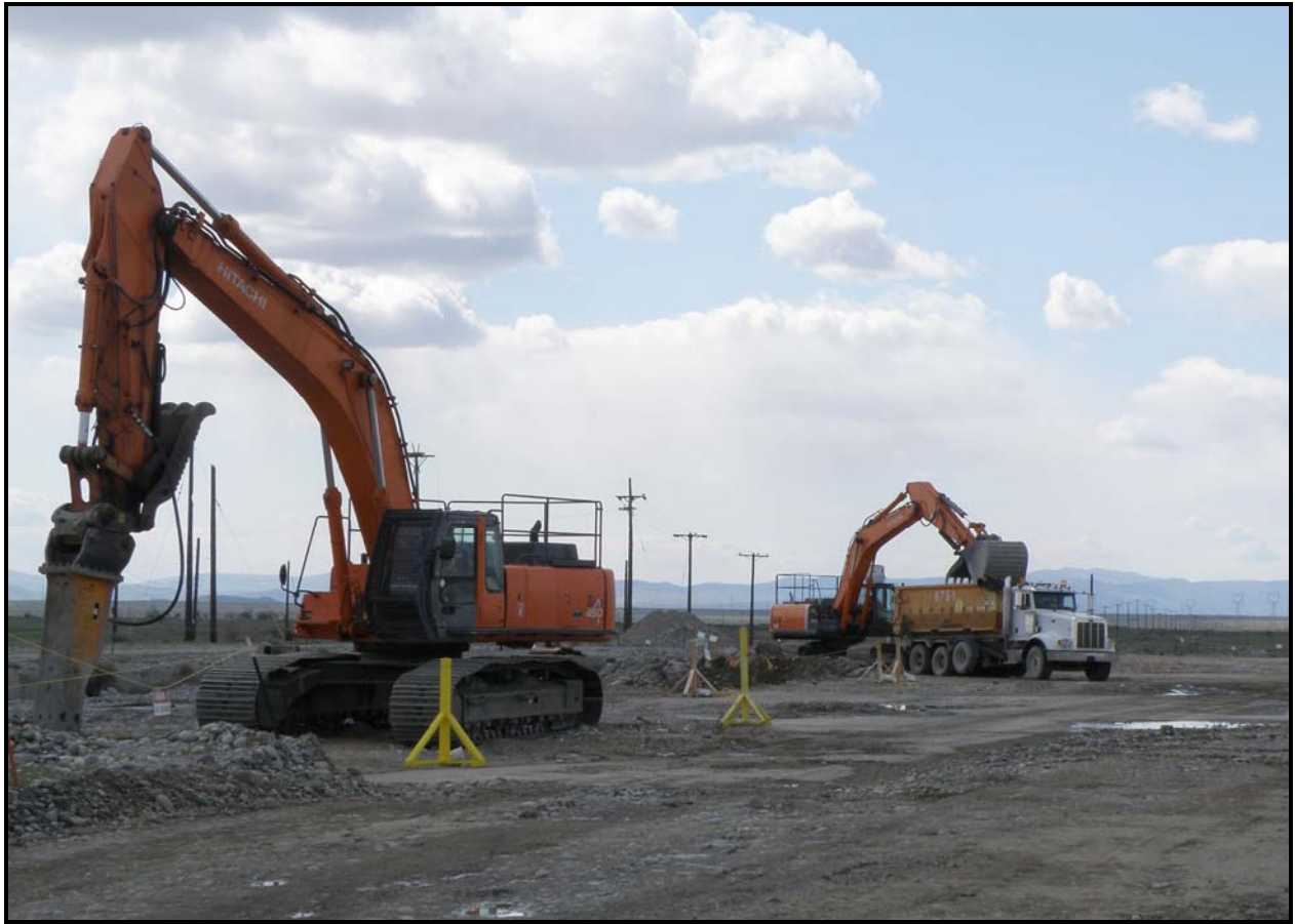
Concrete demolition and loadout of concrete and soil continues at 100-F-57. (Photo 10)
