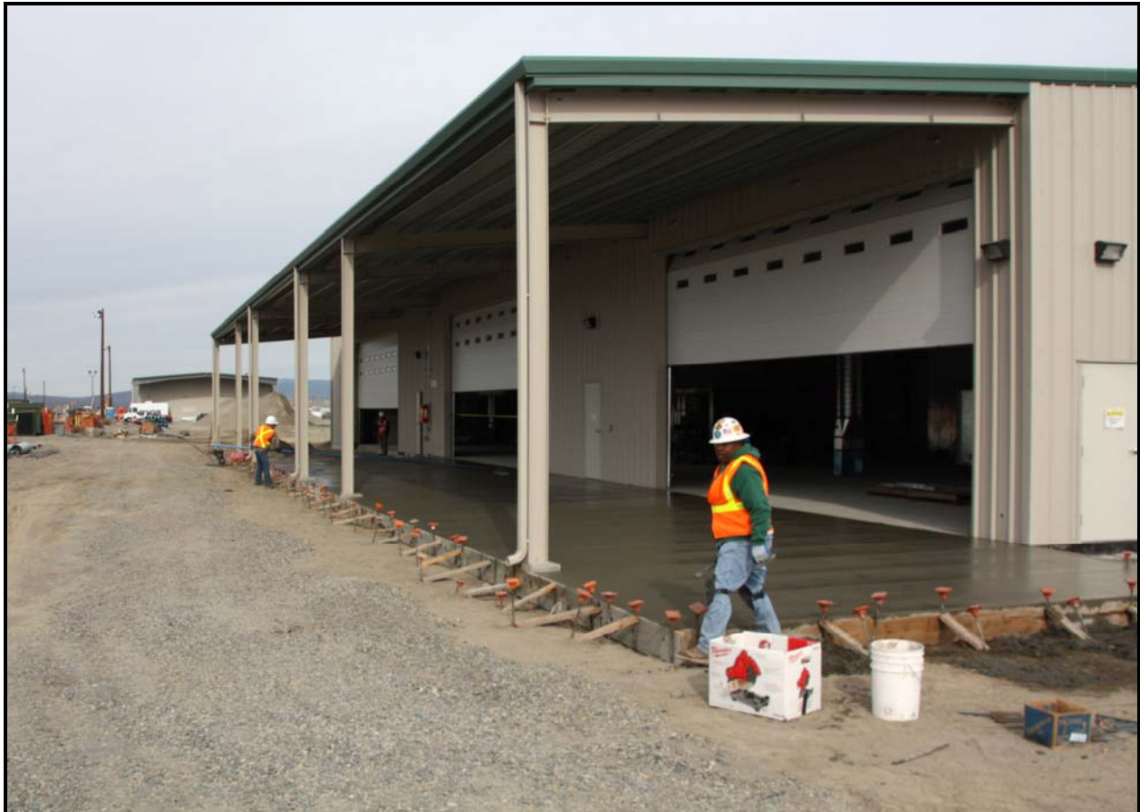
ELRFowler poured the concrete slab outside the front of ERDF's container maintenance facility. (Photo 2)
