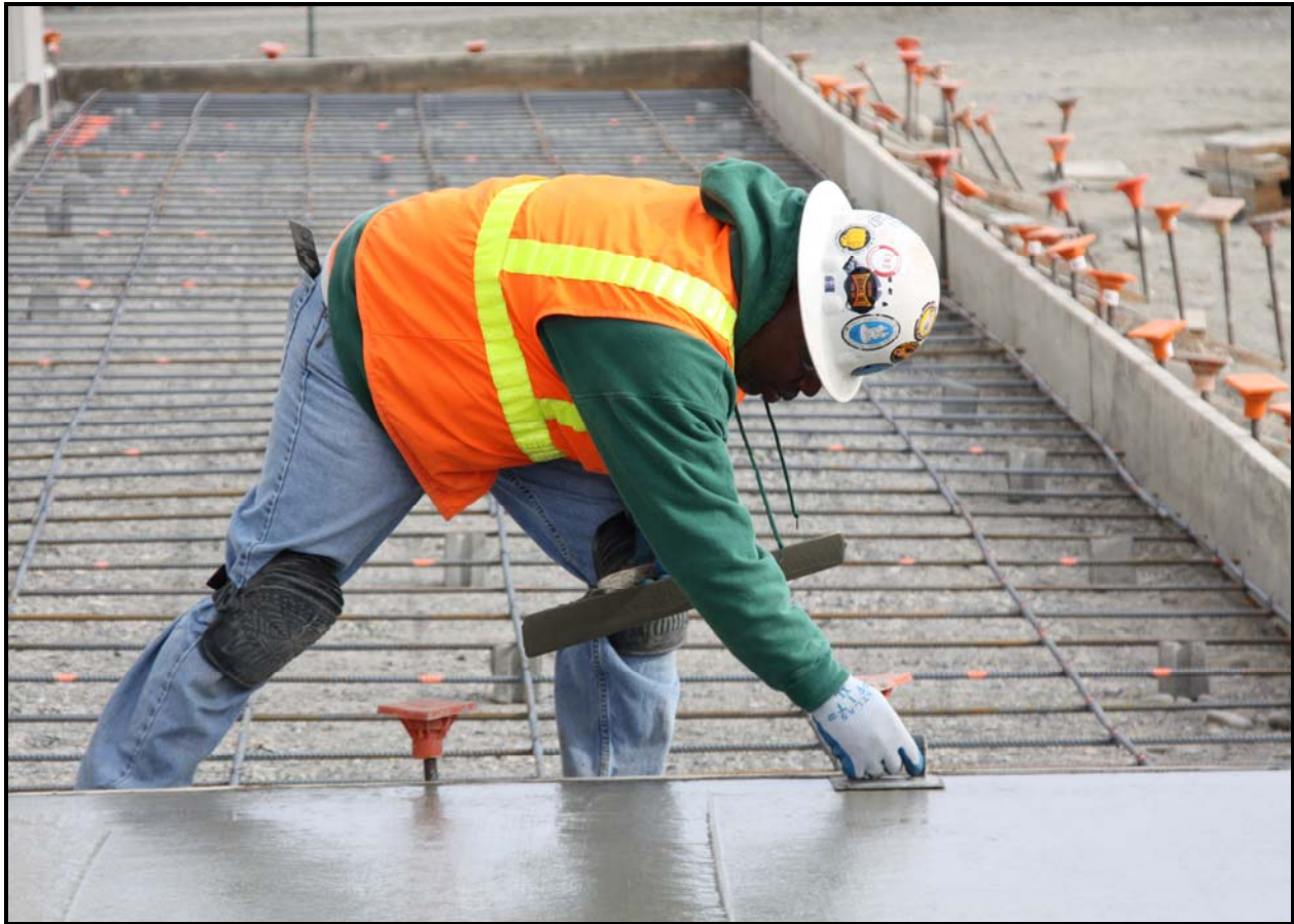
An ELRFowler employee edges the recently poured concrete slab at ERDF's container maintenance facility. (Photo 3)
