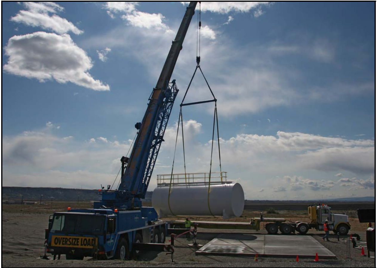
Washington Closure Hanford subcontractor Lampson International moves the first of three water tanks into place at the 618-10 Burial Ground. The tanks are used for dust suppression. (Photo 7)
