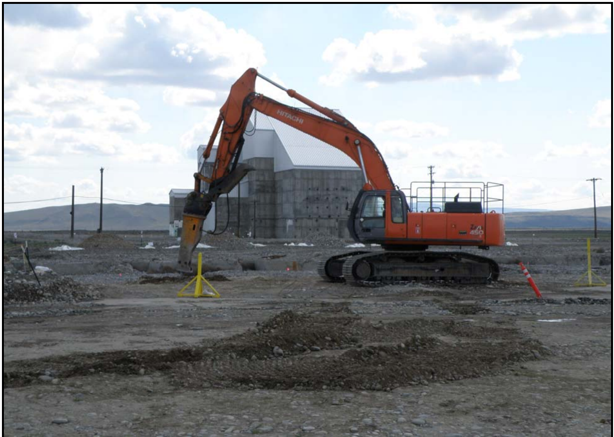
Washington Closure Hanford subcontractor Ojeda Business Ventures continues to break concrete at 100-F-57. The site contains hexavalent chromium. (Photo 9)
