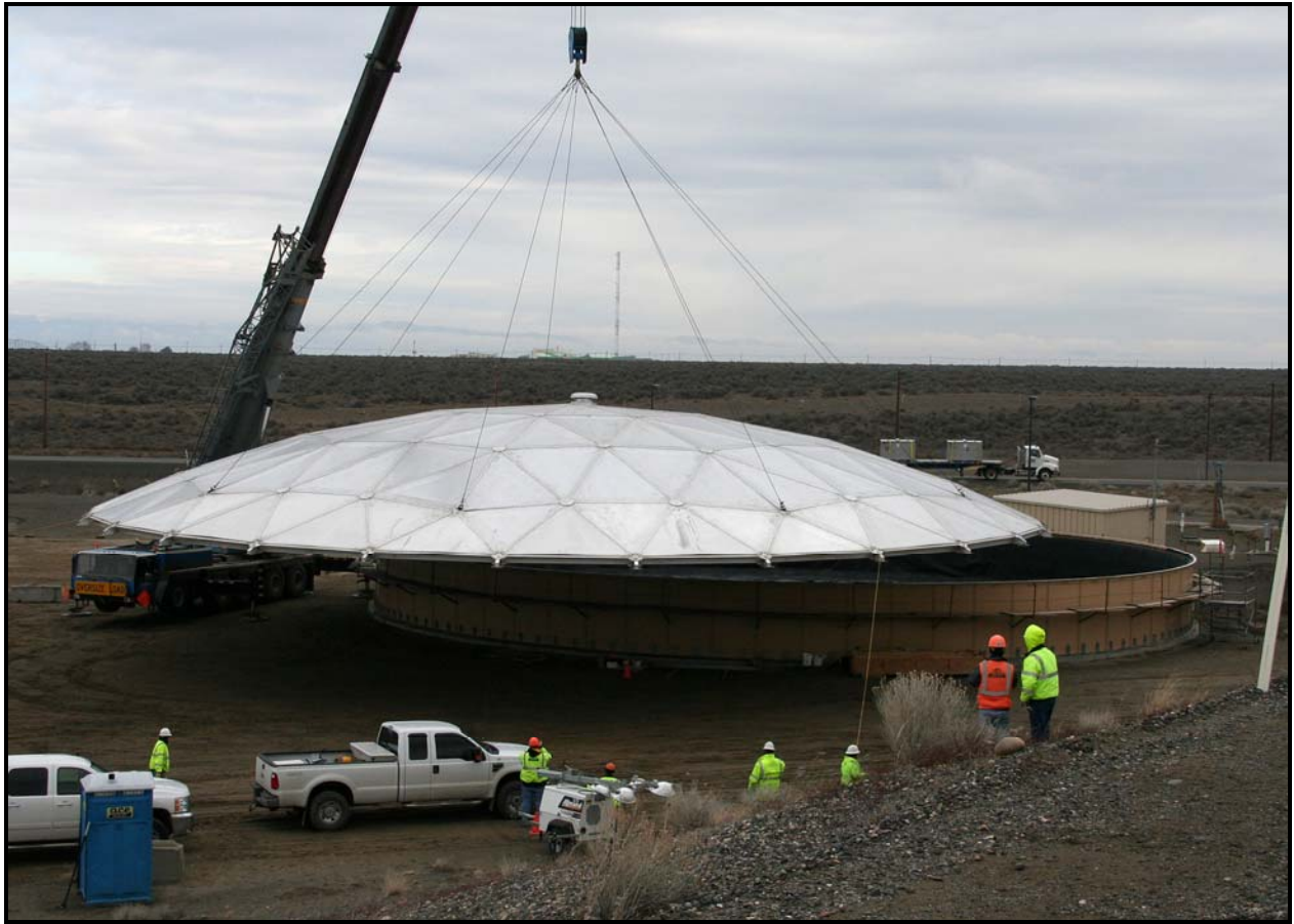
The 27,400-pound dome cover is placed on Leachate Storage Tank No. 4 at the Environmental Restoration Disposal Facility. (Photo 3)
