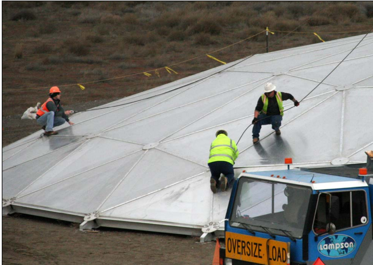
Workers from Lampson International prepare to raise the dome cover for Leachate Storage Tank No. 4 at the Environmental Restoration Disposal Facility. (Photo 1)
