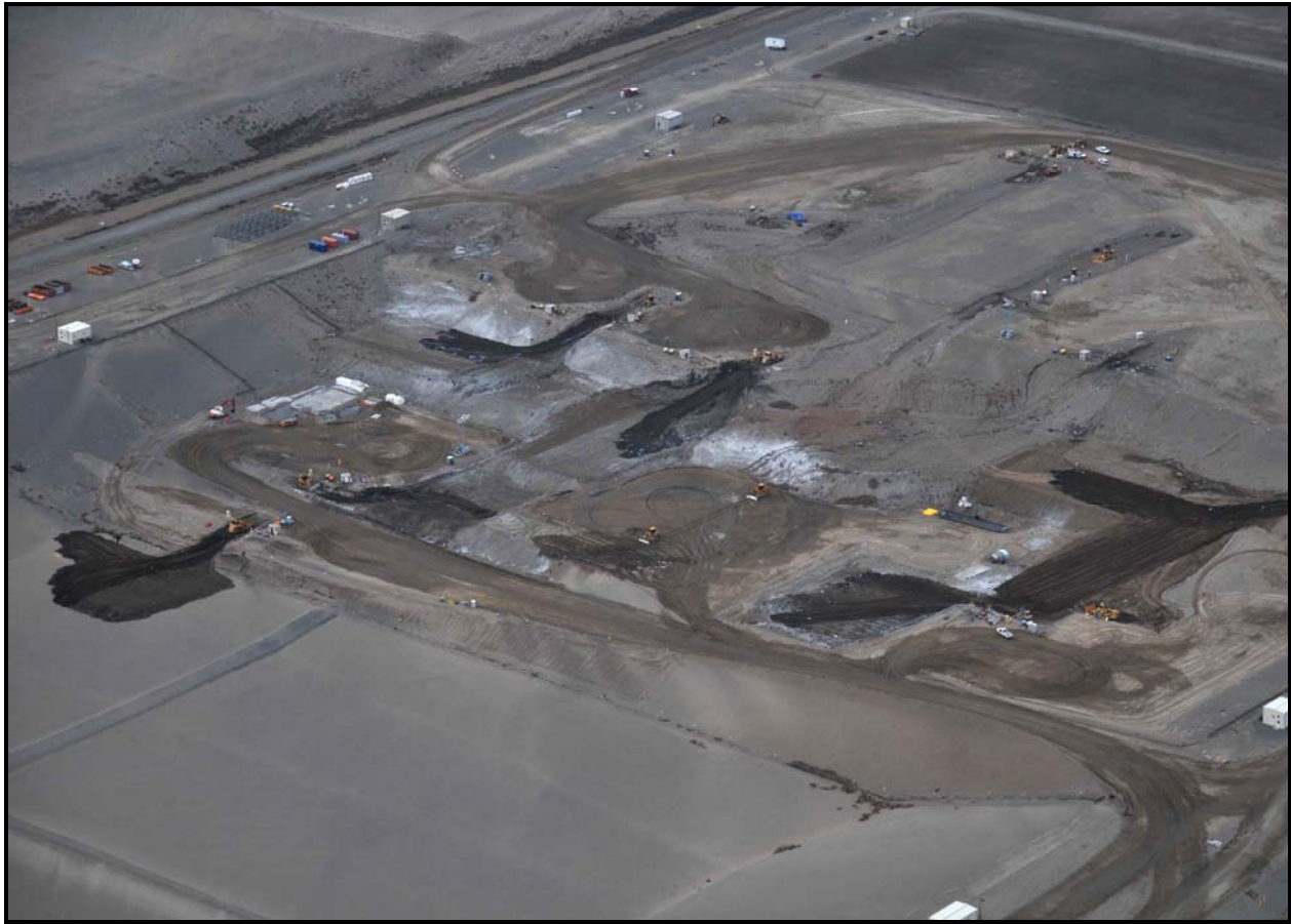
This aerial photo taken in mid-February shows waste being introduced into super cell 9 (lower left) at the Environmental Restoration Disposal Facility. (Photo 4)
