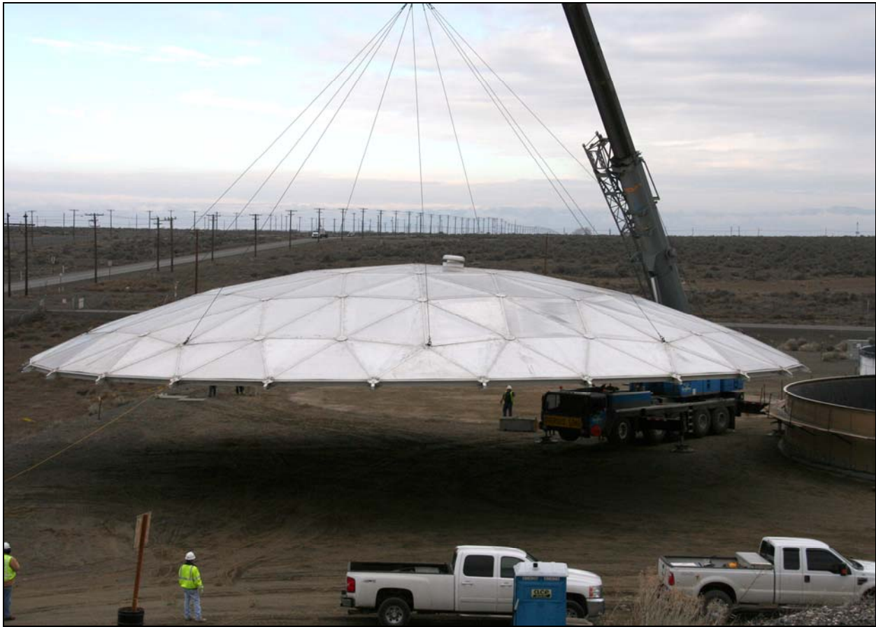
The dome covers for the new leachate storage tanks were constructed by Darrell Thompson Tanks & Construction of Bakersfield, California. (Photo 2)
