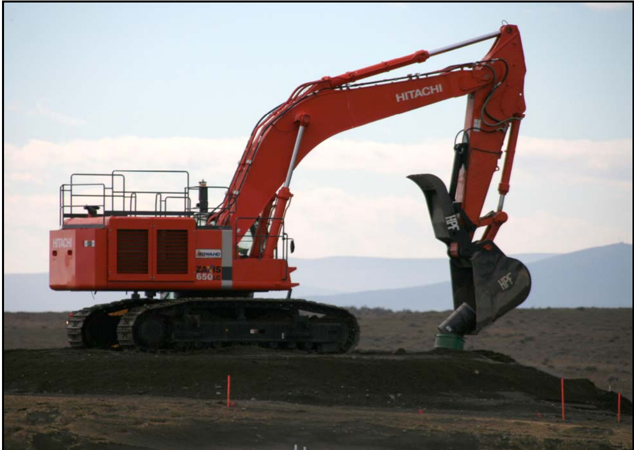
An excavator carefully places a drum inside a salvage container during mock-up exercises at the 618-10 Burial Ground. (Photo 5)
