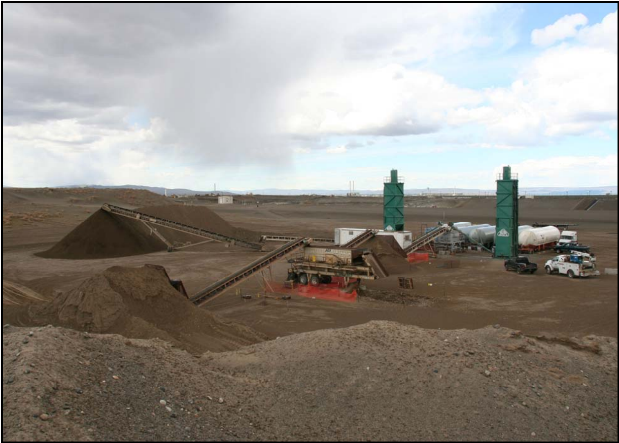
The pug mill manufactures the soil/bentonite admix material that will be used in the liner system of super cell 9 at the Environmental Restoration Disposal Facility.
