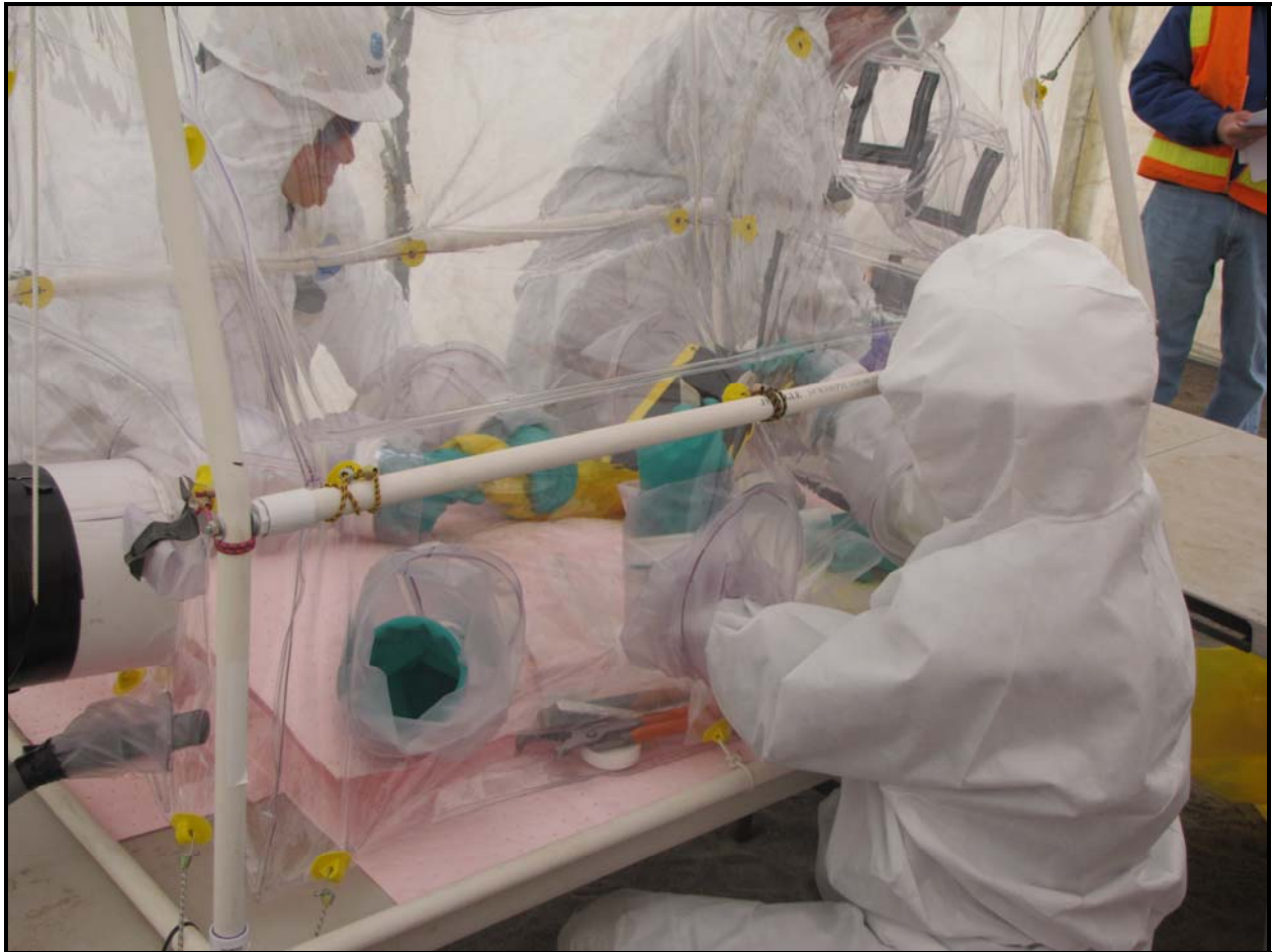
Handling and processing of soil samples collected at the 618-10 Burial Ground will be performed inside a table-mounted glove bag.
