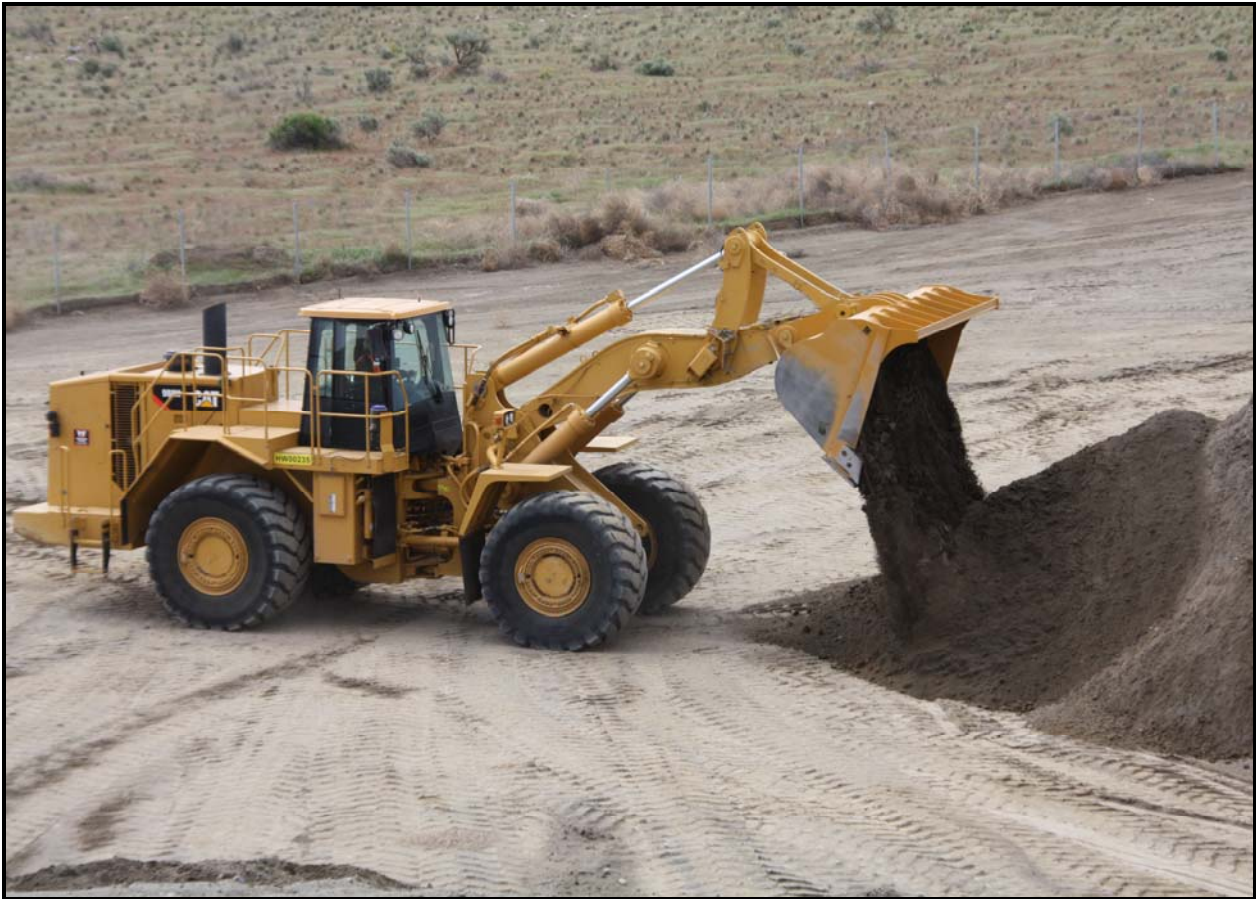
A new front-end loader was placed in operation at the Environmental Restoration Disposal Facility.
