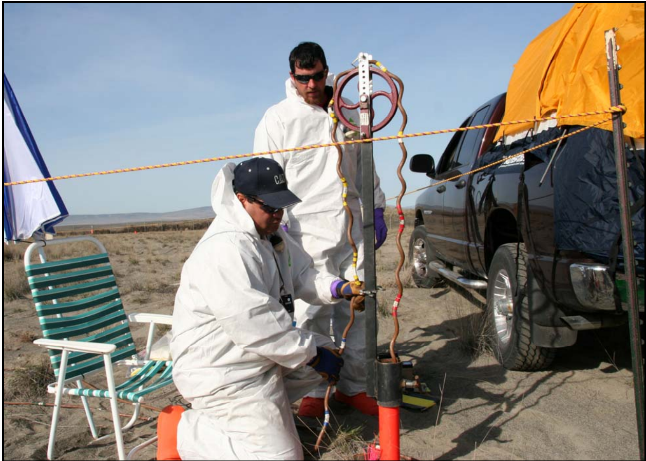
Nonintrusive characterization continues at the 618-10 Burial Ground. A multi-detector probe (MDP) is used to measure radiation sources near the vertical pipe units.
