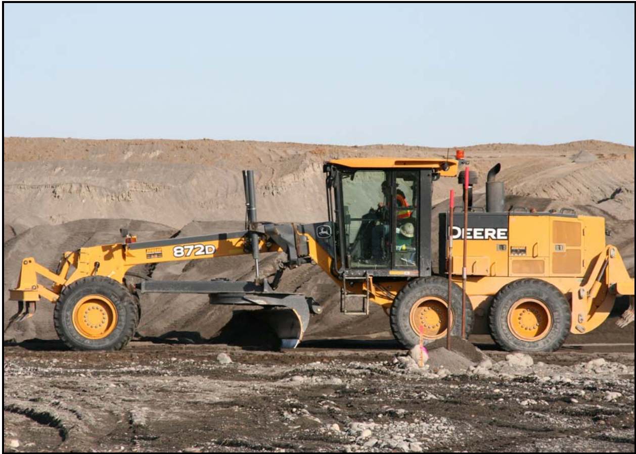
Road construction continues at the 618-10 Burial Ground. Crews are also constructing a drum processing area and a firebreak.
