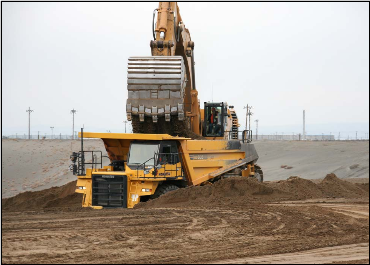
TradeWind Services and its subcontractor, DelHur Industries began excavation of super cell 10 at the Environmental Restoration Disposal Facility.
