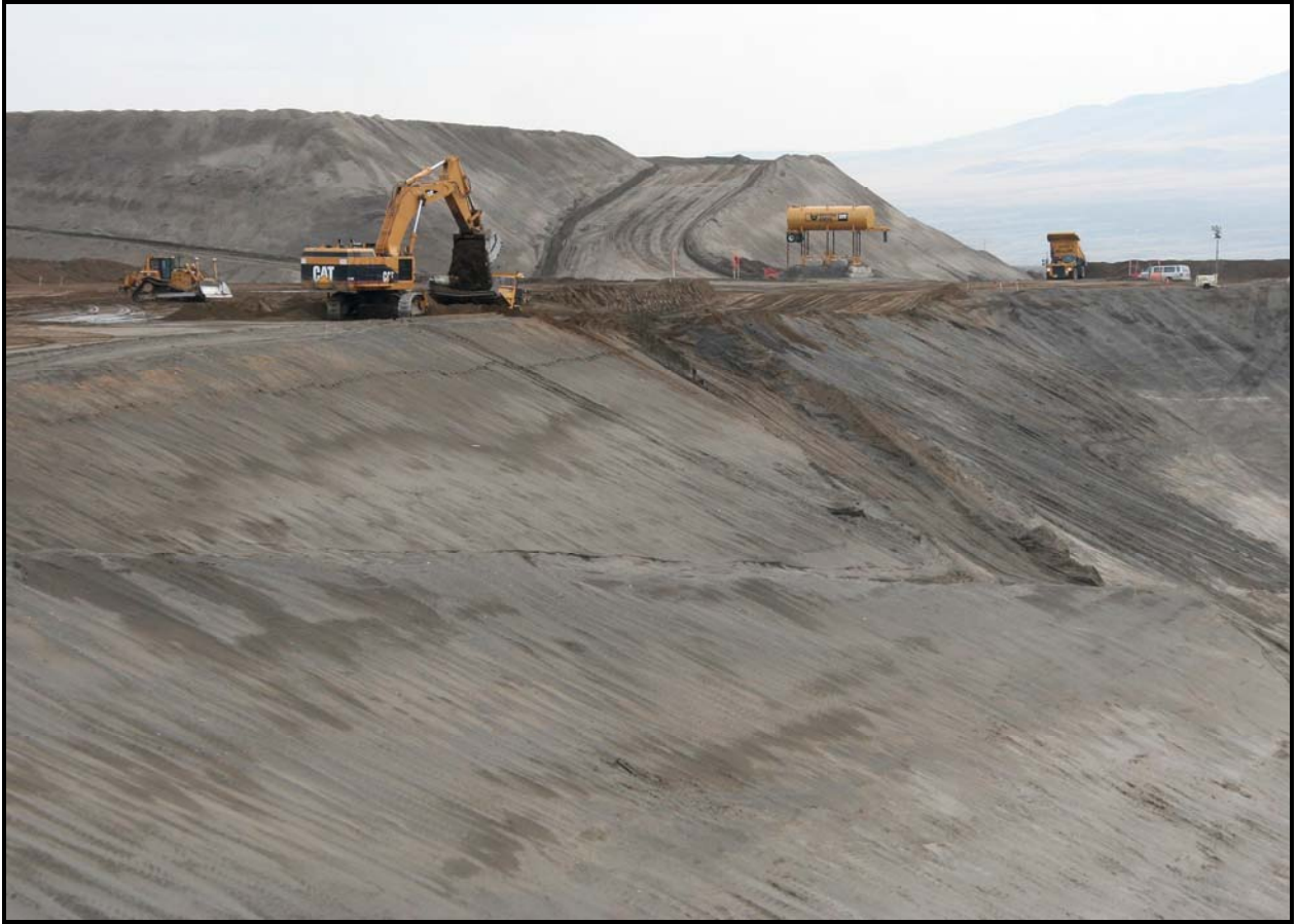
Excavation of super cell 10 is scheduled to be completed in August. This photo shows work next to the east sidewall of super cell 9.
