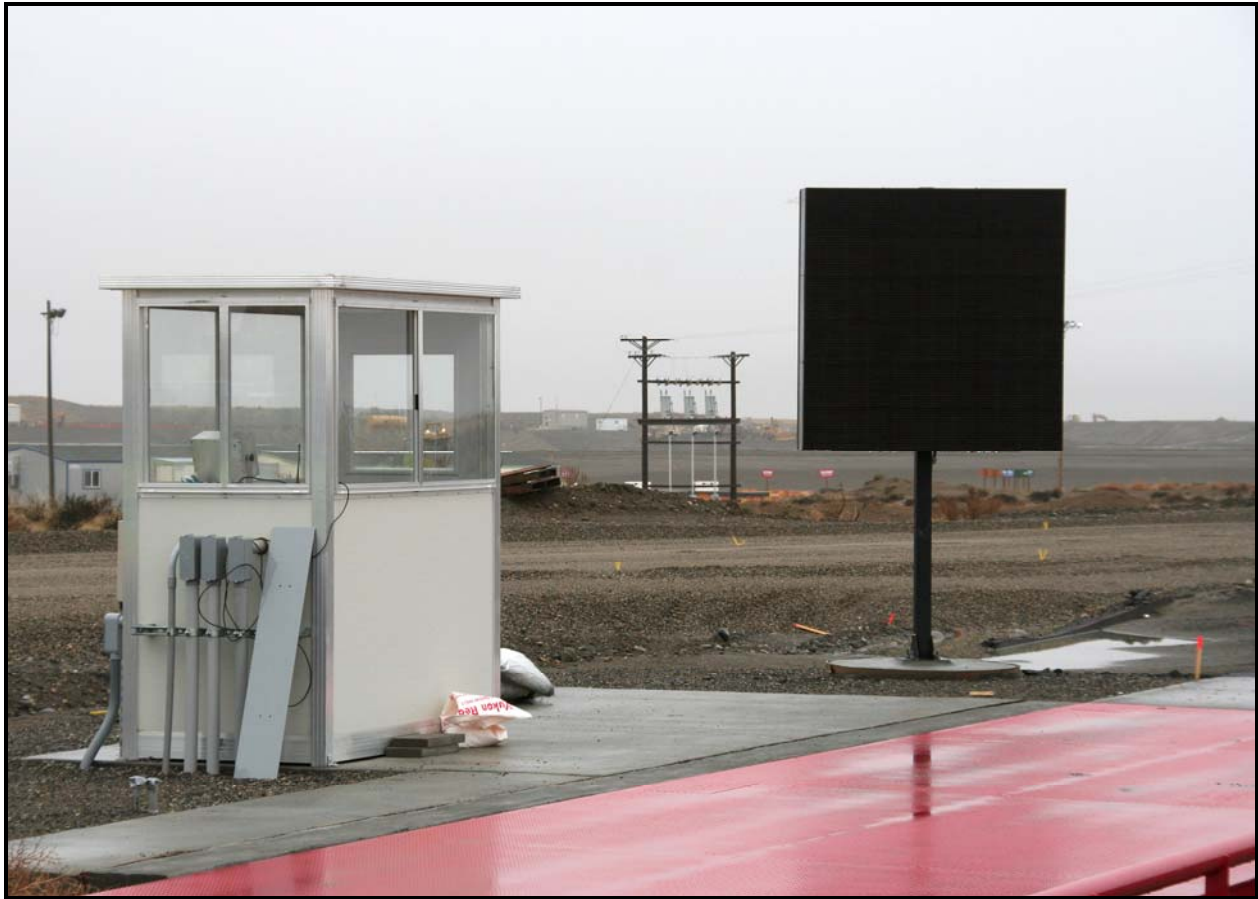
Fiber optic cable has been installed to allow internet access for the new third scale at the Environmental Restoration Disposal Facility.
