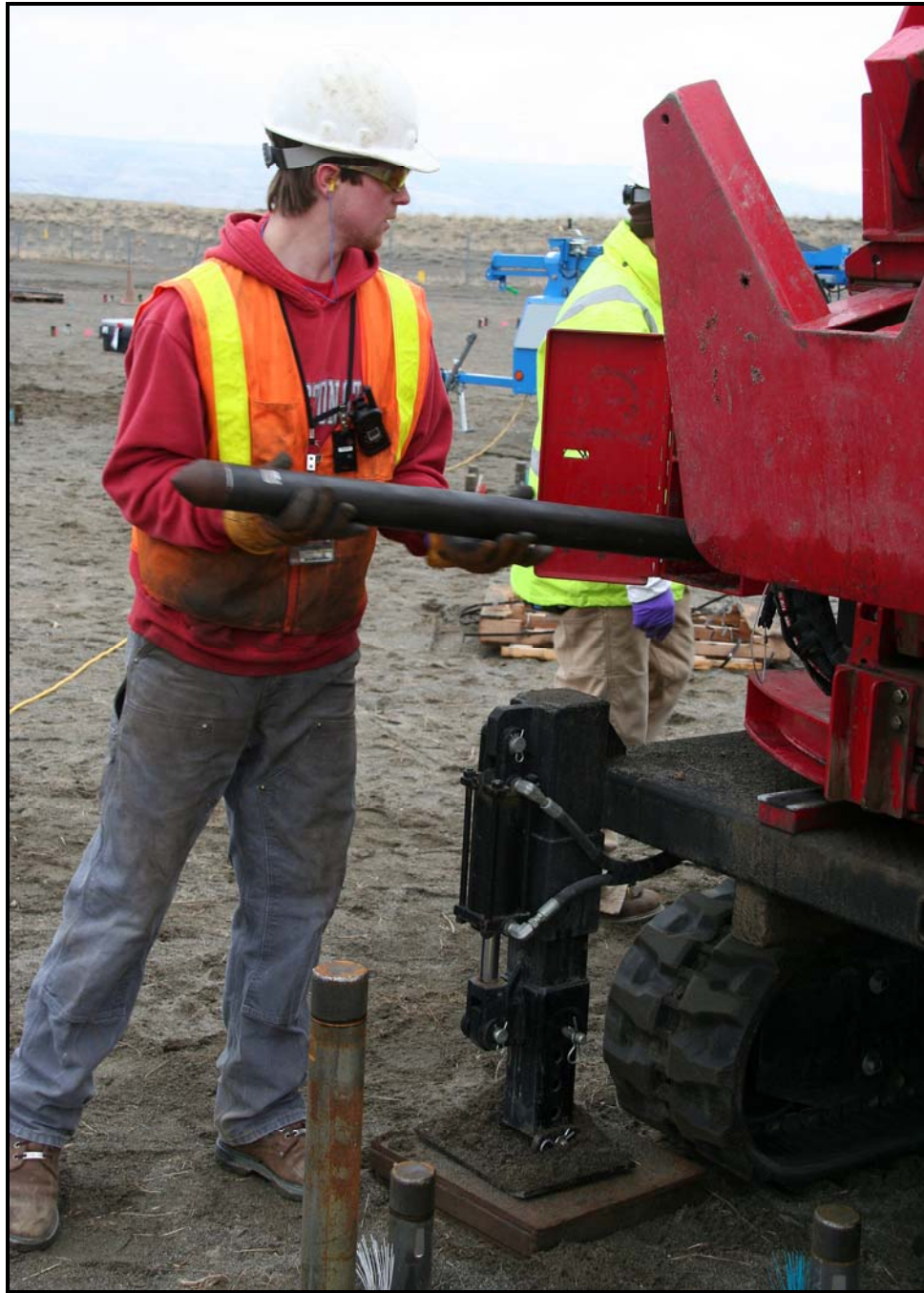
North Wind personnel continues to install cone penetrometers to a target depth of 22 feet at the 618-10 Burial Ground.
