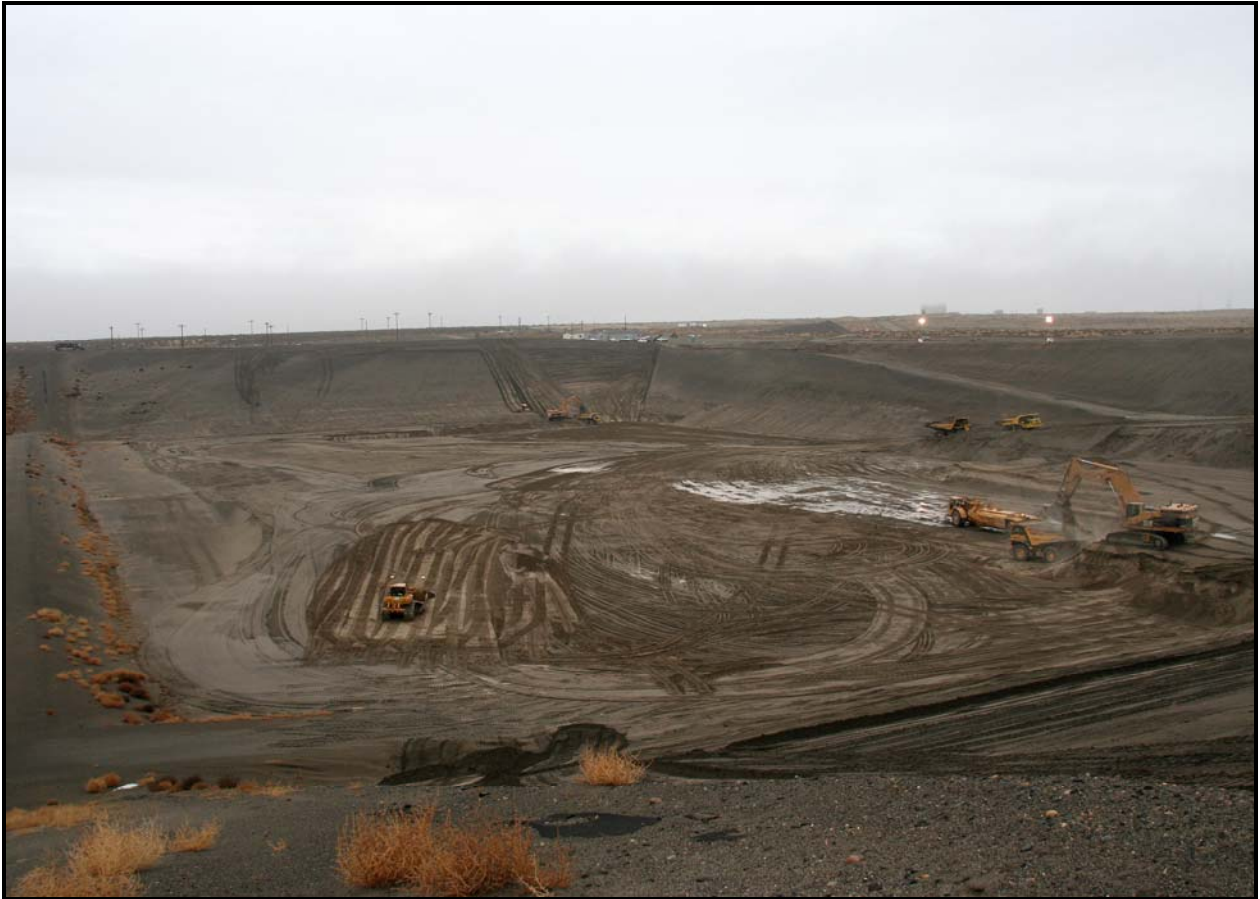
WCH subcontractor DelHur Industries continues excavation of super cell 9 at the Environmental Restoration Disposal Facility. Excavation is 95% complete.
