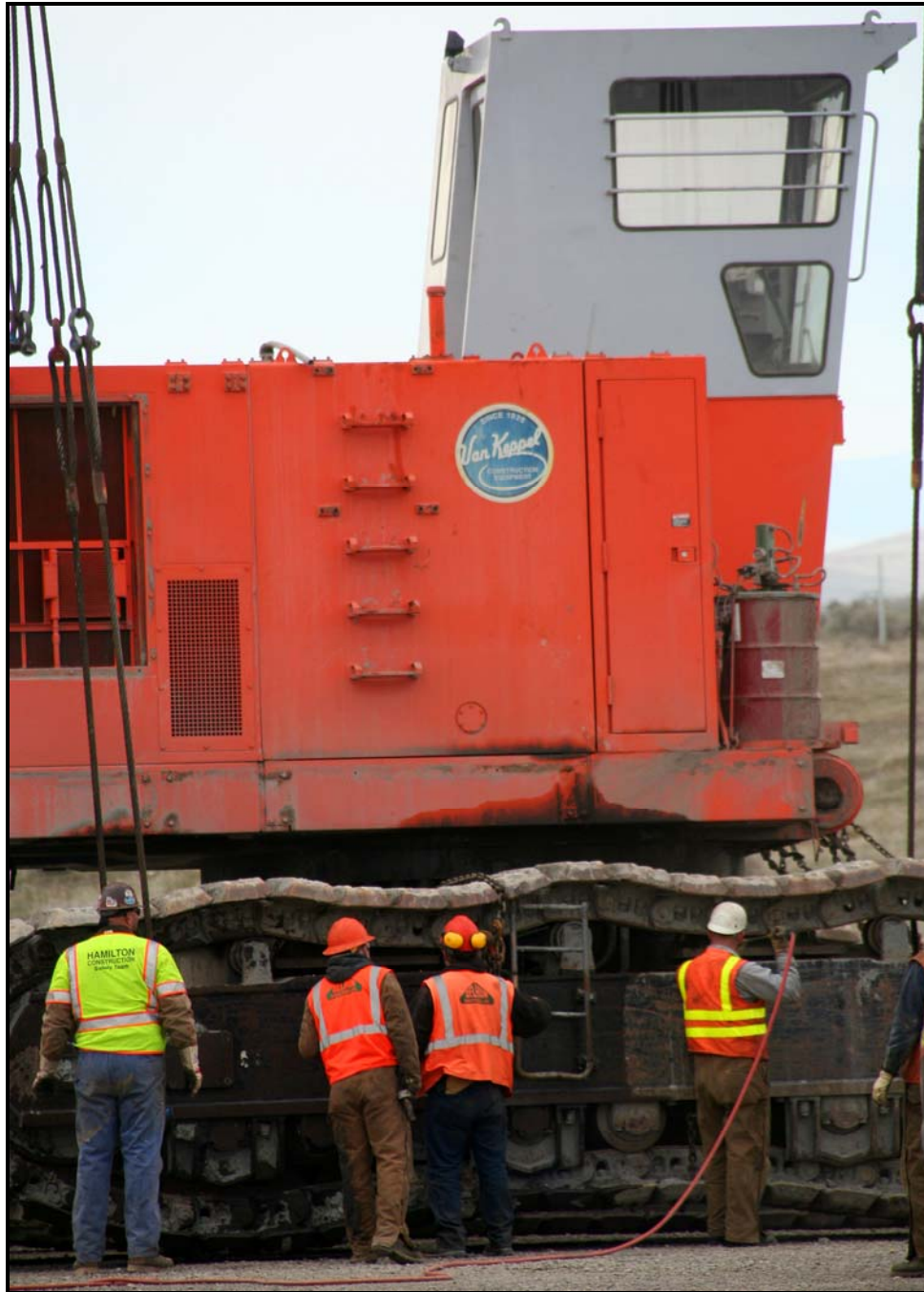
Work has begun on assembling the 13-yard bucket excavator at the Environmental Restoration Disposal Facility.
