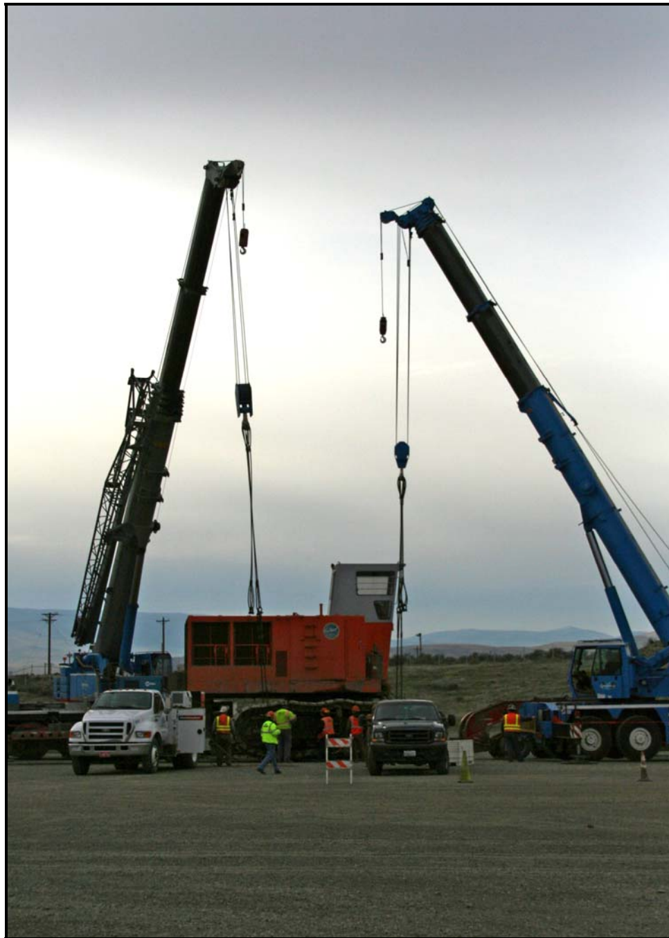
A 13-yard bucket excavator delivered to the Environmental Restoration Disposal Facility will be used to help dig super cell 10.
