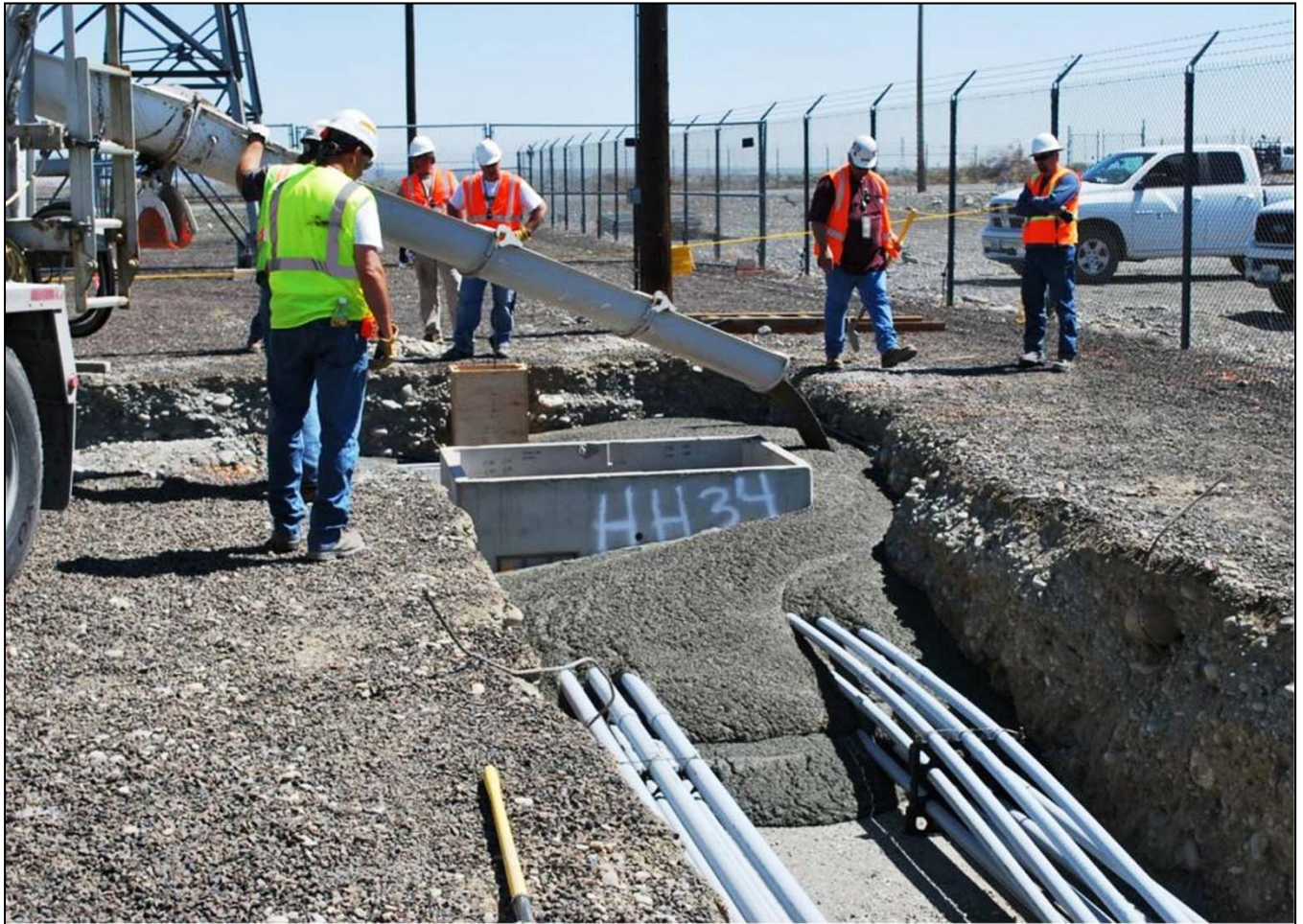
Controlled density fill is placed in conduit trenches on the east side of the A9 Switchyard Site. Last week, 270 cubic feet of the fill was placed in the trenches.
