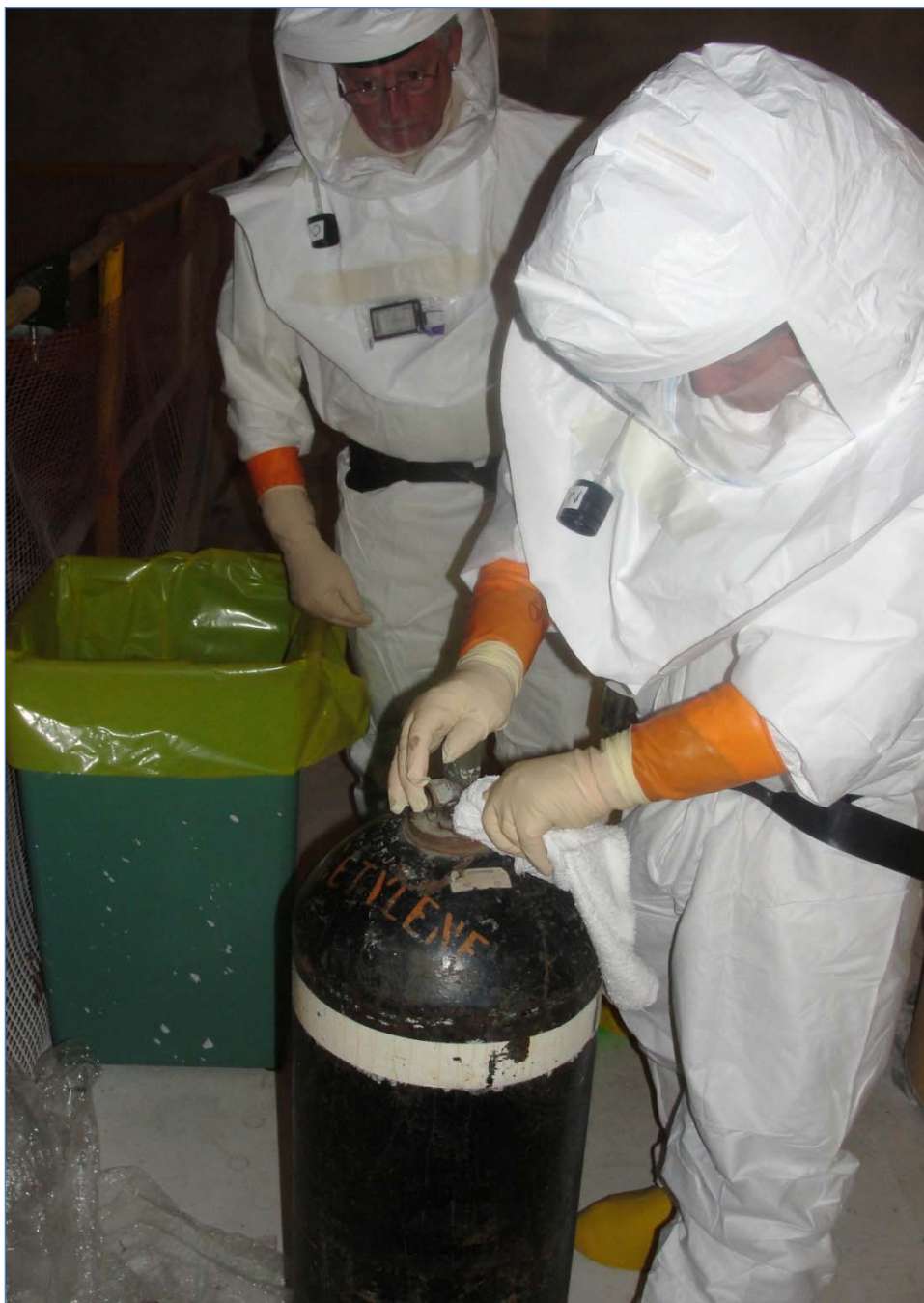
Workers decontaminate a compressed gas cylinder in preparation for removal from the U Canyon and disposal of the contents.
