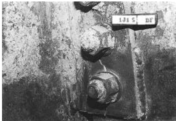
Figure 1-5 Vertical Fracture through Beam Shear Plate Connection
