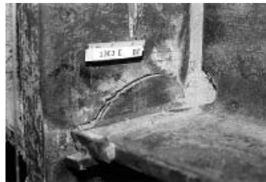
b. Column Flange "Divot" Fracture
