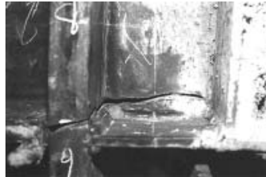
b. Fracture Progresses into Column Web
