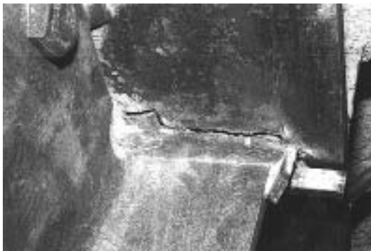
a. Fracture at Fused Zone
