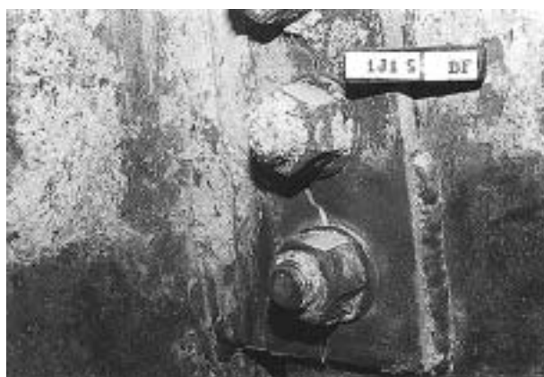
Figure 1-5 Vertical Fracture through Beam Shear Plate Connection
