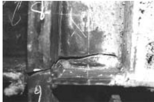
b. Fracture Progresses into Column Web
