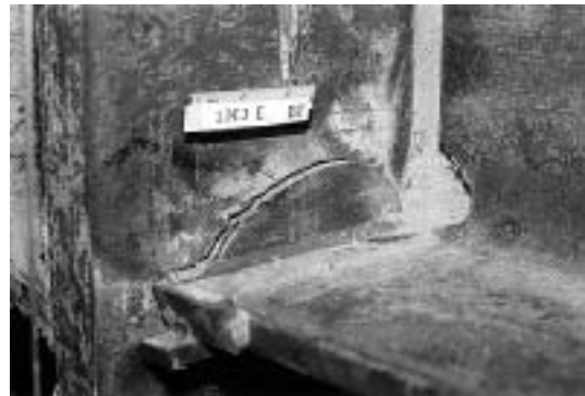
b. Column Flange "Divot" Fracture
