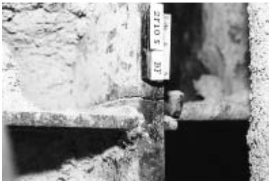
a. Fractures through Column Flange
