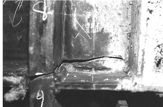
b. Fracture Progresses into Column Web
