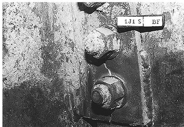
Figure 1-5 Vertical Fracture through Beam Shear Plate Connection
