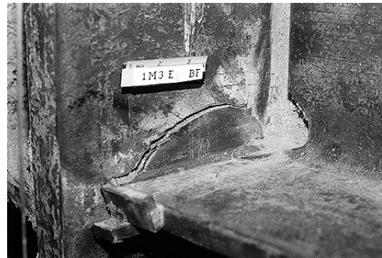
b. Column Flange "Divot" Fracture
