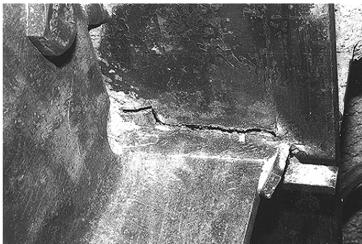
a. Fracture at Fused Zone
