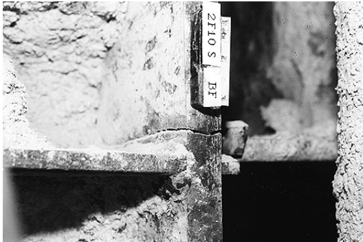
a. Fractures through Column Flange
