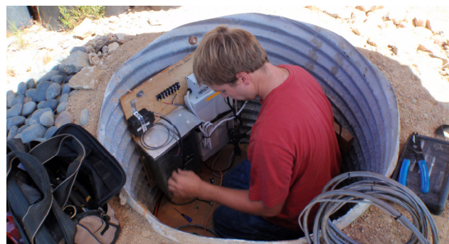
Field Instrumentation Specialist Jacob Crummey of Caltech installing new batteries as part of the final stages of upgrading the Dos Picos County Park seismic station in Rosemont, CA, with modern seismic equipment provided through economic stimulus funding. Credit: David Johnson, Caltech.
