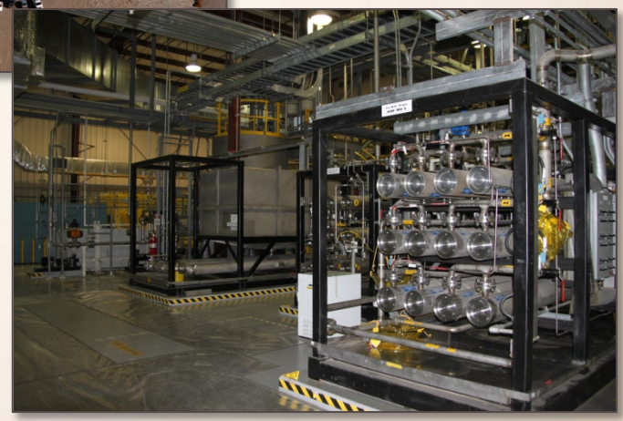
Effluent Treatment Facility
