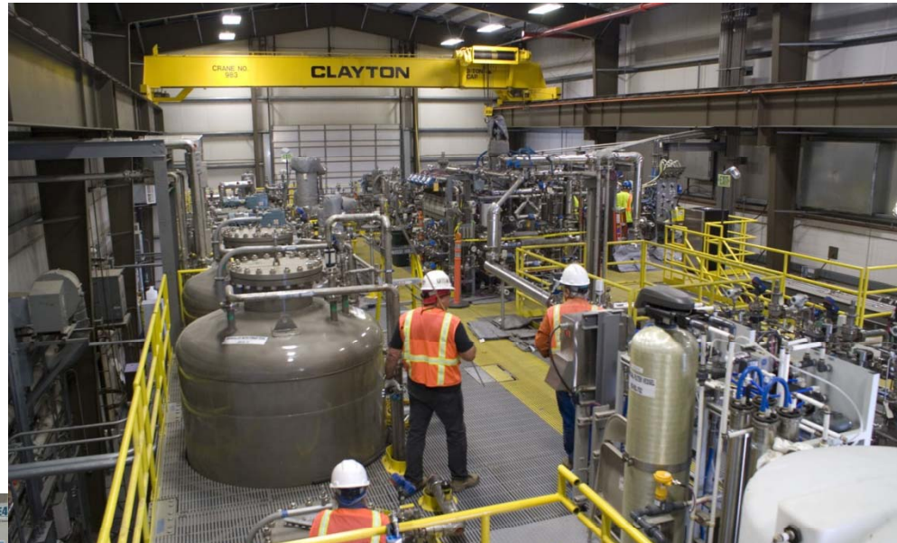
Employees work on the upper level of the Pretreatment Engineering Platform. The upper level contains the pulse jet mixers, samplers, instrumentation, and ventilation valving.
