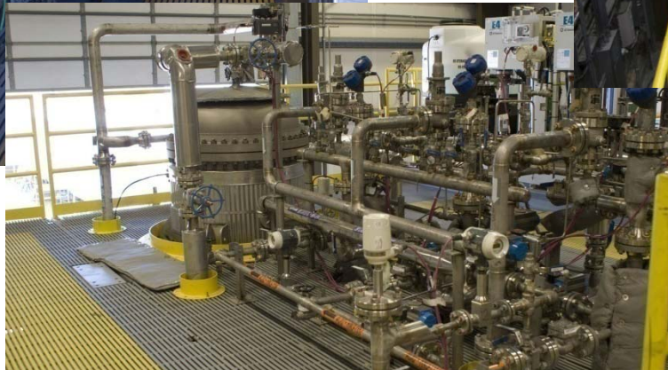
Pretreatment Engineering Platform ultrafilter pulse pots and valves provide the ability to back pulse the ultrafilters to maintain flow
