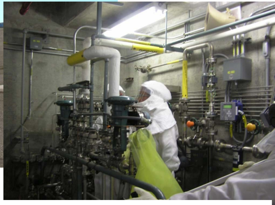
A team of workers is busy decontaminating the condenser room at the 242-A Evaporator. The work follows a major upgrade to the facility.
