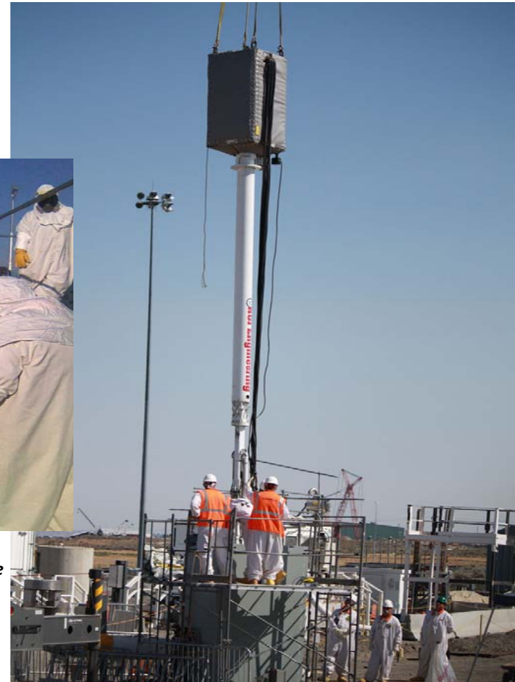
Crews installed a modified slucier with extended reach capabilities into Tank C-112
