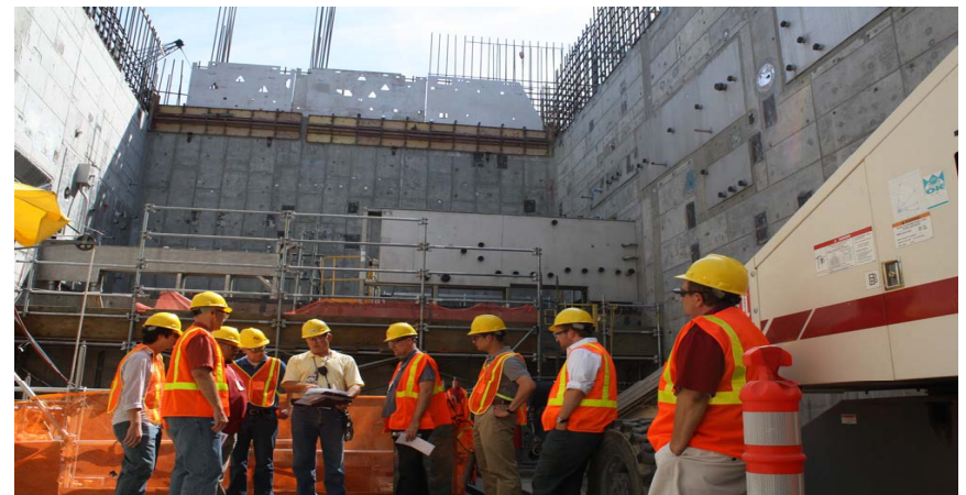
Acting Secretary Huizenga visits the Waste Treatment Plant
